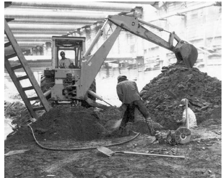
Figure 10.3 Braced cut in the construction of Washington, DC Metro, May 1974 (Courtesy of Ralph B. Peck)
