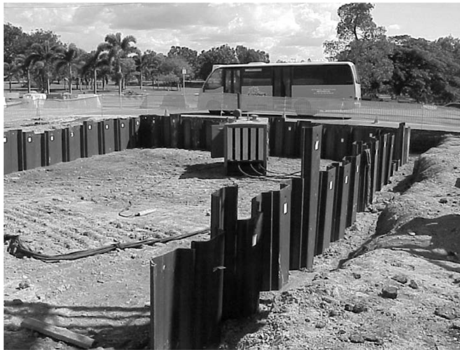
Figure 9.4 A steel sheet pile wall (Courtesy of N. Sivakugan, James Cook University, Australia )
