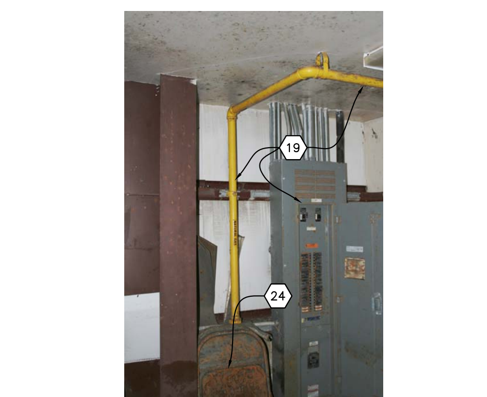
116 OMS 12 - COMM. / TELE. 105 INTERIOR PHOTOGRAPH
