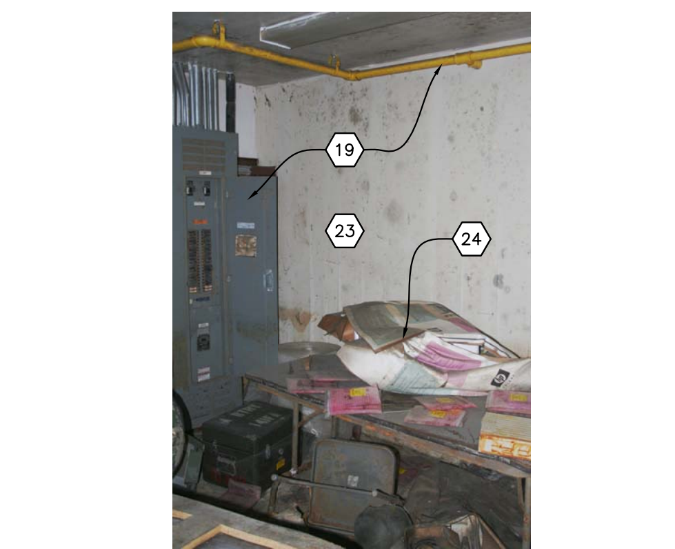
112 OMS 12 - COMM. / TELE. 105 INTERIOR PHOTOGRAPH
