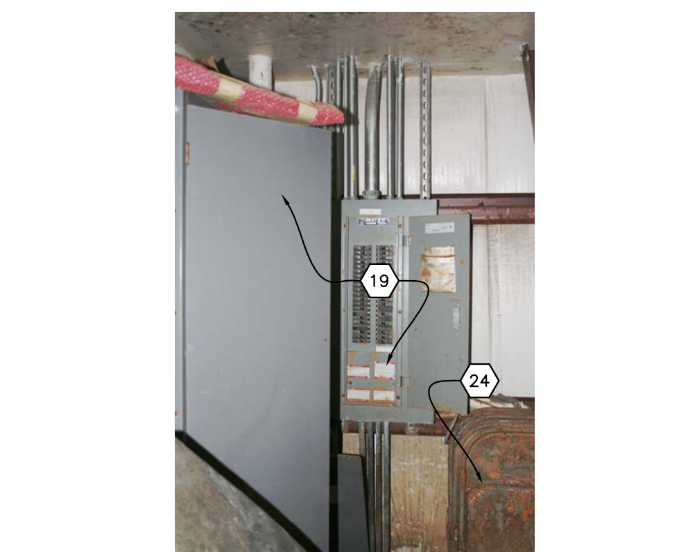
114 OMS 12 - COMM. / TELE. 105 INTERIOR PHOTOGRAPH
