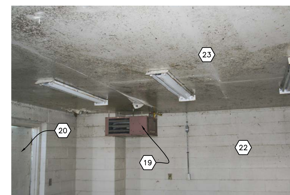
148 OMS 12 - POL EQ. STORAGE 120 INTERIOR PHOTOGRAPH
