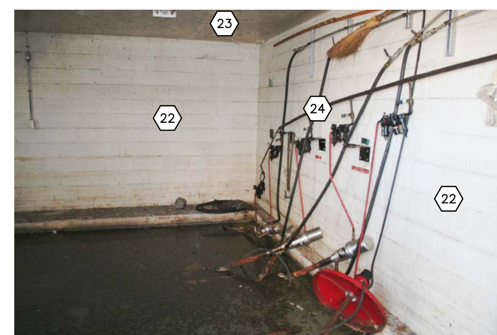
146 OMS 12 - POL EQ. STORAGE 120 INTERIOR PHOTOGRAPH
