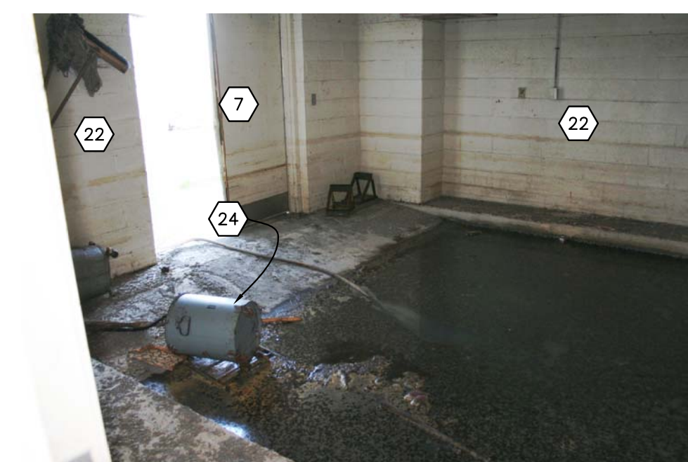
147 OMS 12 - POL EQ. STORAGE 120 INTERIOR PHOTOGRAPH
