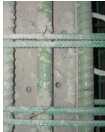
Fig. 4.5: Image of drilled holes that need to be cleaned. The job conditions will vary on different projects. Here the installer has to work around reinforcement (Courtesy of Wiss, Janney, Elstner Associates, Inc.)
