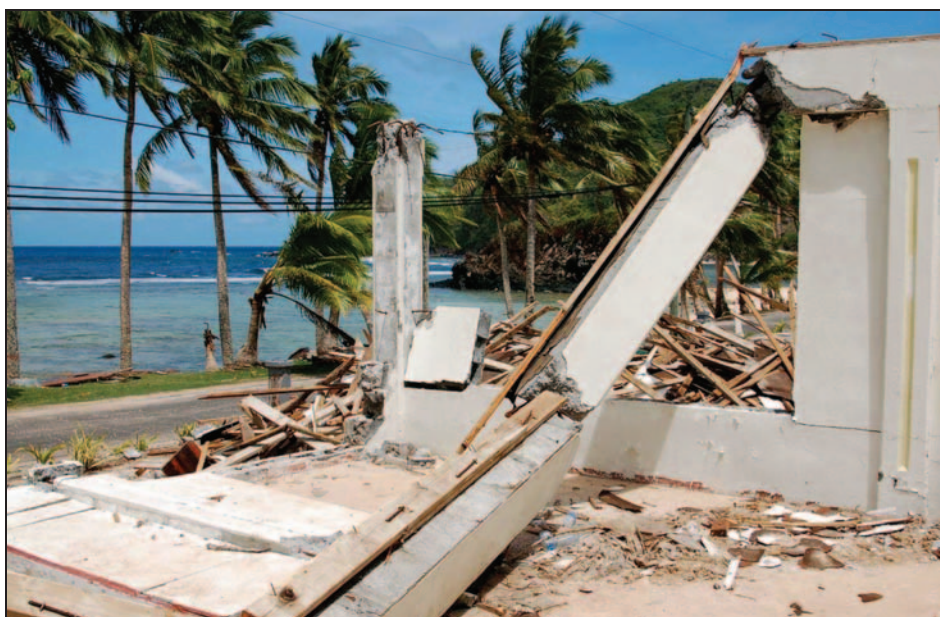
Figure 3-12. Damage from the 2009 tsunami (Amanave, American Samoa)
