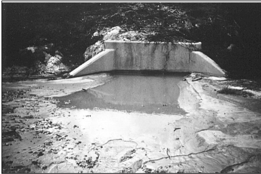
Figure VI-15--Sediment Deposition in Culvert
