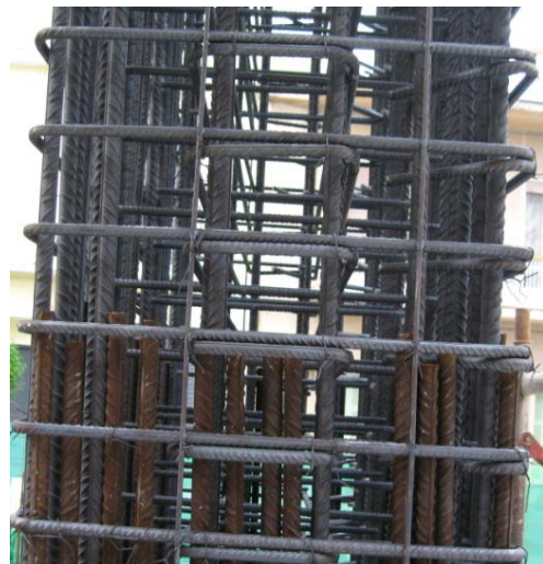
Fig. 1 Poor practice of ties in vertical columns
