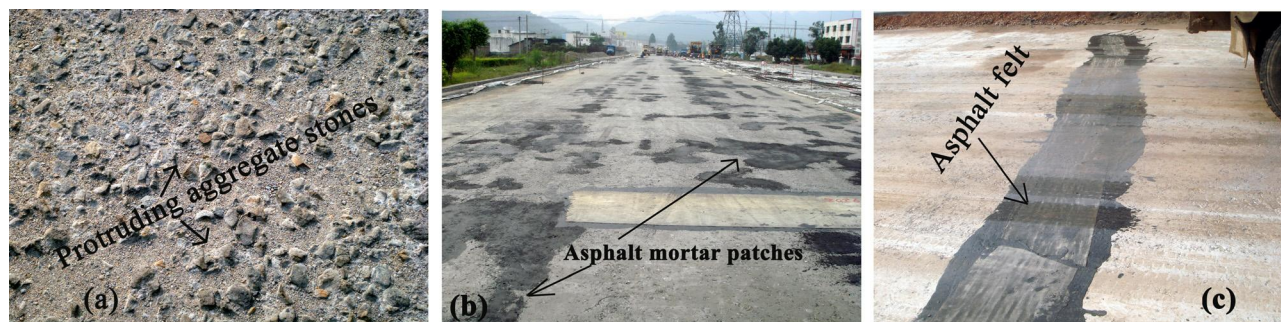
FIG. 2 (a) Aggregate particles protruding on the base surface; (b) local defects patched with asphalt mortar before construction of EWCA interlayer; and (c) cracked base surface fixed with asphalt felt before construction of EWCA interlayer.
