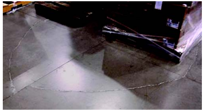
Fig. 2.2.2—Diagonal cracking due to curling of floor slab.
