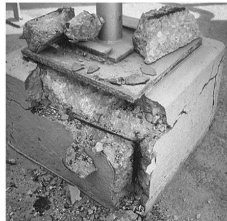
Fig. 2.2.4—Deformation and spalling due to corrosion of reinforcement.
