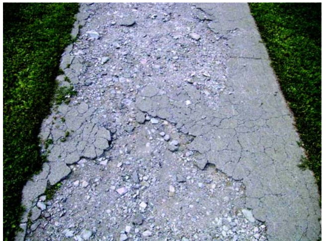
Fig. 2.2.19.4—Very severe scaling.
