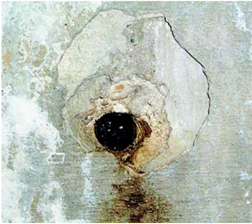
Fig. 2.2.20.1—Small spall due to tie rod rusting.
