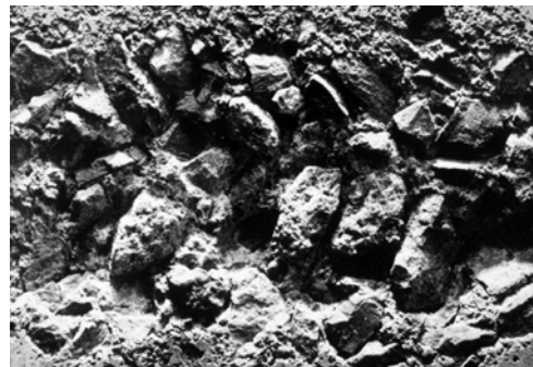
Fig. 2.2.6(f)—Disintegration due to erosion and cavitation damage.
