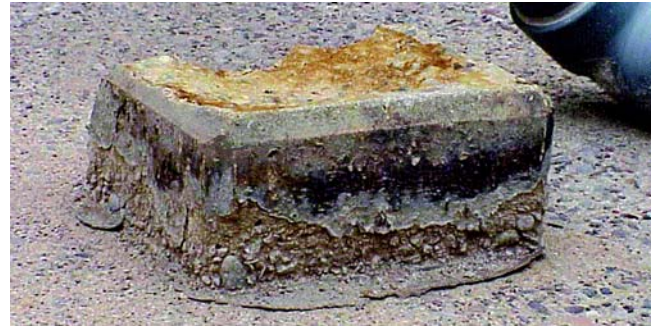
Fig. 2.2.6(c)—Disintegration from chemical attack.
