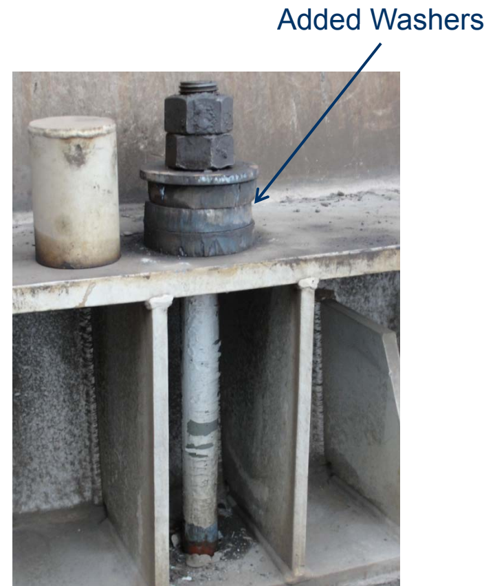
Stretched Bolt on Stack February 27, 2010 Chile Earthquake
