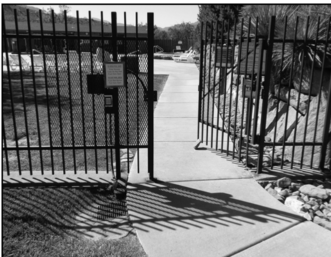
FIGURE 305.3 VIOLATION—WRONG SWING DIRECTION ON PEDESTRIAN ACCESS GATE
