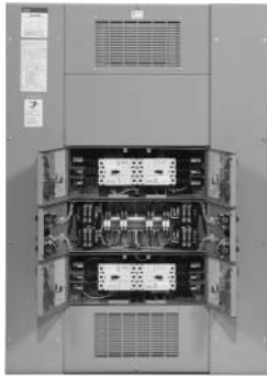
Elevator Control Panelboard
