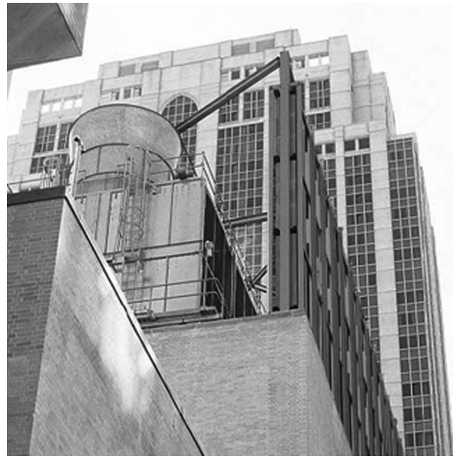
Fig. 1 Cooling Tower Noise Barrier (Courtesy Neil Moiseev)
