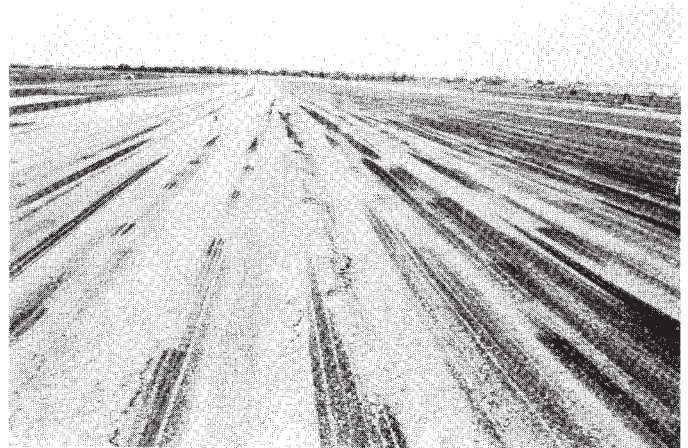
FIG. X1.38 Low-Severity Longitudinal Cracks, Approaching Medium
