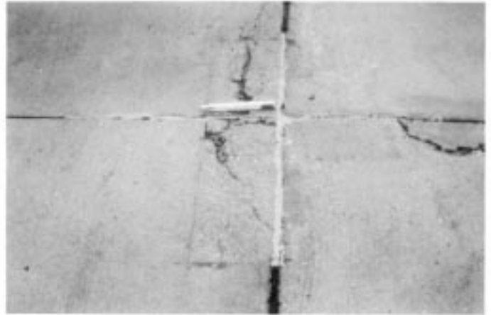
FIG. X2.32 High-Severity Small Patch
