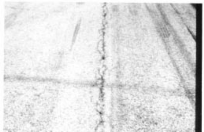
FIG. X1.39 Medium-Severity Longitudinal Construction Joint Crack
