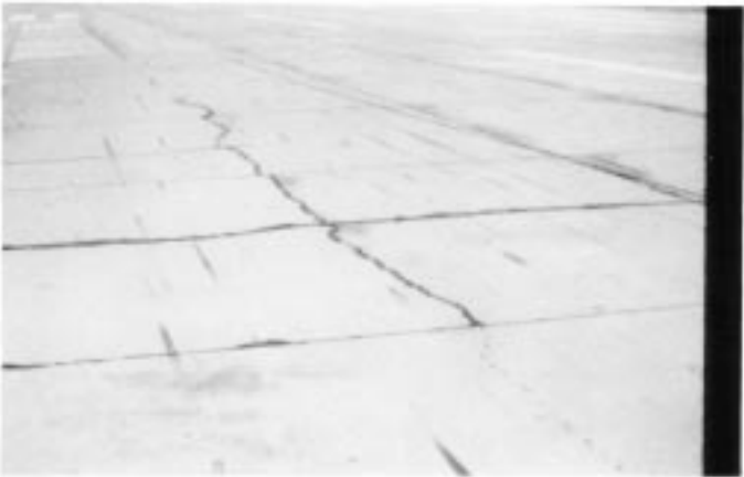
FIG. X2.54 Low-Severity Intersecting Cracks
