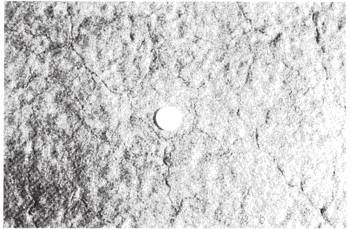
FIG. X1.15 Low-Severity Block Cracking, Small Blocks Defined by Hairline Cracks
