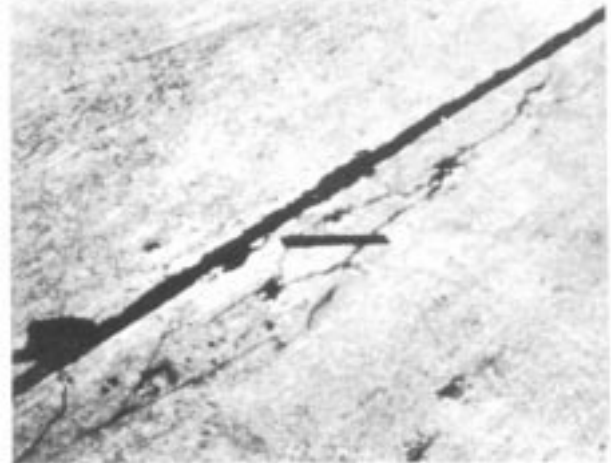
FIG. X2.20 Medium-Severity "D" Cracking
