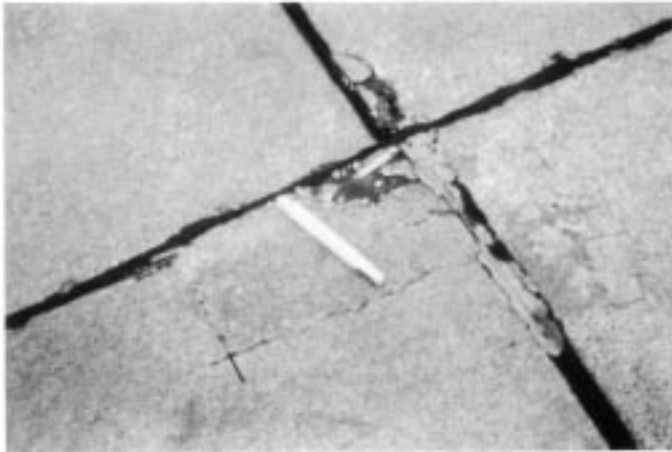
FIG. X2.30 Medium-Severity Small Patch
