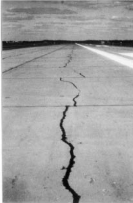
FIG. X2.12 Medium-Severity Longitudinal Crack
