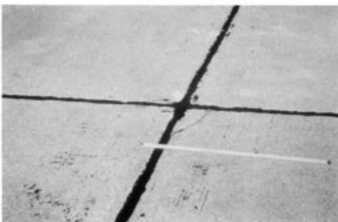
FIG. X2.69 Low-Severity Corner Spall
