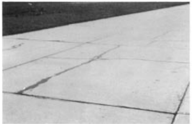
FIG. X2.57 Medium-Severity Intersecting Cracks
