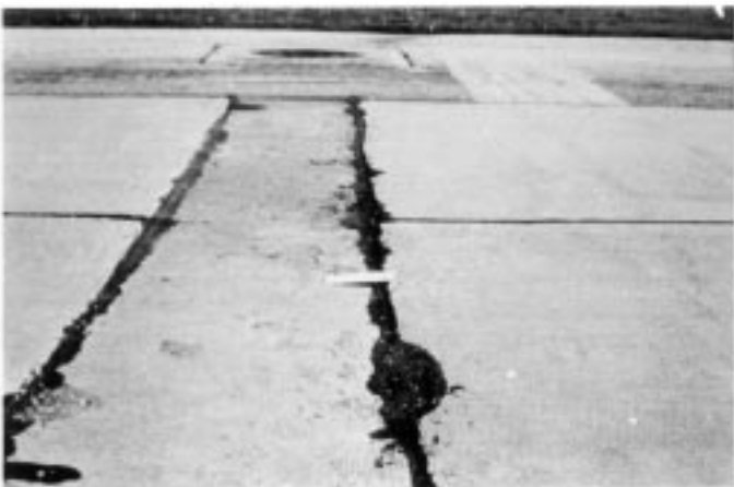
FIG. X2.36 Medium-Severity Utility Cut
