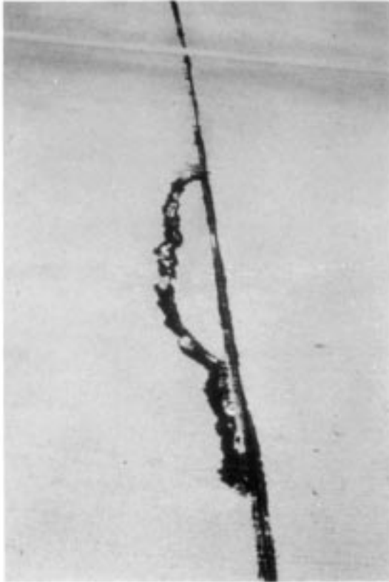
FIG. X2.63 Low-Severity Joint Spall
