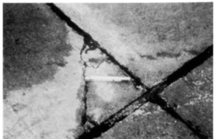
FIG. X2.71 Medium-Severity Corner Spall
