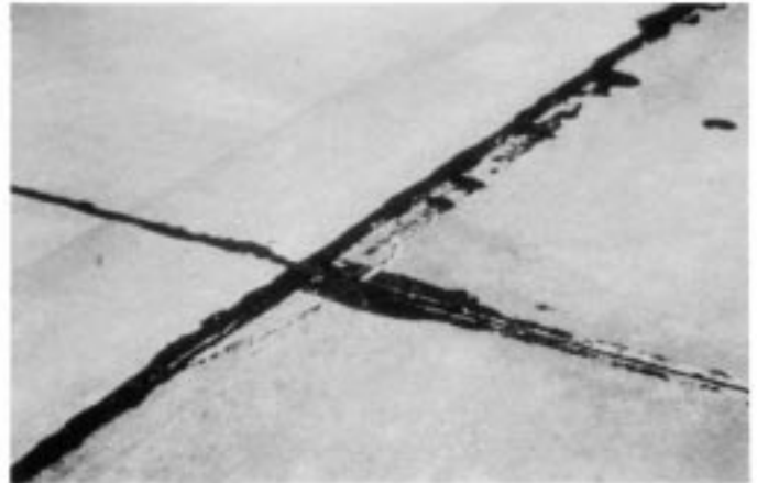
FIG. X2.70 Low-Severity Corner Spall
