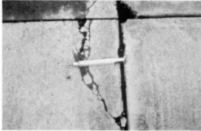
FIG. X2.72 Medium-Severity Corner Spall
