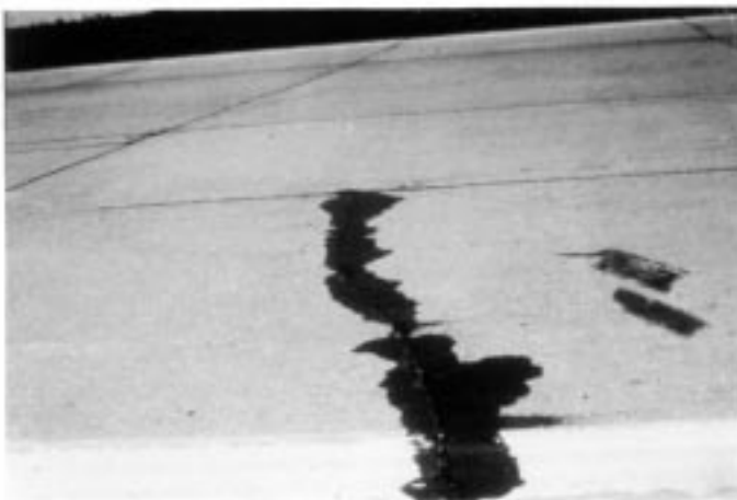
FIG. X2.13 Medium-Severity Transverse Crack
