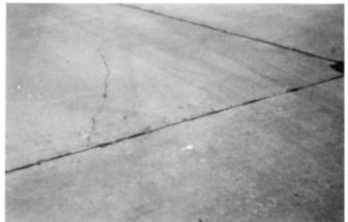
FIG. X2.11 Low-Severity Diagonal Crack
