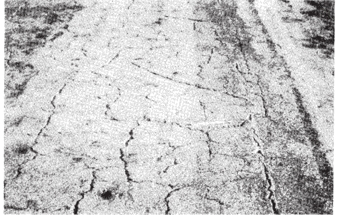
FIG. X1.20 High-Severity Block Cracking
