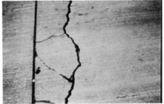
FIG. X2.65 Medium-Severity Joint Spall
