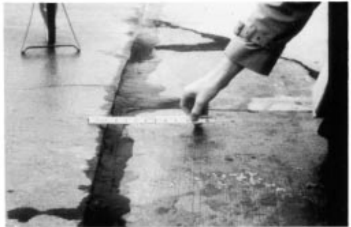
FIG. X2.51 Medium-Severity Settlement on Apron (>1/2 in. (13 mm))
