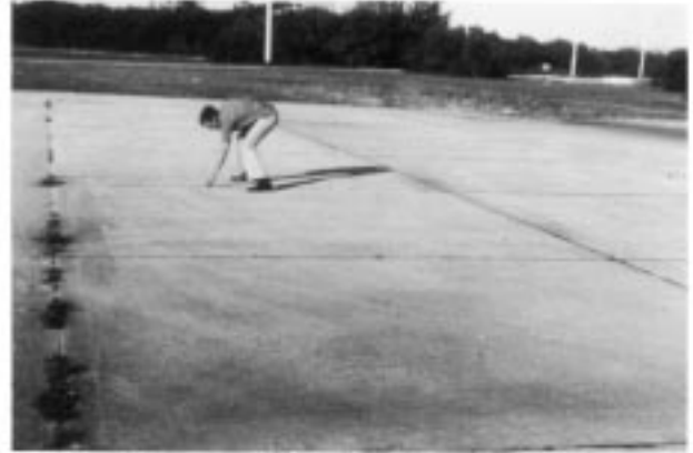
FIG. X2.27 High-Severity Joint Seal Damage (Extensive Amount of Weed Growth)
