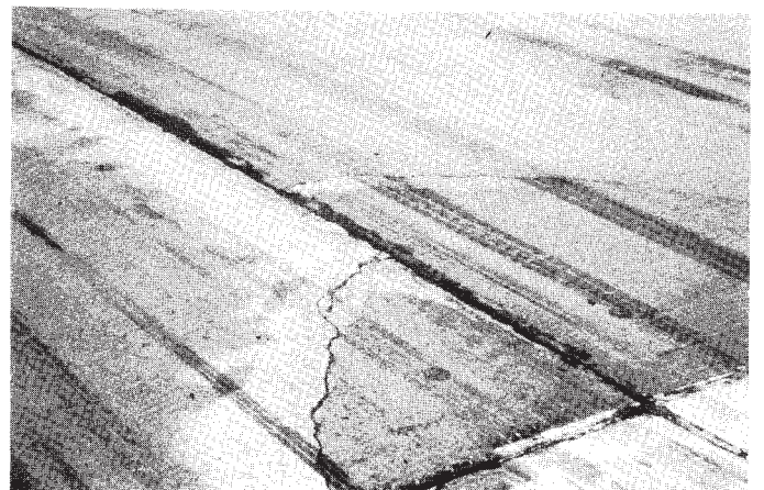
FIG. X2.7 Medium-Severity Corner Break
