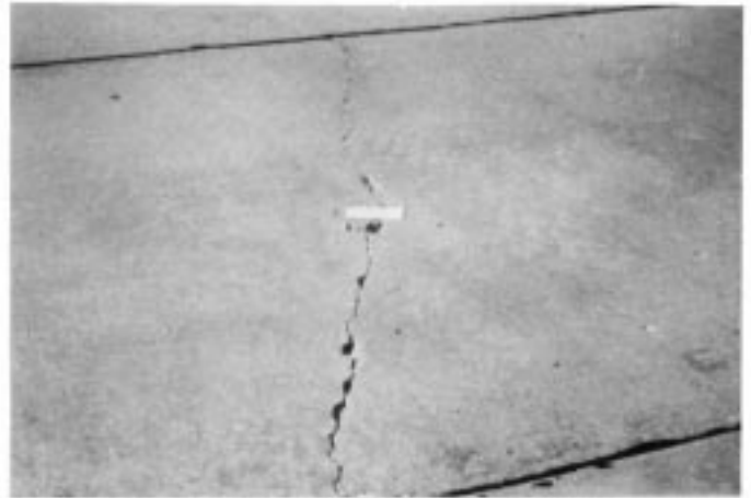
FIG. X2.14 Medium-Severity Transverse Crack
