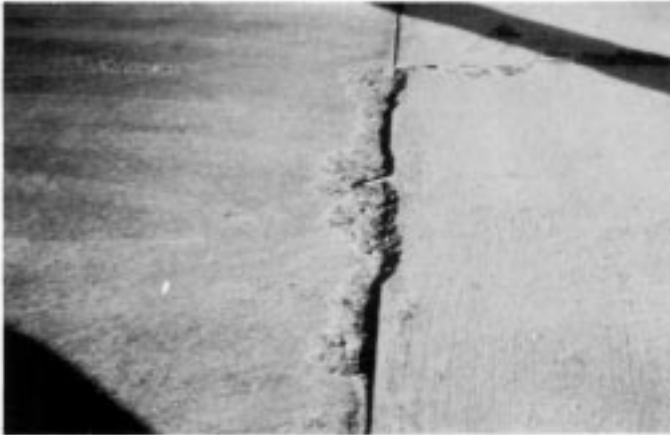
FIG. X2.68 High-Severity Joint Spall
