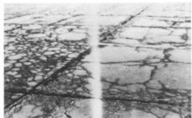
FIG. X2.48 High-Severity Scaling Caused by Alkali Aggregate Reaction
