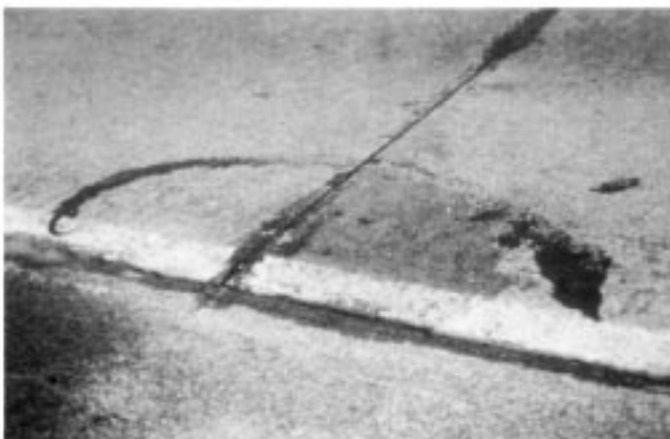
FIG. X2.39 Pumping (Note Fine Material on Surface That has Been Pumped Out Causing Corner Break)
