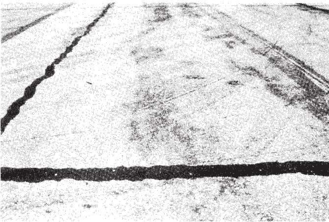
FIG. X1.31 Low-Severity Joint Reflection Cracking, Filled Crack
