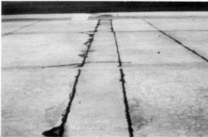
FIG. X2.35 Low-Severity Utility Cut
