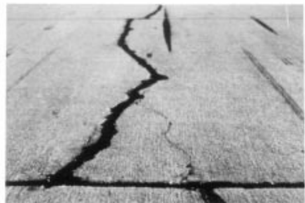
FIG. X2.16 High-Severity Longitudinal Cracks
