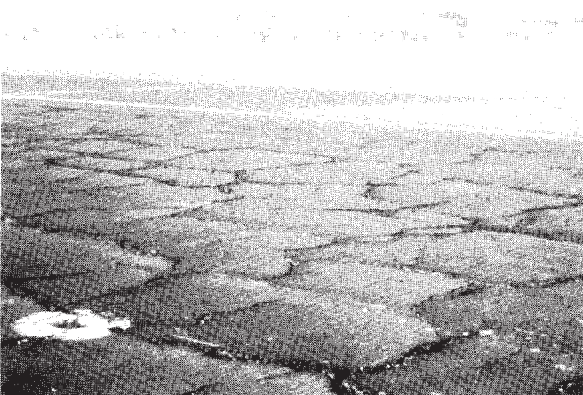
FIG. X1.19 High-Severity Block Cracking
