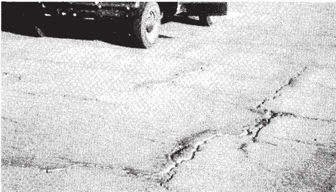
FIG. X1.18 High-Severity Block Cracking
