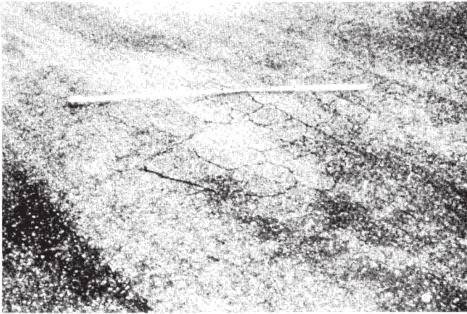
FIG. X1.7 Medium-Severity Alligator Cracking, Approaching High Severity (Example 1)
