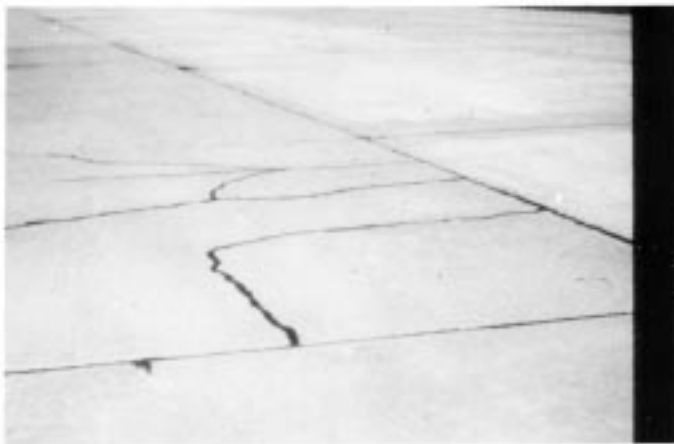
FIG. X2.55 Low-Severity Intersecting Cracks
