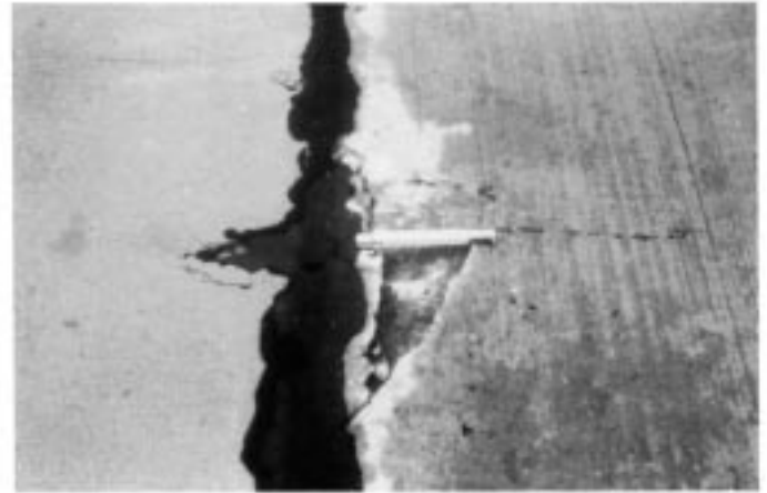
FIG. X2.66 Medium-Severity Joint Spall
