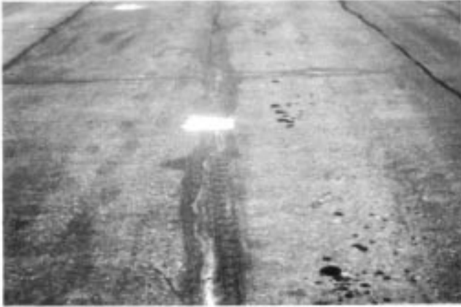
FIG. X1.40 Medium-Severity Longitudinal Crack (Note the Crack is Reflective But Not at the Joint of Slab)
