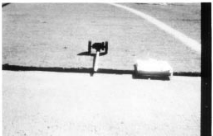
FIG. X2.52 High-Severity Settlement on Taxiway/Runway (3/4 in. (18 mm))
