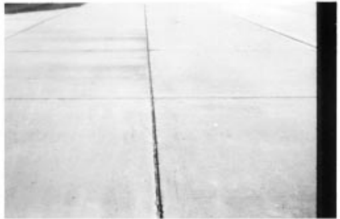
FIG. X2.40 Pumping (Note Stains on Pavement)
