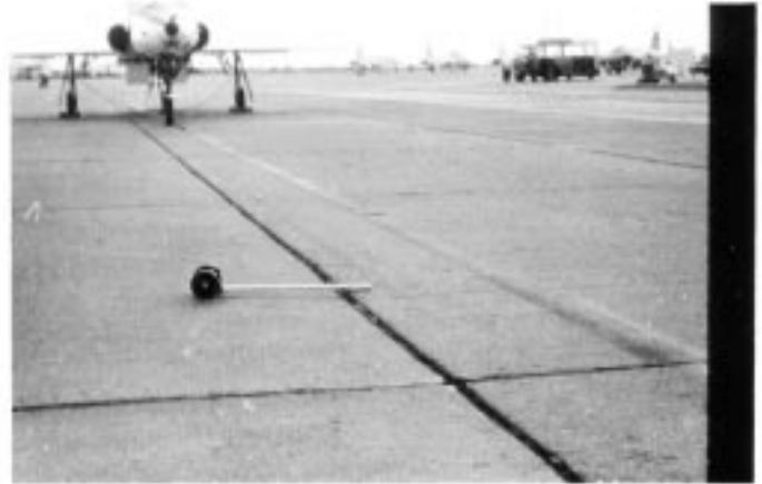
FIG. X2.50 Low-Severity Settlement on Apron
