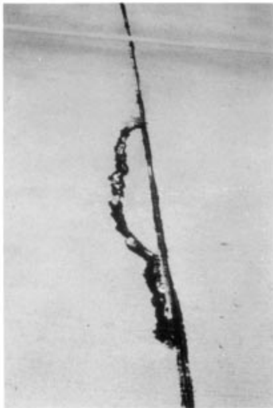
FIG. X2.63 Low-Severity Joint Spall
