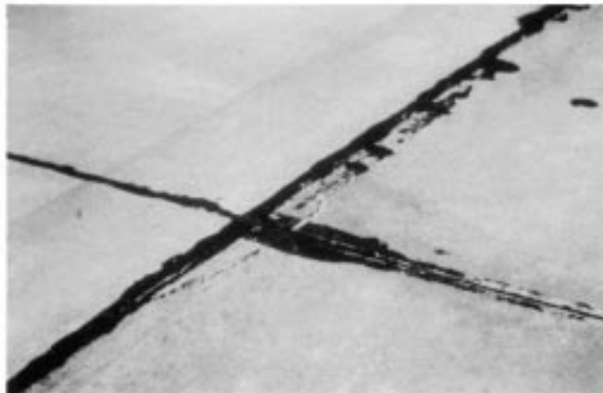
FIG. X2.70 Low-Severity Corner Spall
