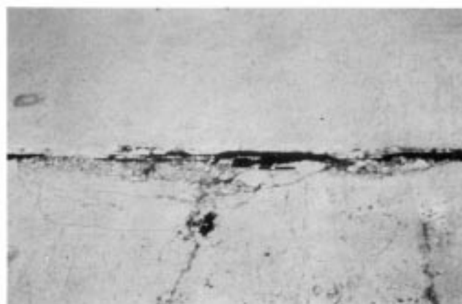
FIG. X2.67 High-Severity Joint Spall
