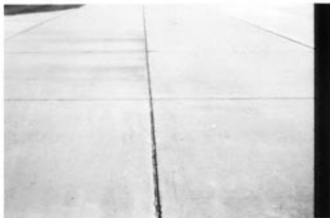
FIG. X2.40 Pumping (Note Stains on Pavement)
