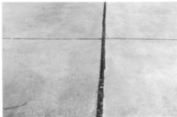
FIG. X2.26 High-Severity Joint Seal Damage (Complete Loss of Sealant; Joint is Filled with Incompressible Material)
