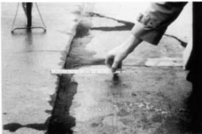
FIG. X2.51 Medium-Severity Settlement on Apron (>1/2 in. (13 mm))
