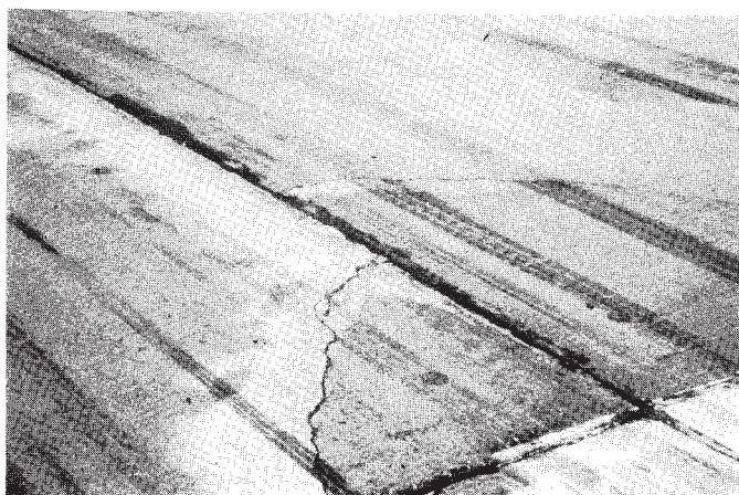
FIG. X2.7 Medium-Severity Corner Break
