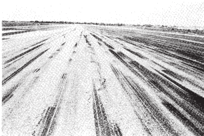
FIG. X1.38 Low-Severity Longitudinal Cracks, Approaching Medium
