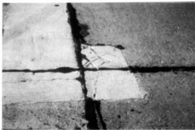
FIG. X2.31 Medium-Severity Small Patch
