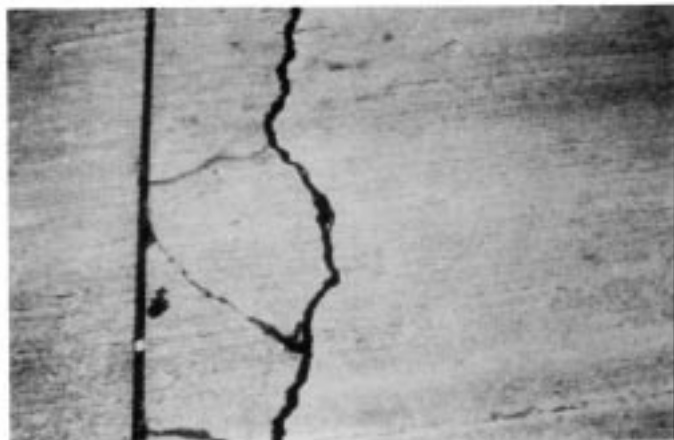
FIG. X2.65 Medium-Severity Joint Spall
