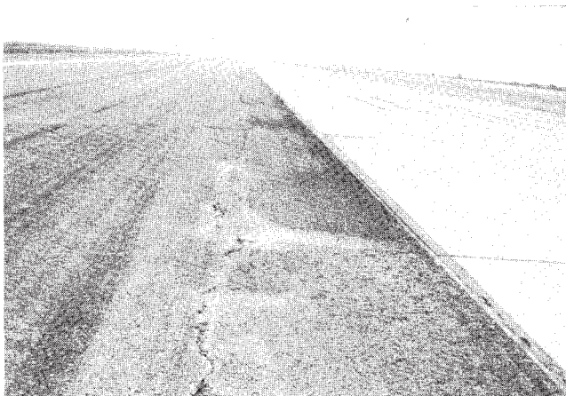
FIG. X1.41 Medium-Severity Longitudinal Crack
