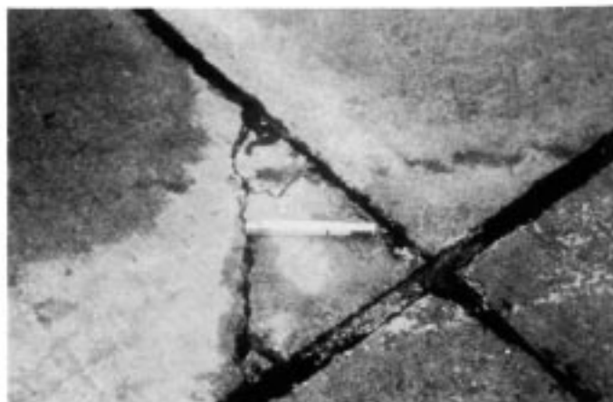
FIG. X2.71 Medium-Severity Corner Spall
