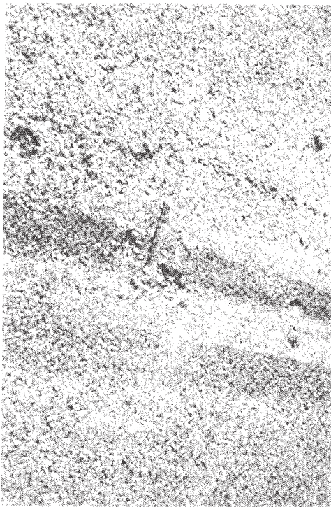
FIG. X1.65 High-Severity Raveling/Weathering on a Porous Friction Course Surface
