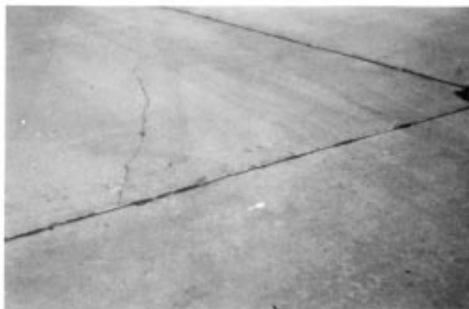
FIG. X2.11 Low-Severity Diagonal Crack
