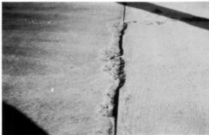
FIG. X2.68 High-Severity Joint Spall
