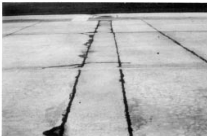
FIG. X2.35 Low-Severity Utility Cut
