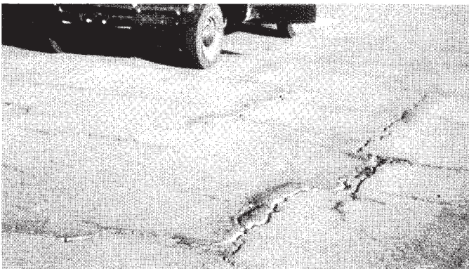
FIG. X1.18 High-Severity Block Cracking
