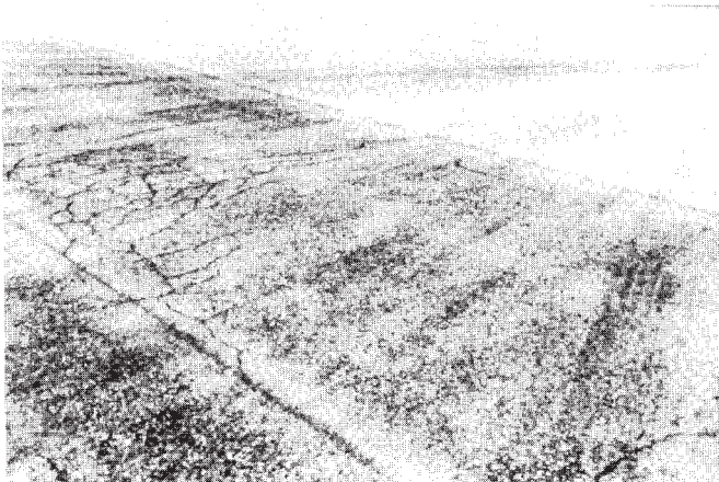
FIG. X1.8 Medium-Severity Alligator Cracking, Approaching High Severity (Example 2)
