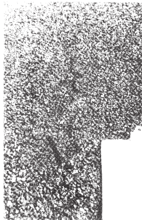
FIG. X1.44 Medium-Severity Crack in Porous Friction Course
