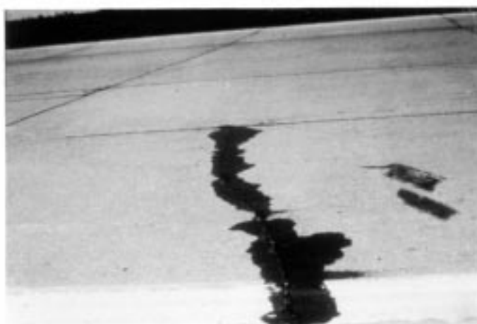
FIG. X2.13 Medium-Severity Transverse Crack
