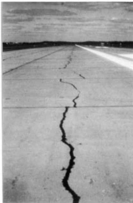
FIG. X2.12 Medium-Severity Longitudinal Crack
