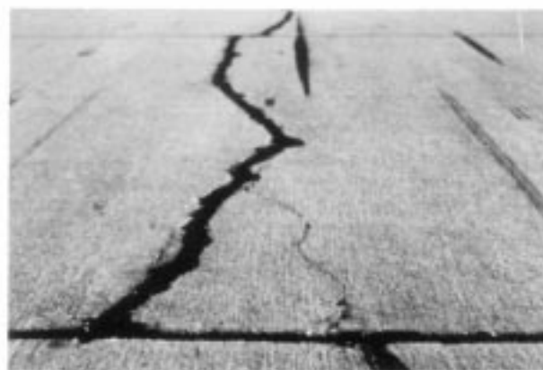
FIG. X2.16 High-Severity Longitudinal Cracks
