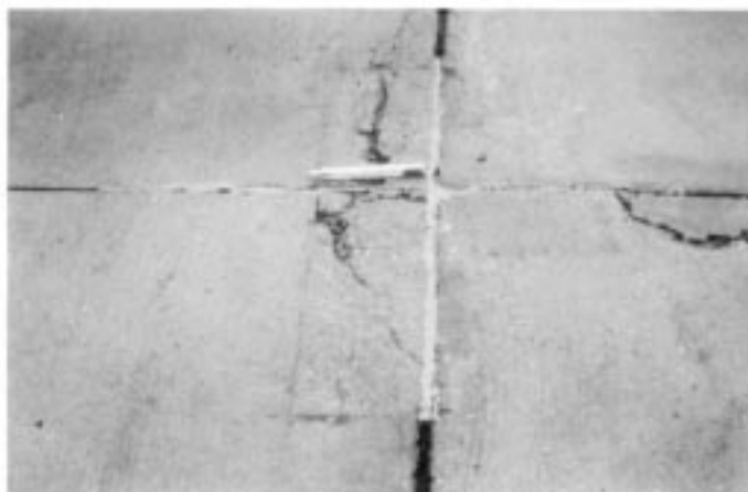
FIG. X2.32 High-Severity Small Patch
