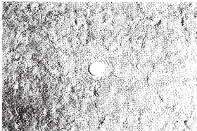
FIG. X1.15 Low-Severity Block Cracking, Small Blocks Defined by Hairline Cracks
