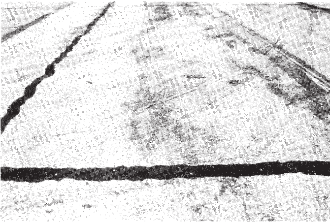
FIG. X1.31 Low-Severity Joint Reflection Cracking, Filled Crack
