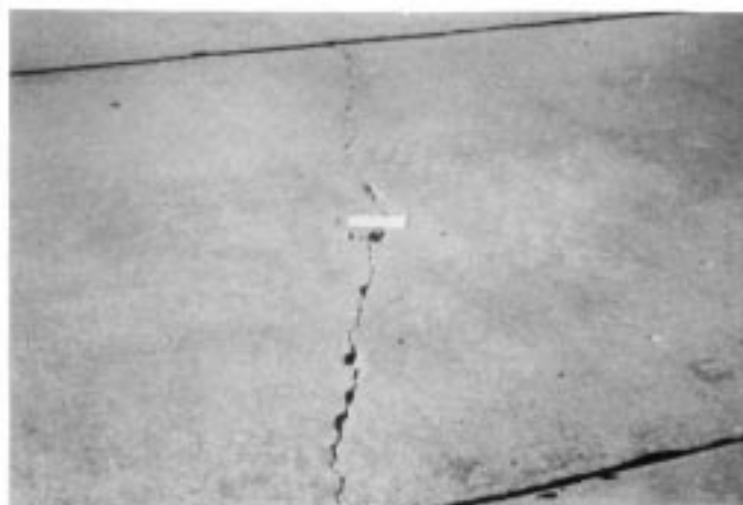
FIG. X2.14 Medium-Severity Transverse Crack
