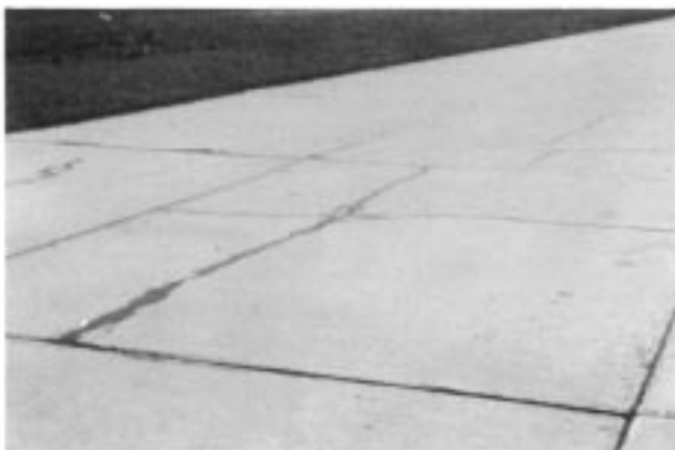
FIG. X2.57 Medium-Severity Intersecting Cracks
