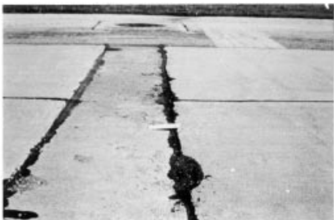
FIG. X2.36 Medium-Severity Utility Cut
