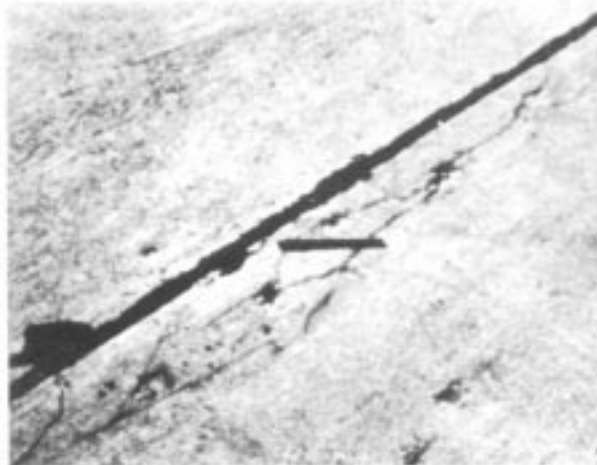
FIG. X2.20 Medium-Severity "D" Cracking
