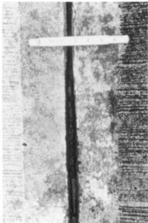
FIG. X2.25 Medium-Severity Joint Seal Damage (Note that Sealant has Lost Bond and is Highly Oxidized)
