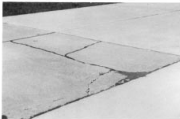
FIG. X2.56 Medium-Severity Intersecting Cracks
