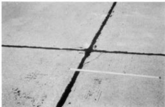
FIG. X2.69 Low-Severity Corner Spall
