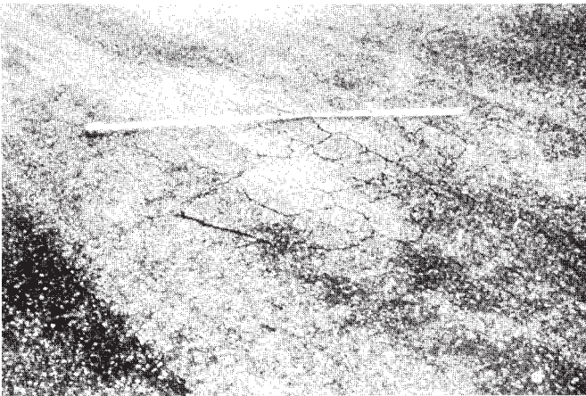
FIG. X1.7 Medium-Severity Alligator Cracking, Approaching High Severity (Example 1)
