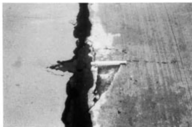
FIG. X2.66 Medium-Severity Joint Spall
