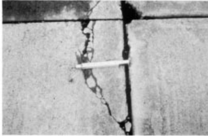
FIG. X2.72 Medium-Severity Corner Spall
