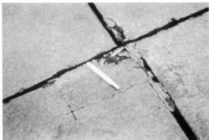
FIG. X2.30 Medium-Severity Small Patch
