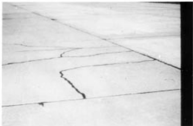
FIG. X2.55 Low-Severity Intersecting Cracks
