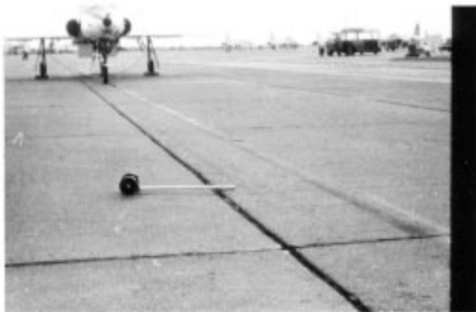
FIG. X2.50 Low-Severity Settlement on Apron
