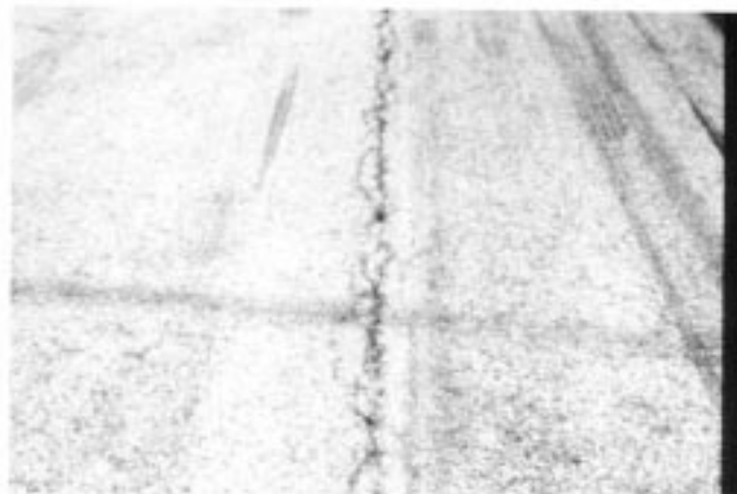
FIG. X1.39 Medium-Severity Longitudinal Construction Joint Crack
