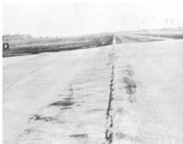
FIG. X1.71 Shove of Low Severity on the Outside and Medium Severity in the Middle
