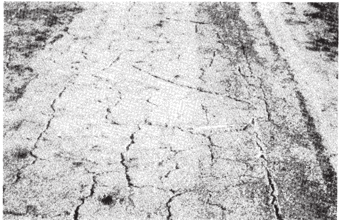
FIG. X1.20 High-Severity Block Cracking
