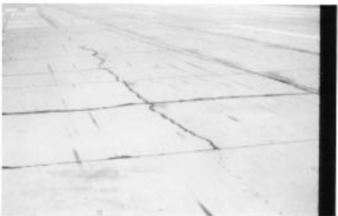
FIG. X2.54 Low-Severity Intersecting Cracks
