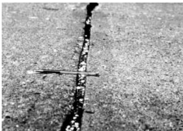
FIG. X2.18 High-Severity Joint Seal Damage
