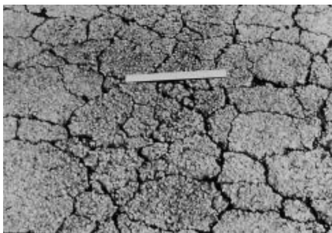
FIG. X1.3 High-Severity Alligator Cracking
