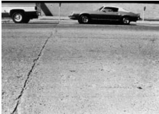
FIG. X2.48 Low-Severity Spalling, Joint
