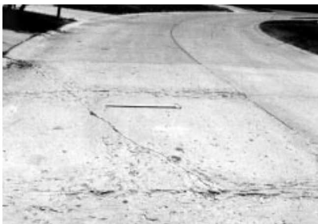
FIG. X2.12 High-Severity Durability Cracking
