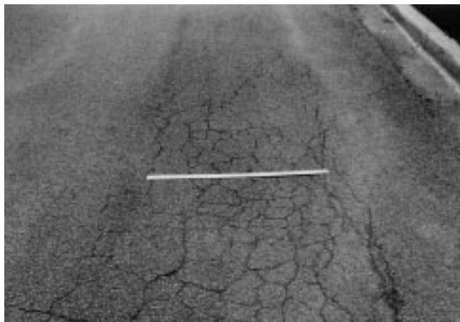
FIG. X1.2 Medium-Severity Alligator Cracking
