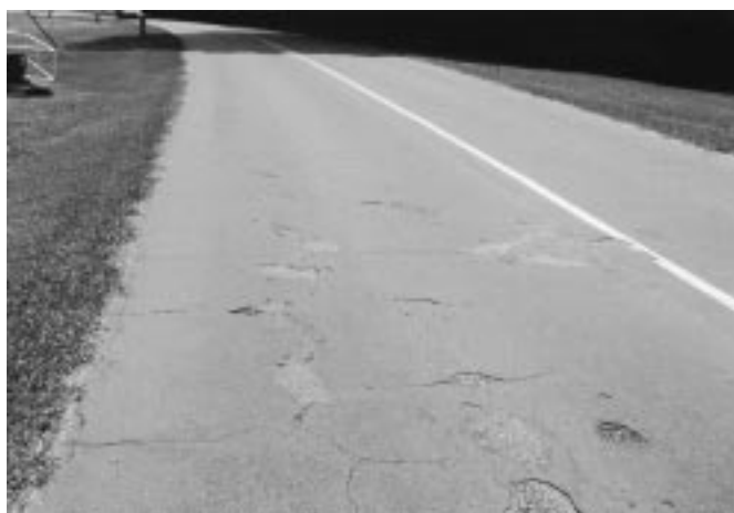
FIG. X1.53 High-Severity Weathering and Raveling
