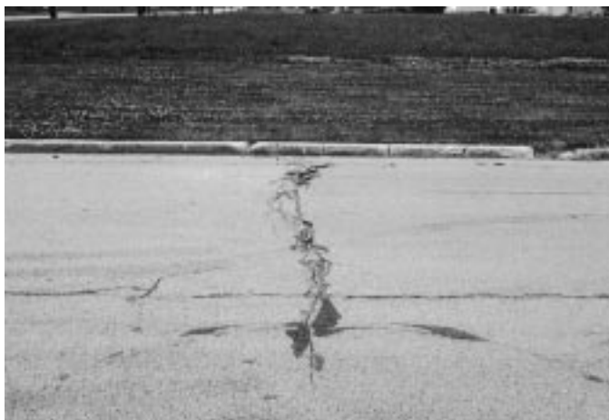
FIG. X1.30 High-Severity Longitudinal and Transverse Cracking
