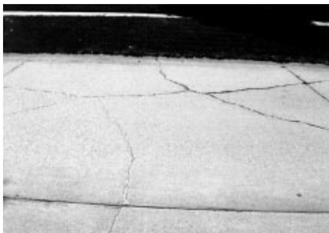
FIG. X2.8 Medium-Severity Divided Slab
