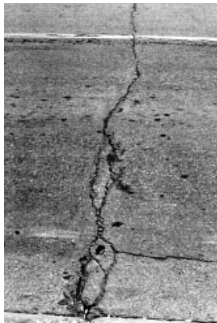
FIG. X1.23 Medium-Severity Joint Reflection Cracking
