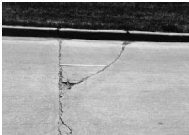
FIG. X2.5 Medium-Severity Corner Break
