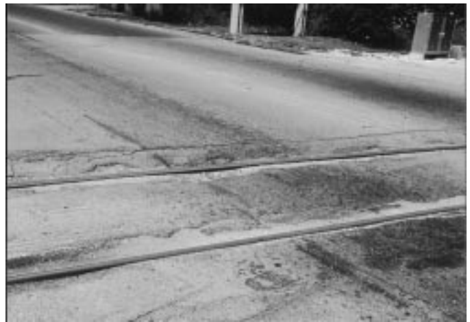
FIG. X1.39 Medium-Severity Railroad Crossing
