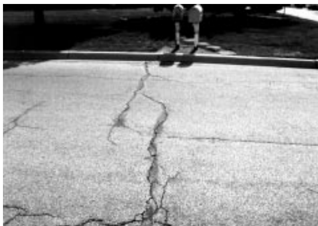
FIG. X1.8 Medium-Severity Block Cracking
