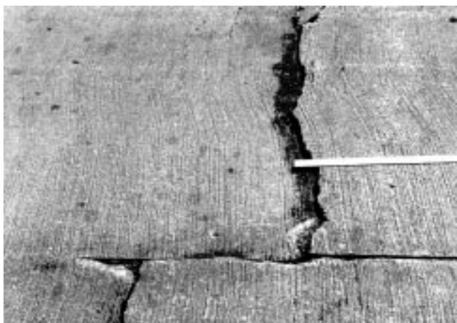
FIG. X2.24 High-Severity Linear Cracking
