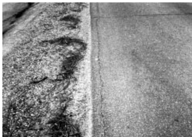
FIG. X1.19 Low-Severity Edge Cracking
