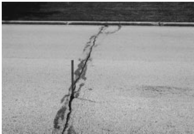
FIG. X1.29 Medium-Severity Longitudinal and Transverse Cracking
