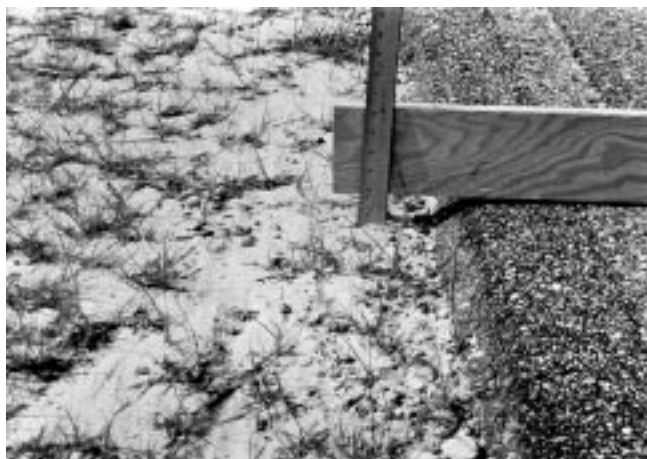
FIG. X1.25 Low-Severity Lane/Shoulder Drop-Off
