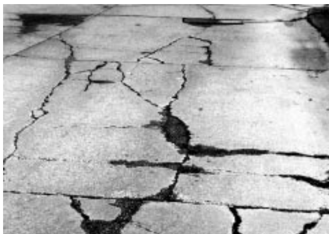
FIG. X2.9 High-Severity Divided Slab
