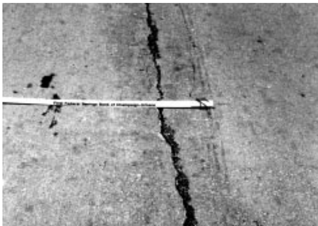
FIG. X2.23 Medium-Severity Linear Cracking
