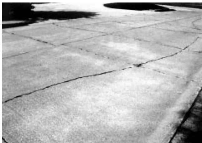
FIG. X2.7 Low-Severity Divided Slab
