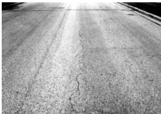
FIG. X1.1 Low-Severity Alligator Cracking
