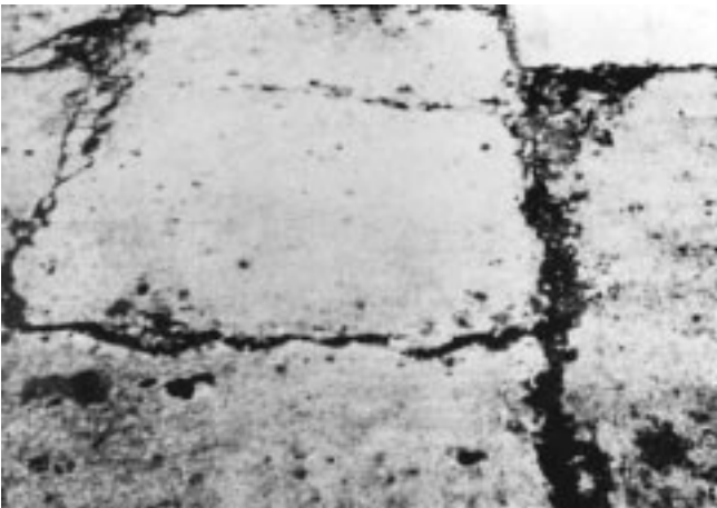
FIG. X2.27 High-Severity Patching, Large and Utility Cuts
