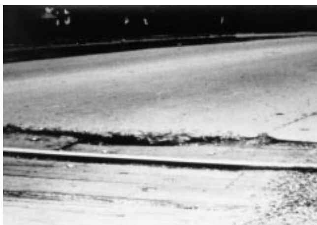
FIG. X2.40 High-Severity Railroad Crossing
