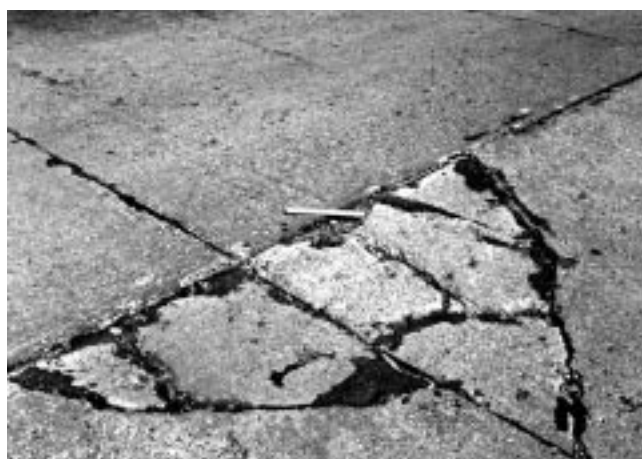
FIG. X2.6 High-Severity Corner Break
