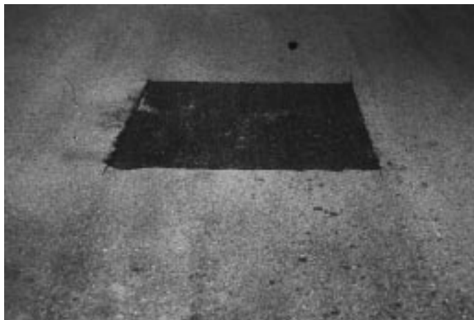
FIG. X1.31 Low-Severity Patching and Utility Cut Patching
