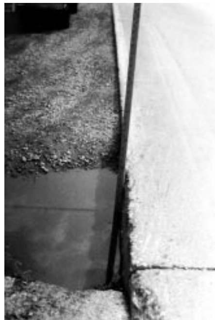
FIG. X2.21 High-Severity Lane/Shoulder Drop-Off
