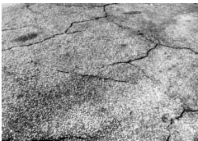
FIG. X1.9 High-Severity Block Cracking
