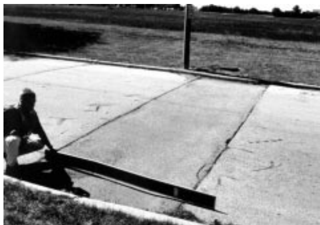
FIG. X1.32 Medium-Severity Patching and Utility Cut Patching
