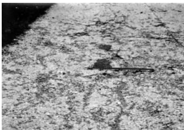
FIG. X2.43 High-Severity Scaling, Map Cracking, and Crazing
