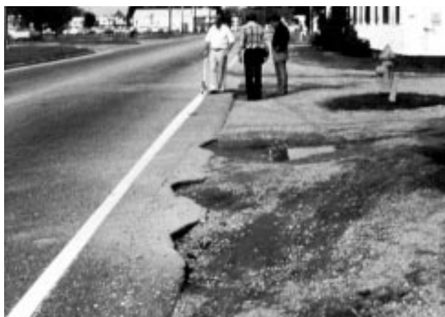
FIG. X1.21 High-Severity Edge Cracking
