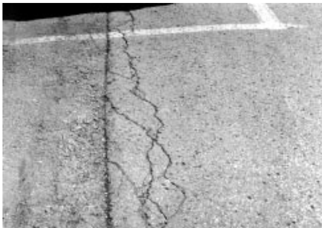
FIG. X1.20 Medium-Severity Edge Cracking
