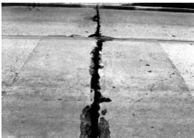
FIG. X2.16 Low-Severity Joint Seal Damage
