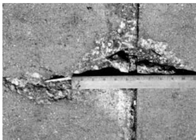
FIG. X2.46 Medium-Severity Spalling, Corner
