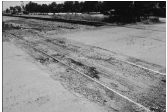
FIG. X1.40 High-Severity Railroad Crossing
