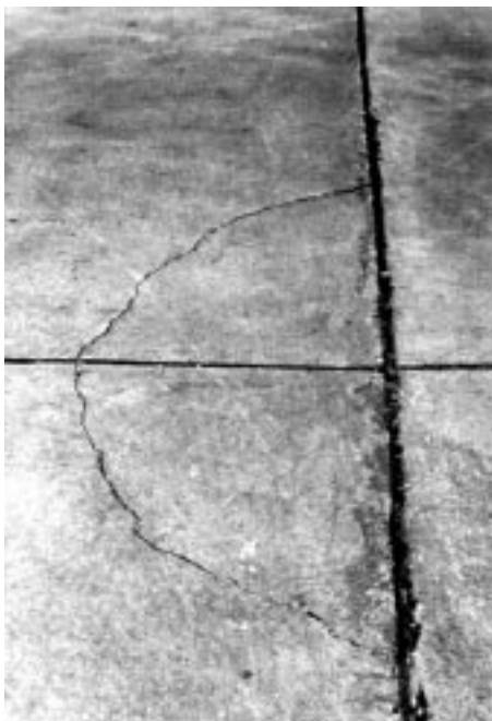
FIG. X2.4 Low-Severity Corner Break
