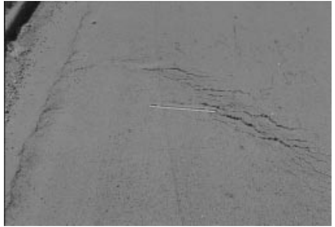
FIG. X1.48 Medium-Severity Slippage Cracking
