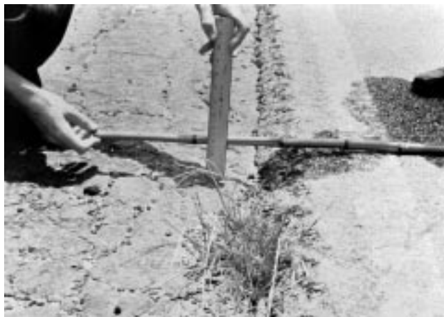
FIG. X1.26 Medium-Severity Lane/Shoulder Drop-Off
