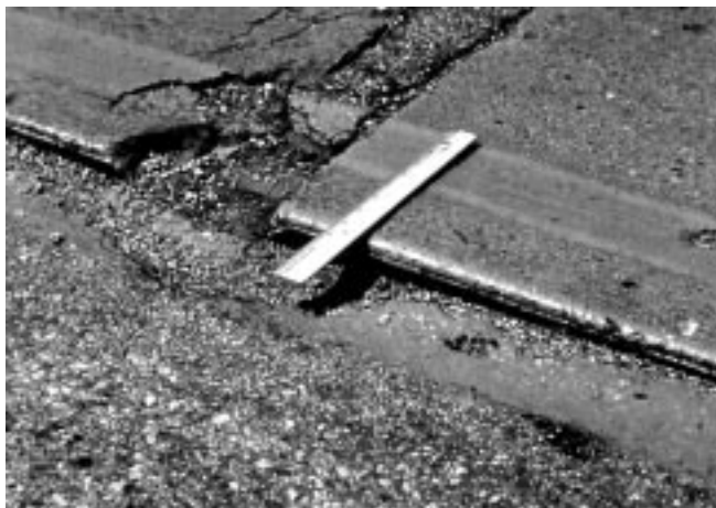
FIG. X2.19 Low-Severity Lane/Shoulder Drop-Off
