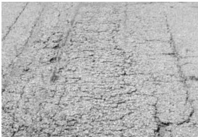
FIG. X1.52 Medium-Severity Weathering and Raveling
