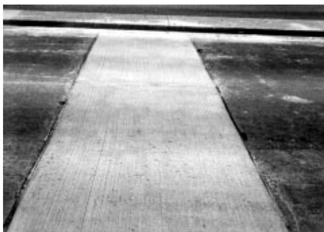
FIG. X2.25 Low-Severity Patching, Large and Utility Cuts
