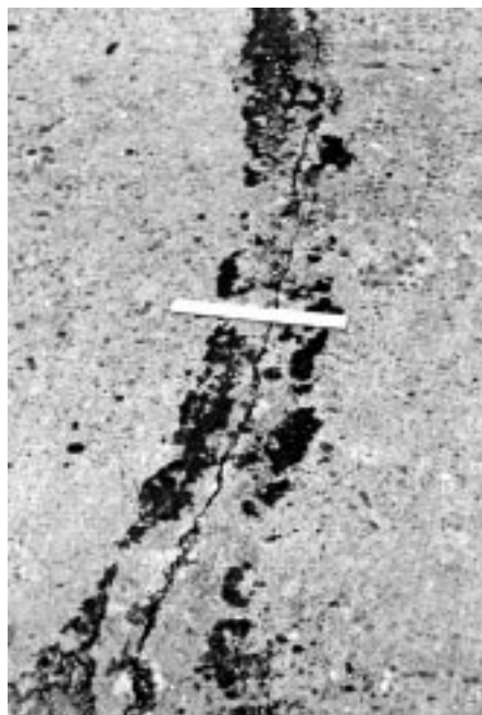
FIG. X2.22 Low-Severity Linear Cracking
