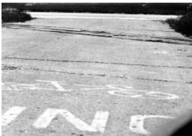
FIG. X2.39 Medium-Severity Railroad Crossing
