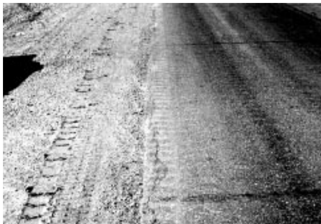
FIG. X1.22 Low-Severity Joint Reflection Cracking
