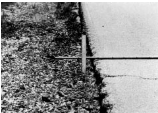
FIG. X1.27 High-Severity Lane/Shoulder Drop-Off
