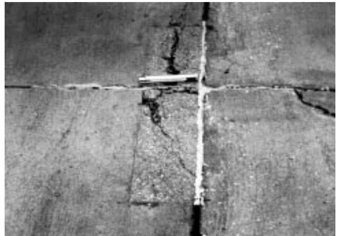
FIG. X2.30 High-Severity Patching, Small
