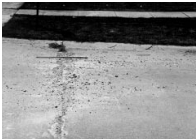
FIG. X2.1 Low Severity Blowup/Buckling
