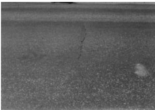
FIG. X1.28 Low-Severity Longitudinal and Transverse Cracking
