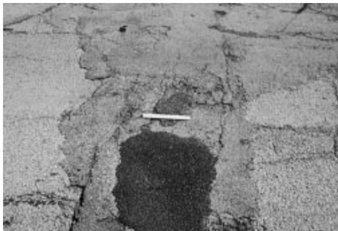
FIG. X1.33 High-Severity Patching and Utility Cut Patching
