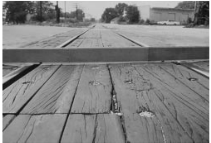
FIG. X1.38 Low-Severity Railroad Crossing
