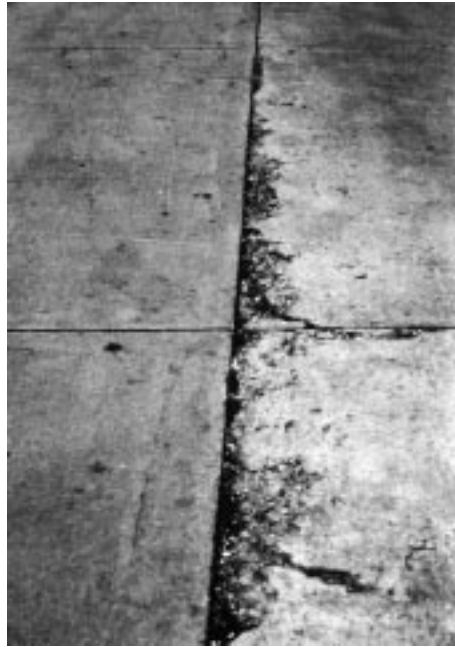
FIG. X2.49 Medium-Severity Spalling, Joint
