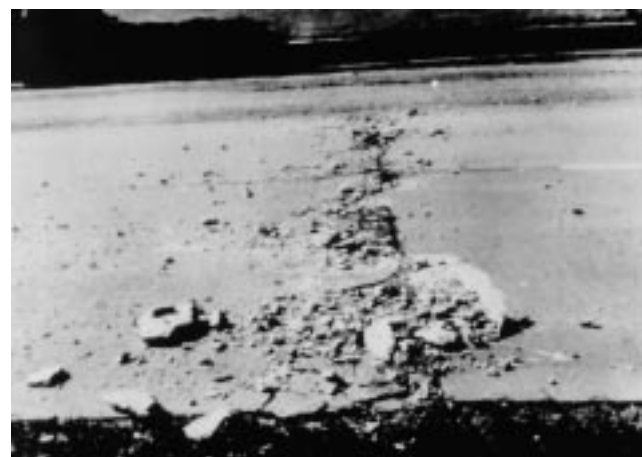
FIG. X2.2 Medium Severity Blowup/Buckling
