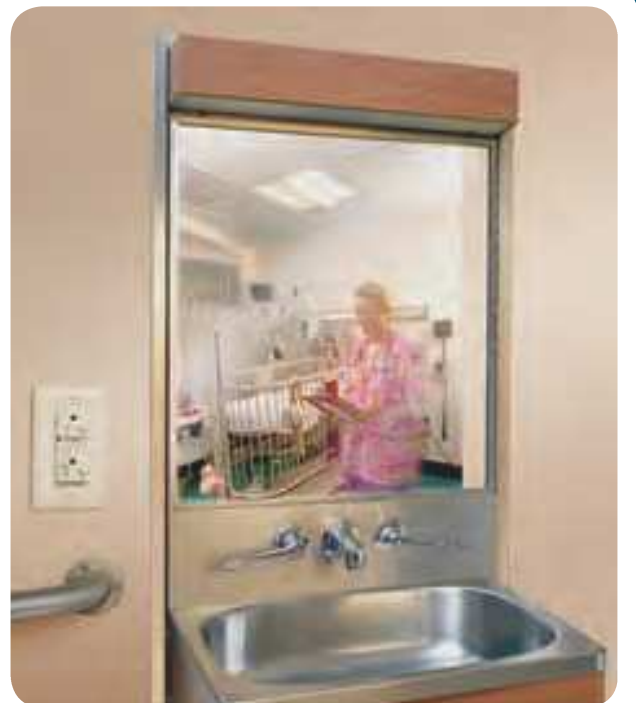
EXHIBIT 517.3 Hospital grade tamper-resistant GFCI in a hospital environment. (Courtesy of Legrand/Pass & Seymour®)
