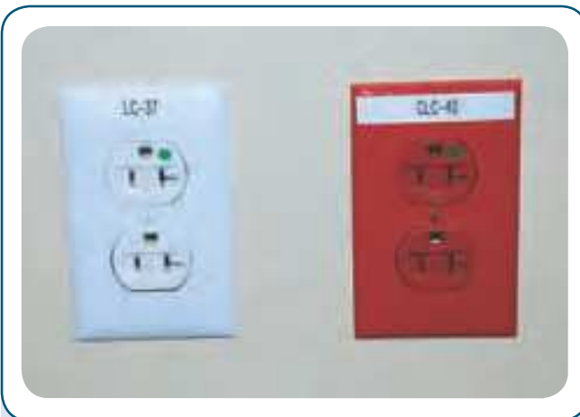
EXHIBIT 517.4 A receptacle from the normal system (left) and the emergency system (right). Note the label that indicates the panelboard and the circuit number. (Courtesy of the International Association of Electrical Inspectors)
