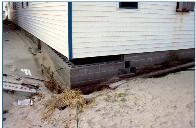
Failure of crawlspace foundation undermined by scour.
