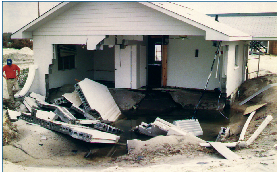
Building failure caused by undermining of slab-on-grade foundation during Hurricane Fran.
