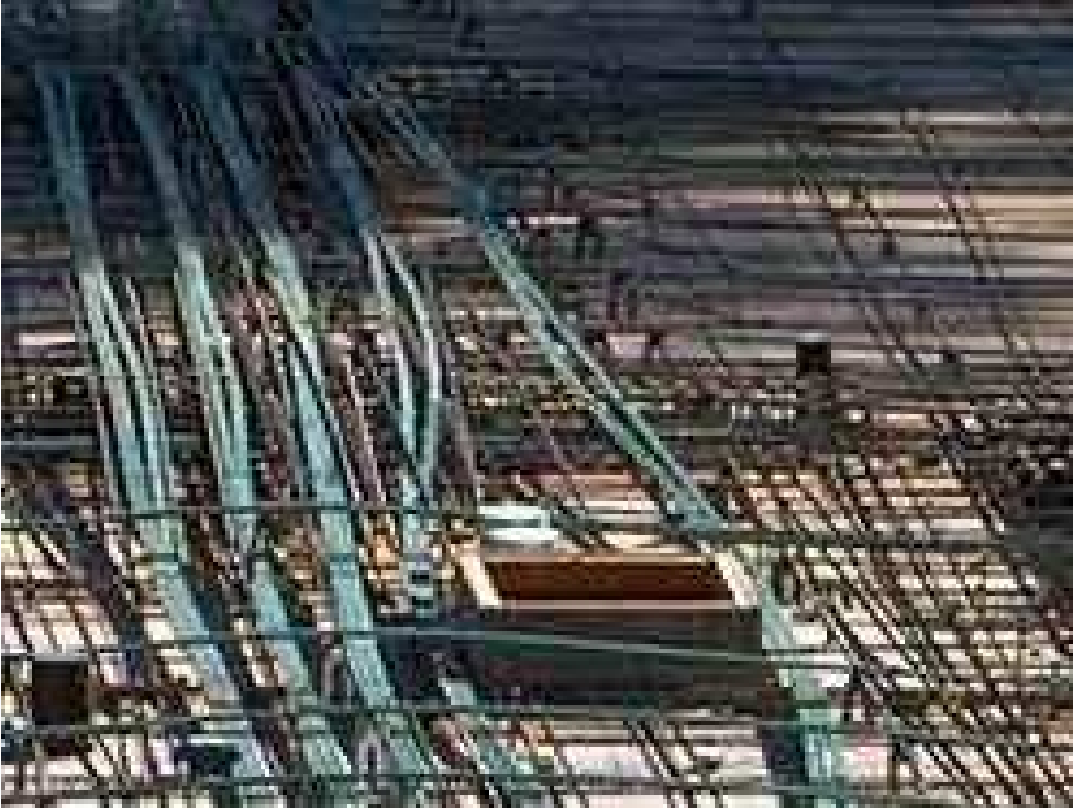
Even congested tendons can be routed around obstructions. Digital Concrete Scanning Services
