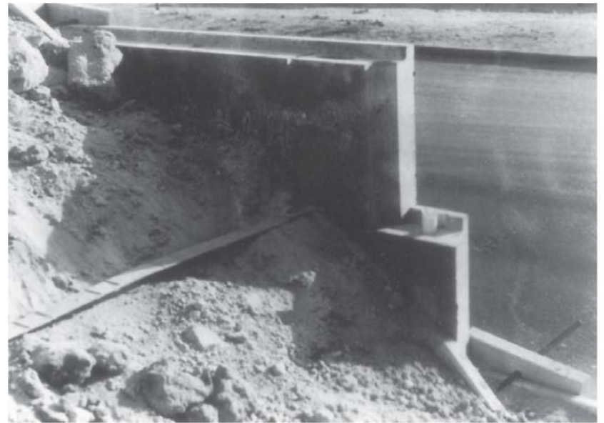
Figure 8.28 Metallic strip attachment to the precast concrete slab used as the skin (Courtesy of Braja M. Das, Henderson, NV)
