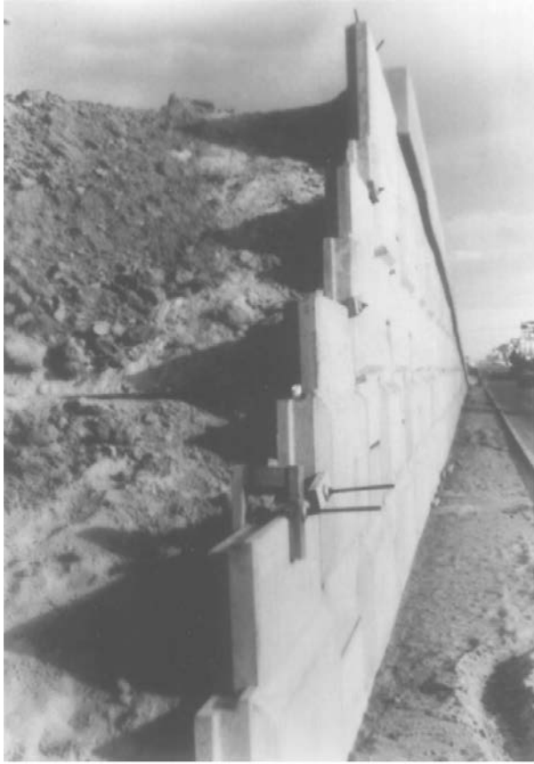
Figure 8.26 Reinforced-earth retaining wall (with metallic strip) under construction (Courtesy of Braja M. Das, Henderson, NV)
