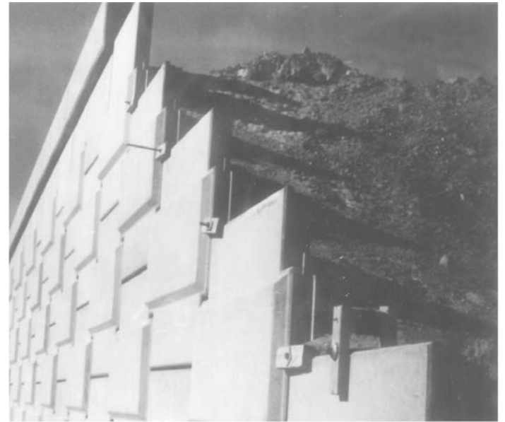
Figure 8.27 Another view of the retaining wall shown in Figure 8.26 (Courtesy of Braja M. Das, Henderson, NV)
