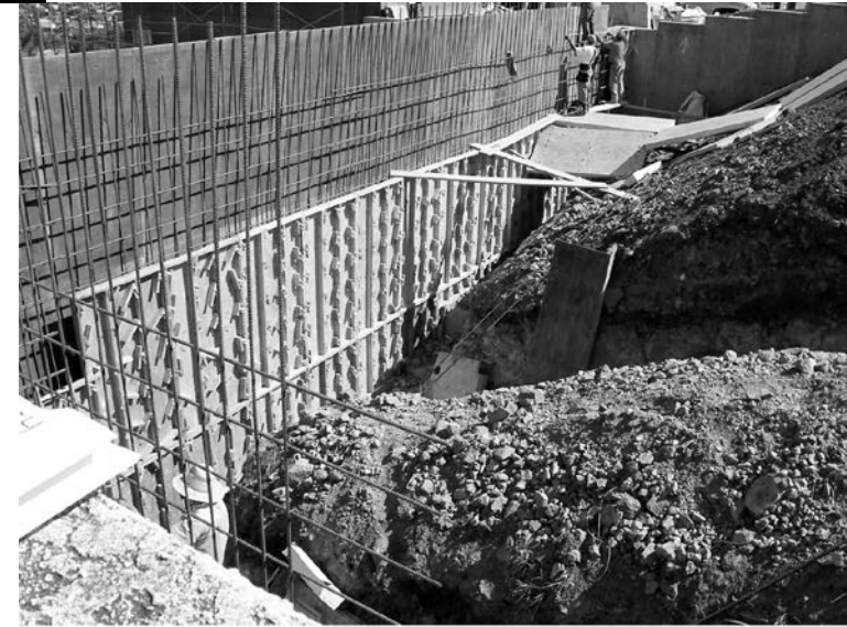
Figure 8.2 A cantilever retaining wall under construction (Courtesy of Dharma Shakya, Geotechnical Solutions, Inc., Irvine, California)
