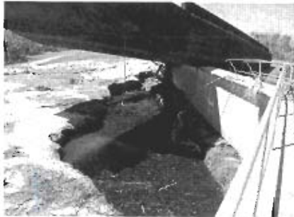
Scour Hole at BV Control Structure
