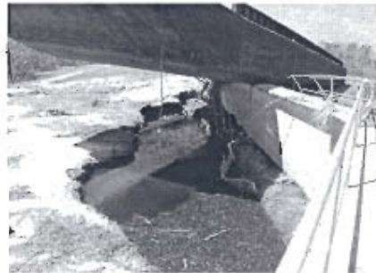
Scour Hole at BV Control Structure
