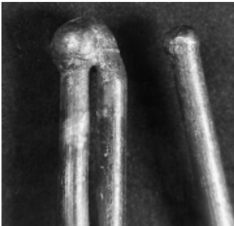
FIGURE 6.10.3(b) Copper conductors severed by arcing through the charred insulation with a large bead welding the two conductors together.
