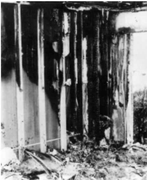
FIGURE 4.17.1 Typical V pattern showing wall and wood stud damage.
