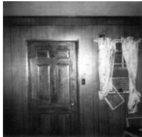
FIGURE 4.19.2 Blistering of varnish on door and slight scorching of draperies, the only indications of the natural gas flash fire.
