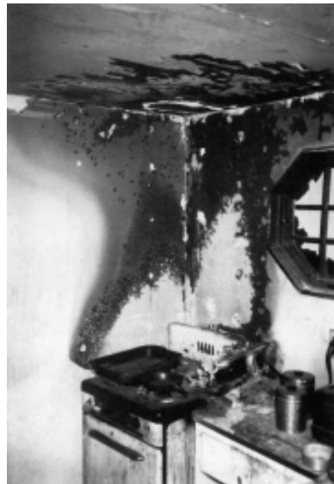
FIGURE 4.11 Clean burn on wall surface.
