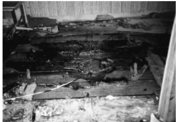
FIGURE 4.17.10 Saddle burn in a floor joist.
