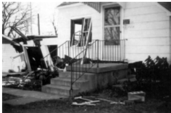
FIGURE 18.3.1 Low-order damage in a dwelling.
