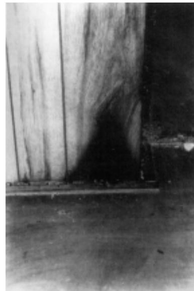
FIGURE 4.17.2.2 Inverted cone pattern fueled by a natural gas leak below the floor level.
