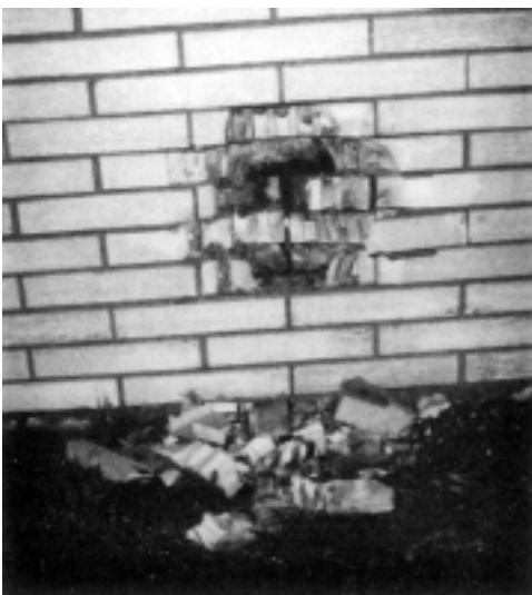
FIGURE 4.20.2 Damage to an outside brick wall caused by thermal expansion of an I-beam in the basement.
