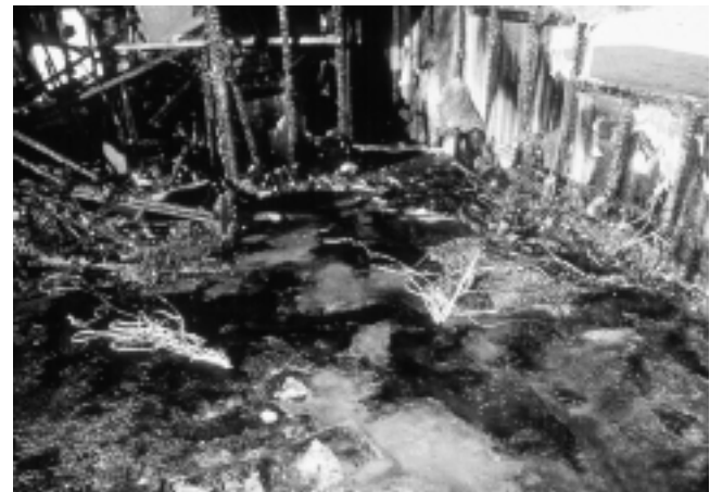
FIGURE 4.17.7.2(a) Irregular burn patterns on a floor of a room burned in a test fire in which no ignitable liquids were used.
