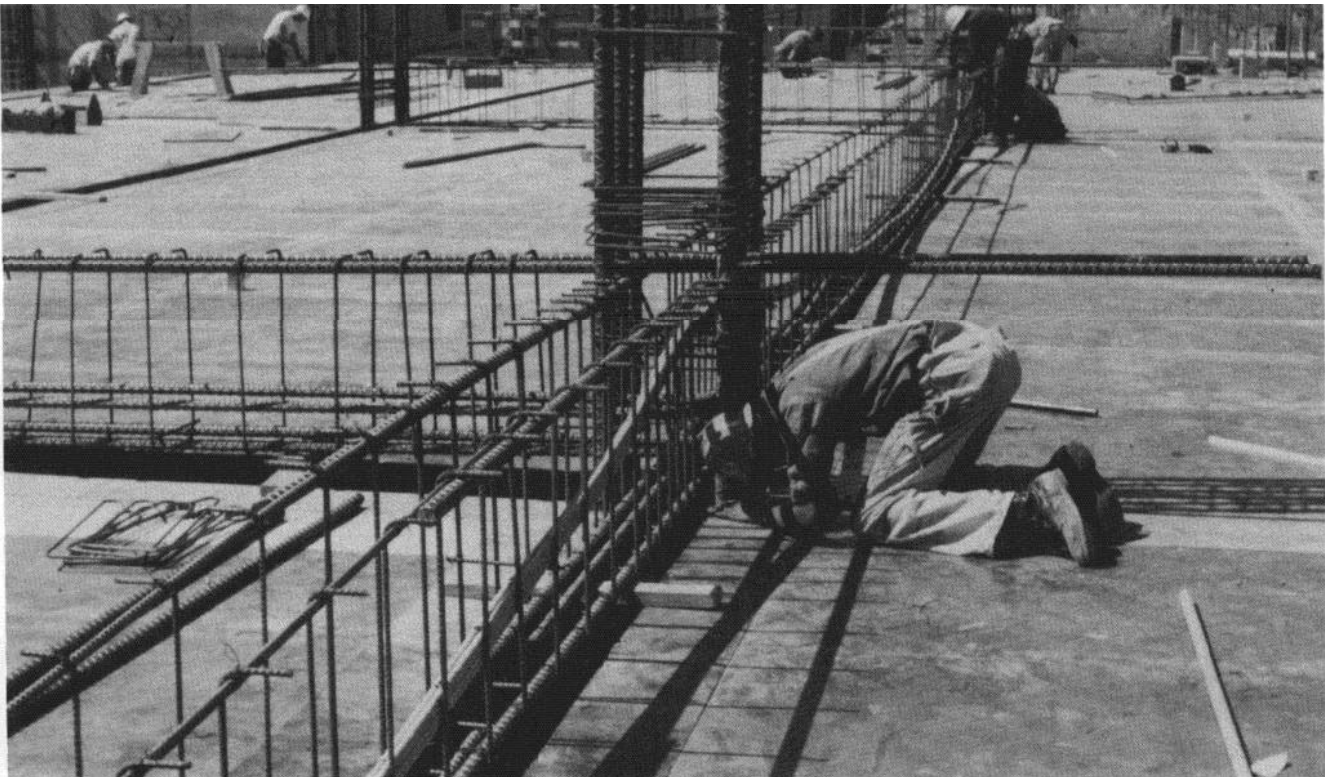
Fig. 6.5 — Fabrication of conventional reinforcement and post-tensioning tendons in beams as detailed in Fig. 6.4.
