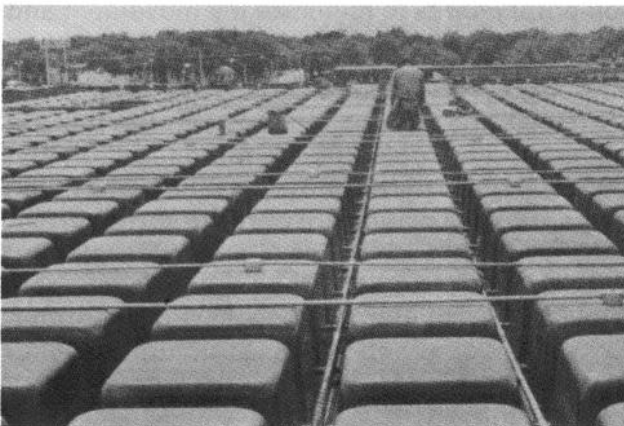
Fig. 6.19 — Tendons in place in a waffle slab as final preparations are made for concrete placement.
