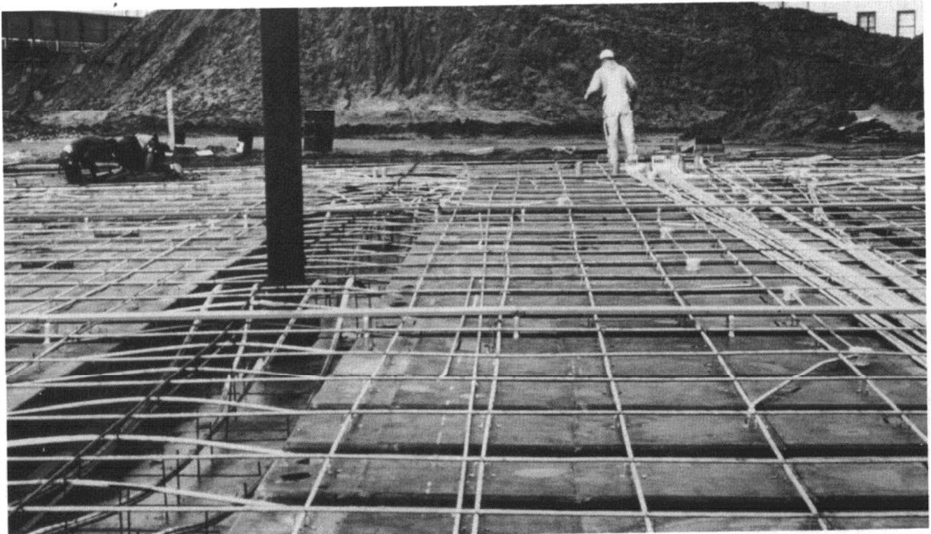
Fig. 6.8 — Construction view of forming and tendon installation for a one-way joist building.
