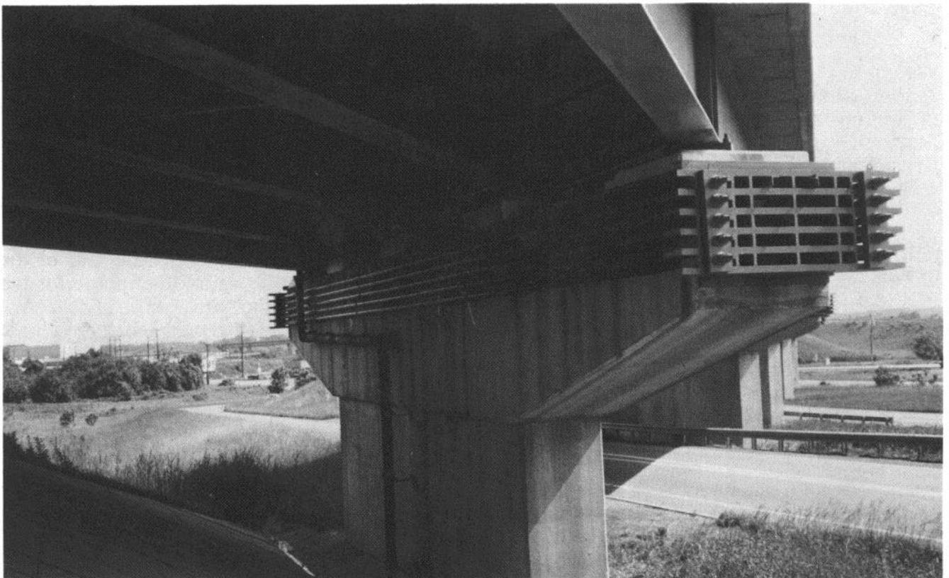
Fig. 1.64 — Repair and Strengthening of pier caps by use of external post-tensioning. Route 695 Bridge over Route 151. Baltimore, Maryland.
