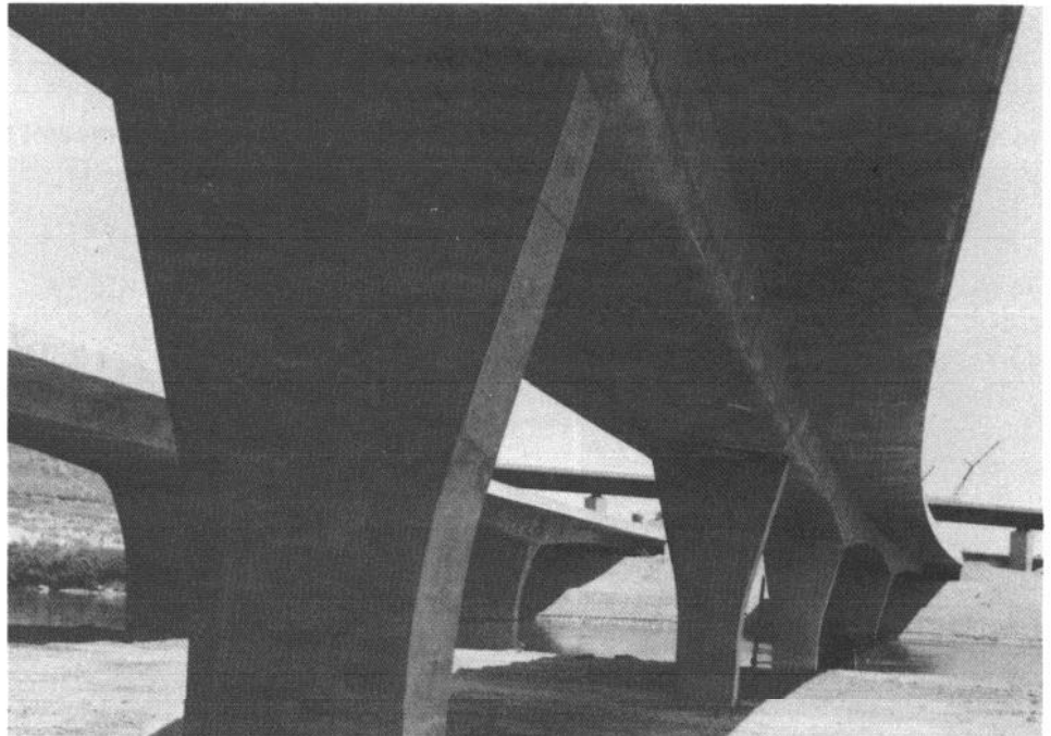
Fig. 1.45 — Yakima River Bridge, SR 182, Benton County, Oregon. Spans range from 140 ft. to 215 ft.
