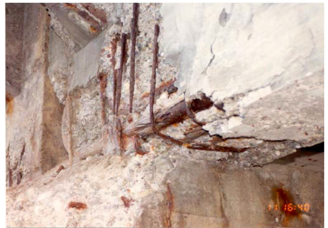
Fig. 1—Example of severe reinforcing steel deterioration due to corrosion in a reinforced concrete beam (courtesy of the Ministry of Transportation of Quebec).
