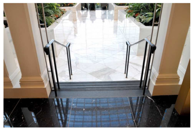
Tread cover striping clearly indicates the location of each tread edge. (Photo courtesy of Jake Pauls)
