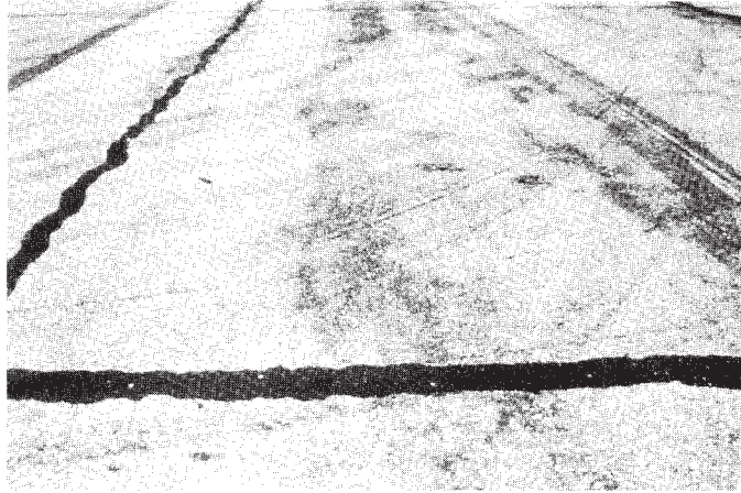
FIG. X1.31 Low-Severity Joint Reflection Cracking, Filled Crack
