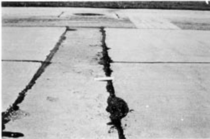
FIG. X2.36 Medium-Severity Utility Cut
