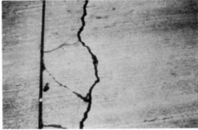
FIG. X2.65 Medium-Severity Joint Spall
