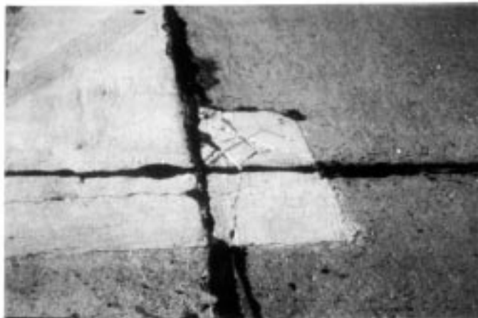
FIG. X2.31 Medium-Severity Small Patch
