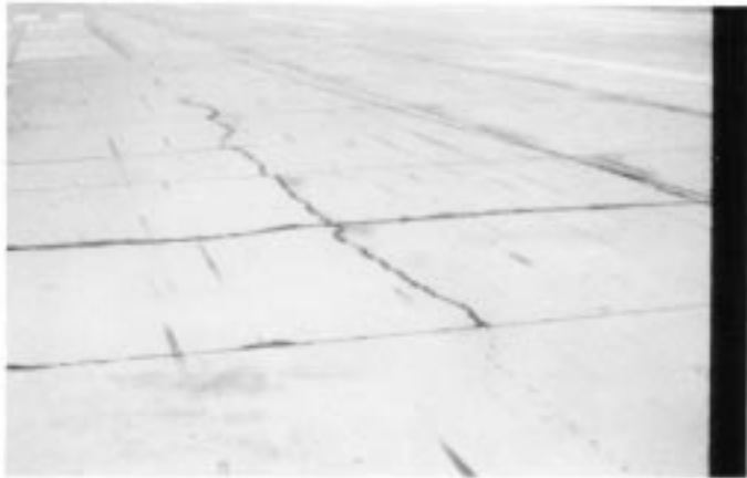
FIG. X2.54 Low-Severity Intersecting Cracks
