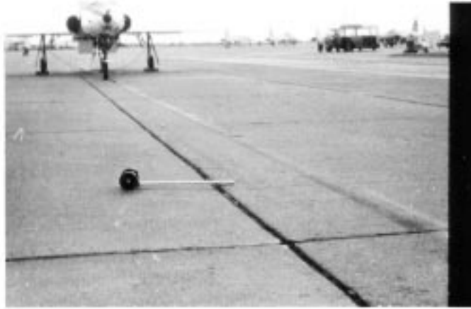
FIG. X2.50 Low-Severity Settlement on Apron
