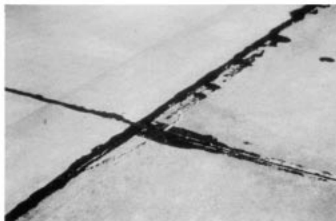
FIG. X2.70 Low-Severity Corner Spall
