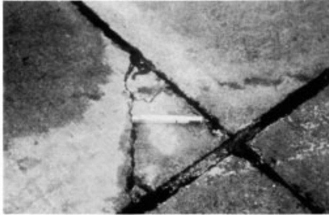
FIG. X2.71 Medium-Severity Corner Spall
