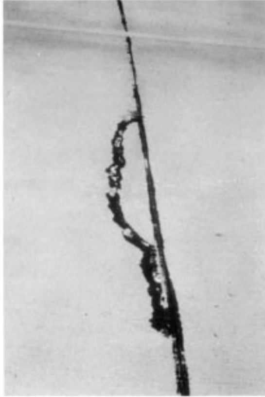
FIG. X2.63 Low-Severity Joint Spall
