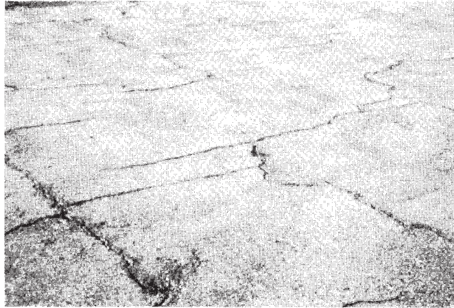
FIG. X1.17 Medium-Severity Block Cracking
