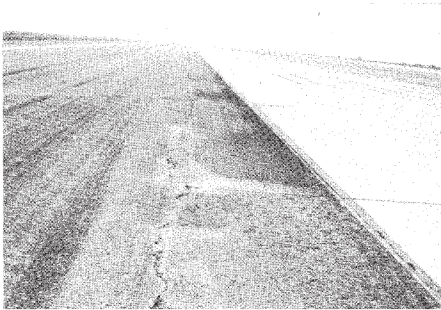
FIG. X1.41 Medium-Severity Longitudinal Crack
