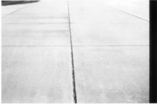
FIG. X2.40 Pumping (Note Stains on Pavement)
