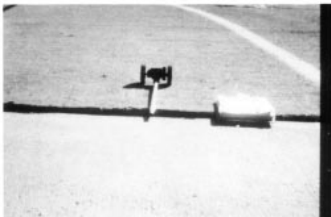
FIG. X2.52 High-Severity Settlement on Taxiway/Runway ( 3/4 in. (18 mm))
