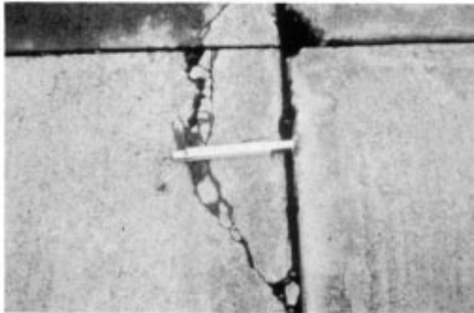
FIG. X2.72 Medium-Severity Corner Spall
