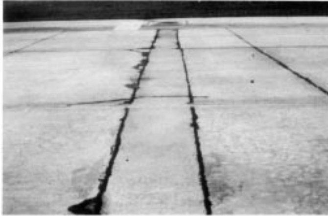
FIG. X2.35 Low-Severity Utility Cut
