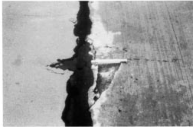
FIG. X2.66 Medium-Severity Joint Spall
