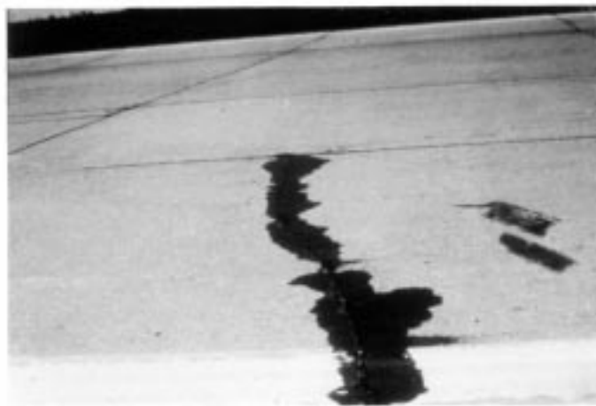
FIG. X2.13 Medium-Severity Transverse Crack
