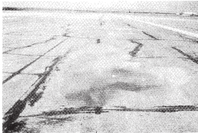
FIG. X1.27 High-Severity Depression (2 in. (50 mm))
