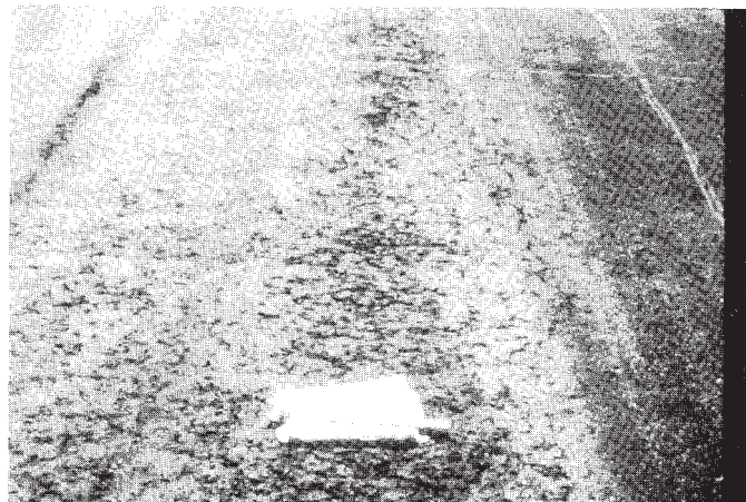
FIG. X1.56 Low-Severity Raveling/Weathering, Approaching Medium Severity
