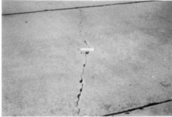
FIG. X2.14 Medium-Severity Transverse Crack
