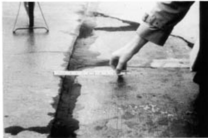
FIG. X2.51 Medium-Severity Settlement on Apron ( >1/2 in. (13 mm))
