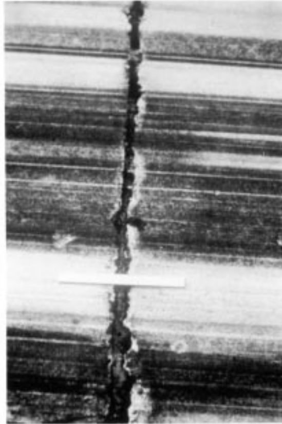
FIG. X2.62 Low-Severity Joint Spalling (if the Frayed Area was Less Than 2 ft (0.6 m) Long it Would not be Counted)
