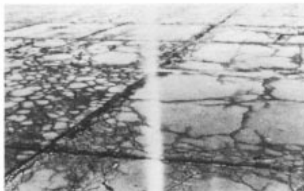
FIG. X2.48 High-Severity Scaling Caused by Alkali Aggregate Reaction
