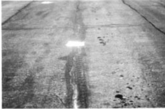
FIG. X1.40 Medium-Severity Longitudinal Crack (Note the Crack is Reflective But Not at the Joint of Slab)
