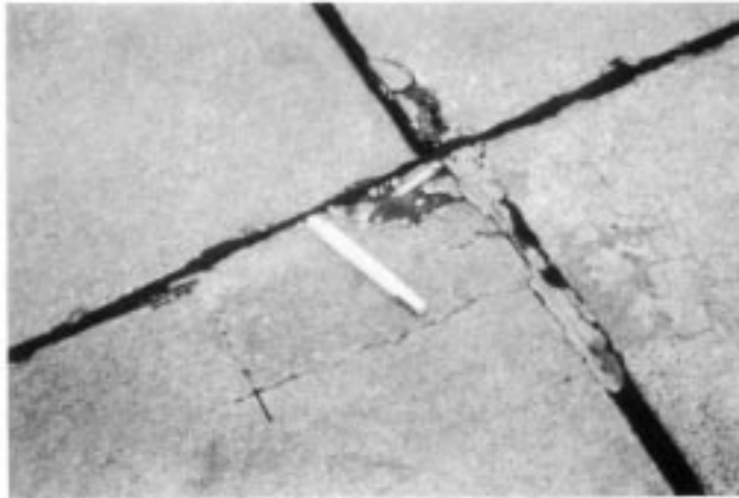
FIG. X2.30 Medium-Severity Small Patch
