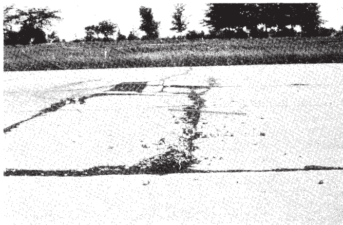
NOTE 1—This would only be considered low severity if the shattering in the foreground was the only part existing and the foreign material removed.
