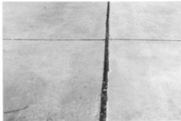
FIG. X2.26 High-Severity Joint Seal Damage (Complete Loss of Sealant; Joint is Filled with Incompressible Material)
