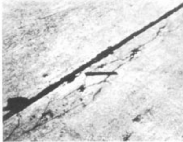
FIG. X2.20 Medium-Severity "D" Cracking
