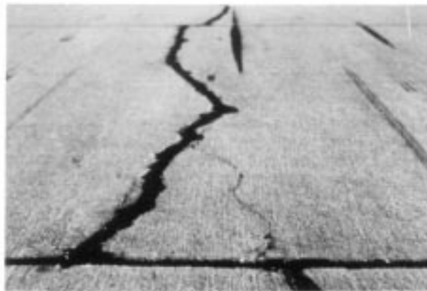
FIG. X2.16 High-Severity Longitudinal Cracks
