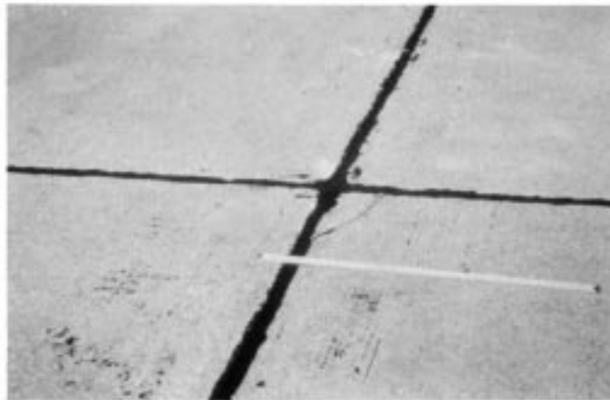
FIG. X2.69 Low-Severity Corner Spall
