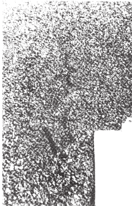
FIG. X1.44 Medium-Severity Crack in Porous Friction Course
