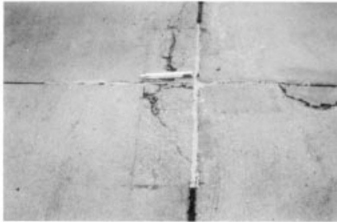
FIG. X2.32 High-Severity Small Patch
