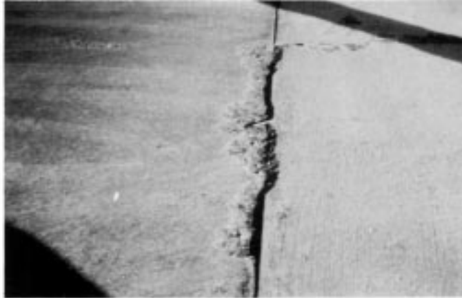
FIG. X2.68 High-Severity Joint Spall
