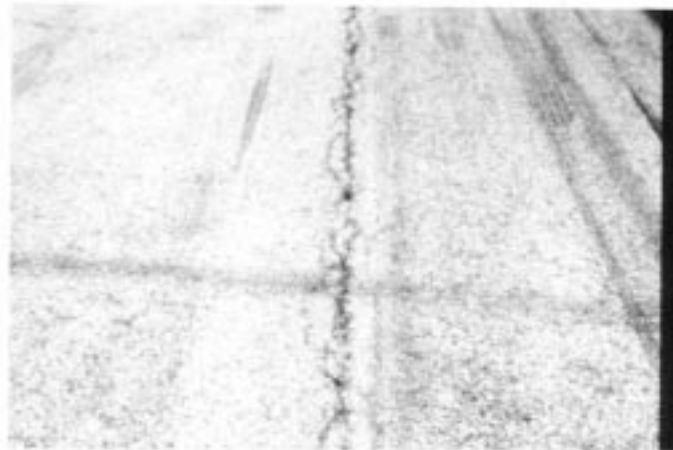
FIG. X1.39 Medium-Severity Longitudinal Construction Joint Crack
