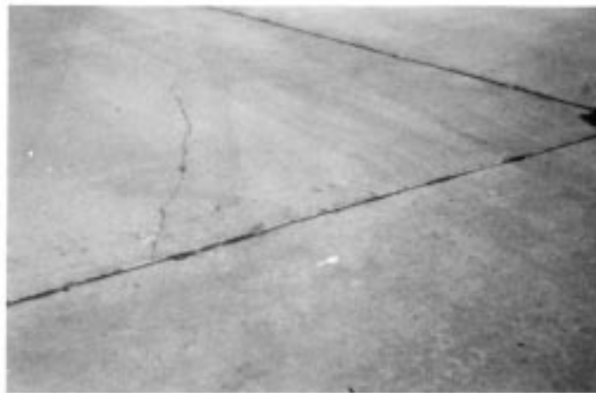
FIG. X2.11 Low-Severity Diagonal Crack
