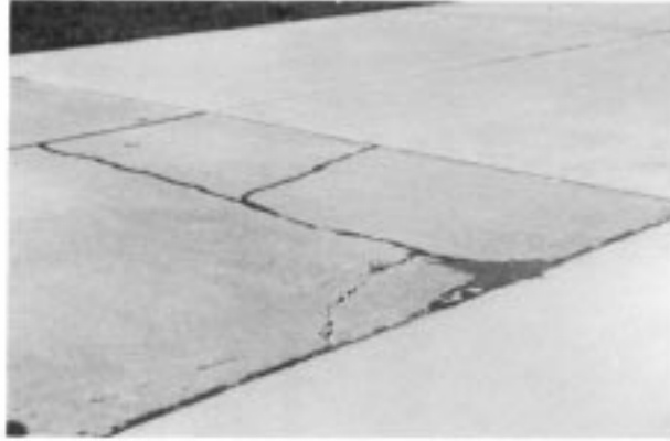
FIG. X2.56 Medium-Severity Intersecting Cracks
