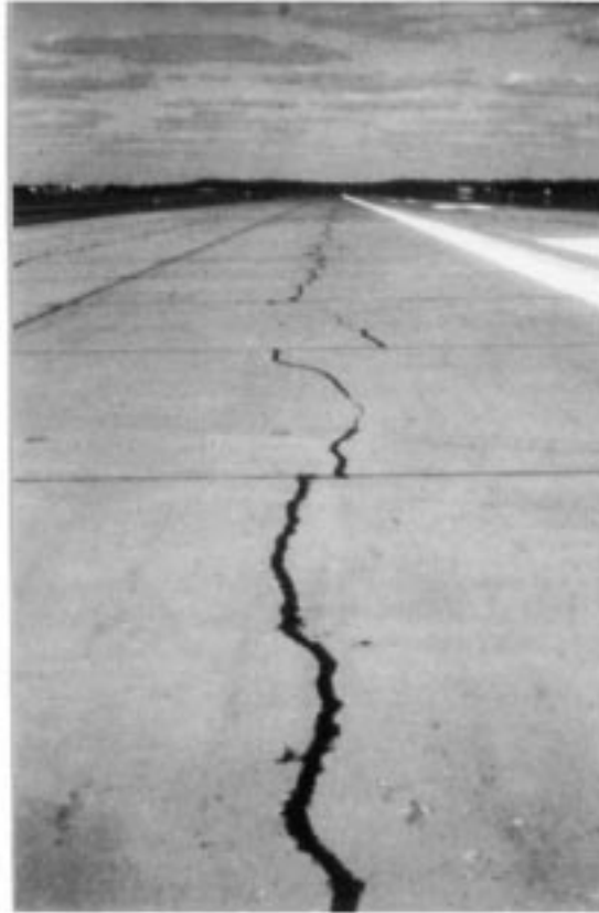
FIG. X2.12 Medium-Severity Longitudinal Crack
