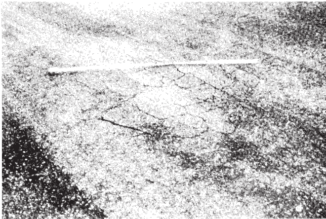
FIG. X1.7 Medium-Severity Alligator Cracking, Approaching High Severity (Example 1)
