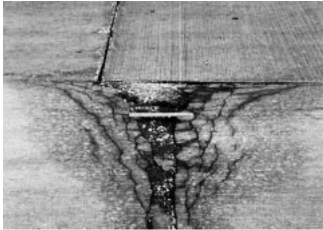
FIG. X2.11 Medium-Severity Durability Cracking
