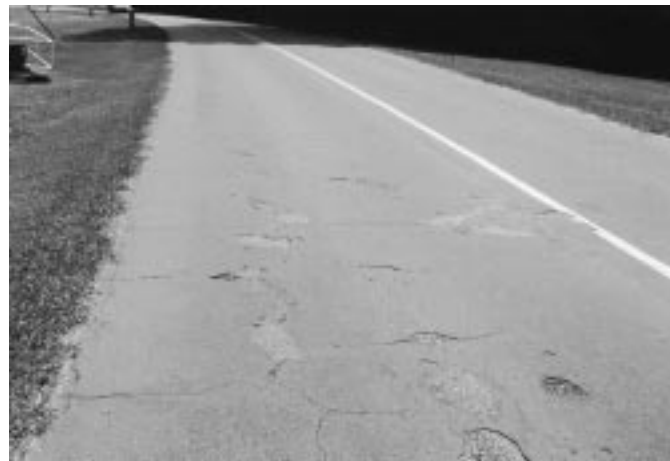
FIG. X1.53 High-Severity Weathering and Raveling
