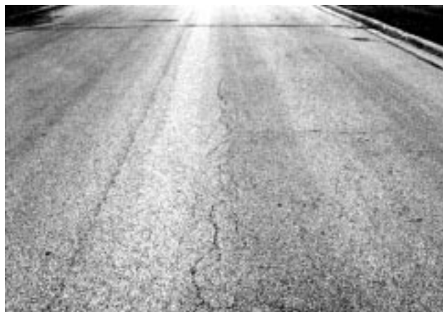
FIG. X1.1 Low-Severity Alligator Cracking
