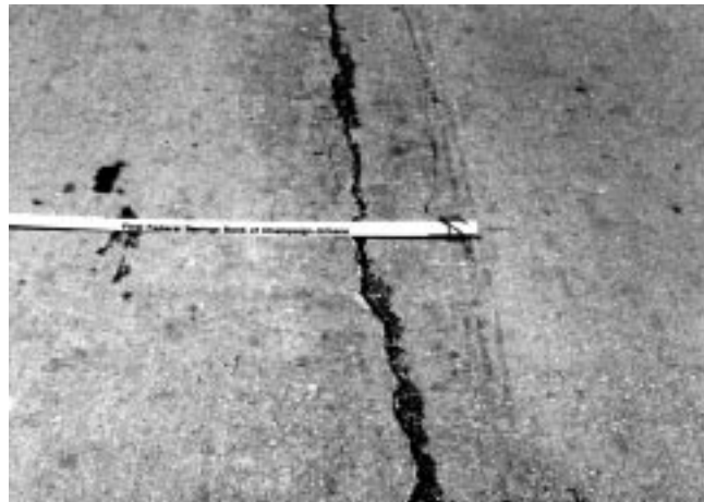
FIG. X2.23 Medium-Severity Linear Cracking
