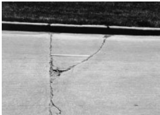
FIG. X2.5 Medium-Severity Corner Break
