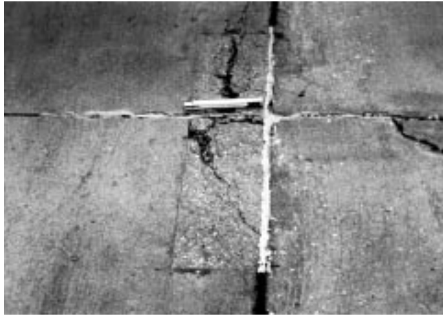
FIG. X2.30 High-Severity Patching, Small
