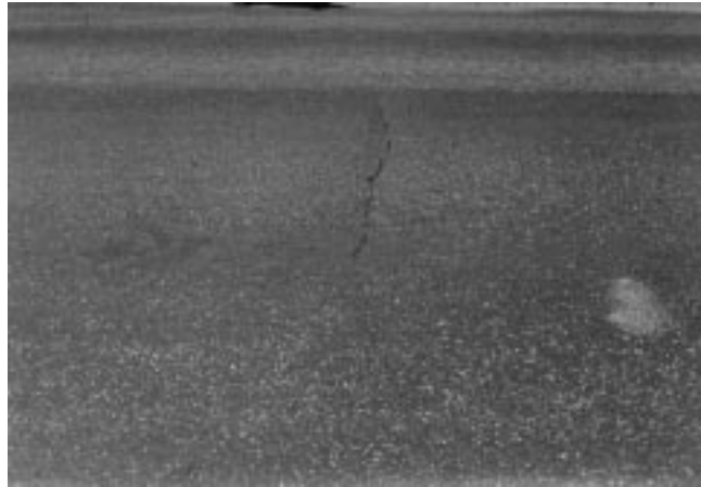
FIG. X1.28 Low-Severity Longitudinal and Transverse Cracking
