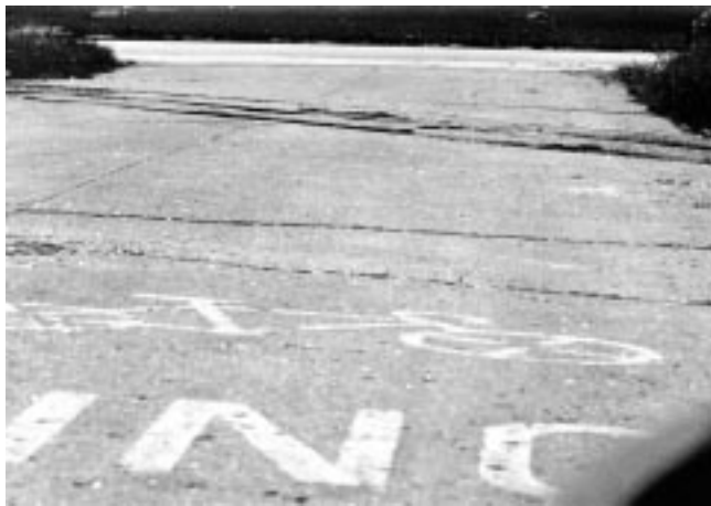
FIG. X2.39 Medium-Severity Railroad Crossing
