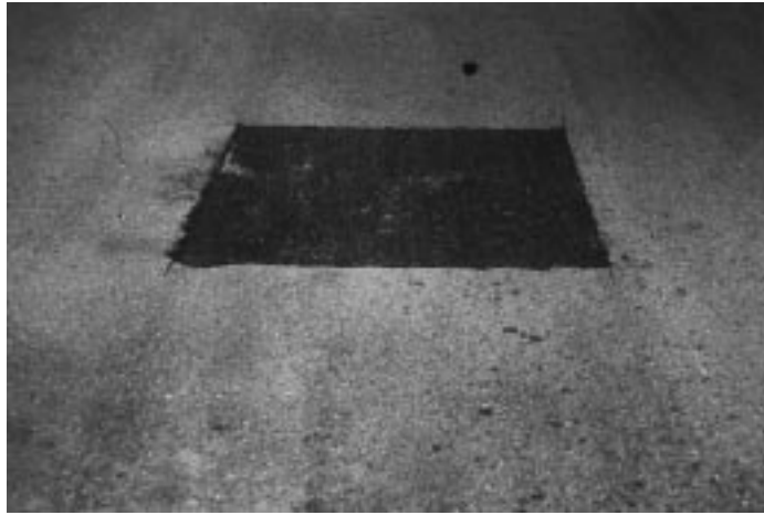
FIG. X1.31 Low-Severity Patching and Utility Cut Patching
