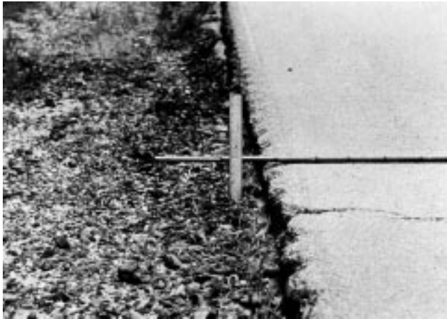
FIG. X1.27 High-Severity Lane/Shoulder Drop-Off
