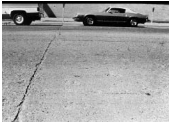
FIG. X2.48 Low-Severity Spalling, Joint
