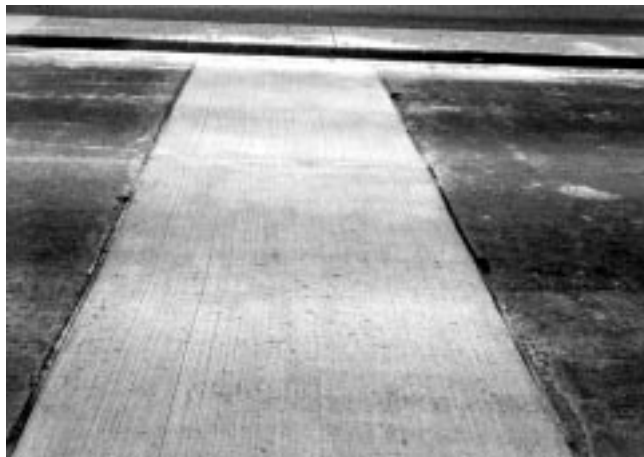
FIG. X2.25 Low-Severity Patching, Large and Utility Cuts
