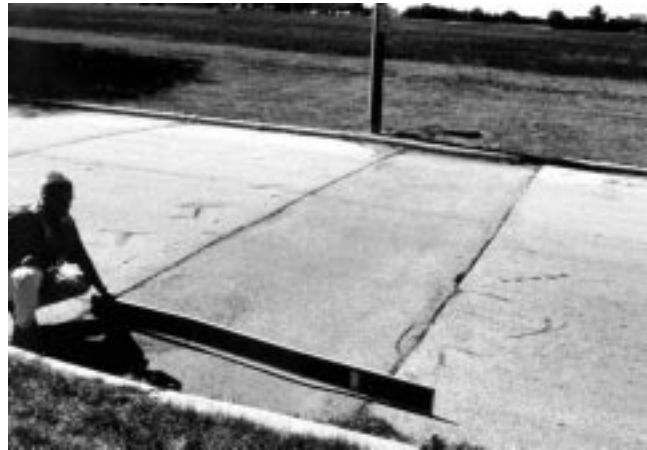
FIG. X1.32 Medium-Severity Patching and Utility Cut Patching
