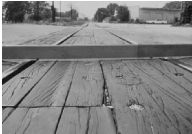
FIG. X1.38 Low-Severity Railroad Crossing
