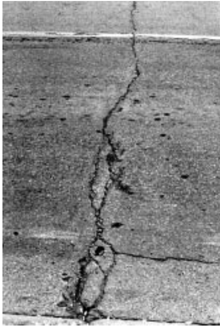
FIG. X1.23 Medium-Severity Joint Reflection Cracking
