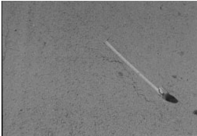
FIG. X1.47 Low-Severity Slippage Cracking
