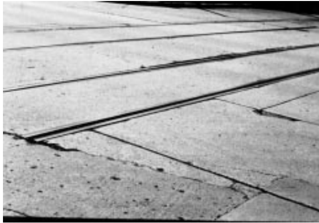
FIG. X2.38 Low-Severity Railroad Crossing
