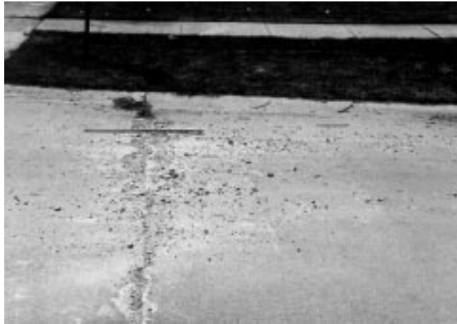
FIG. X2.1 Low Severity Blowup/Buckling
