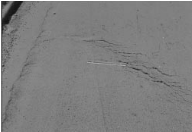
FIG. X1.48 Medium-Severity Slippage Cracking
