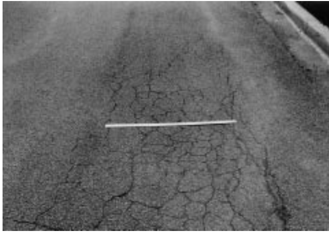
FIG. X1.2 Medium-Severity Alligator Cracking
