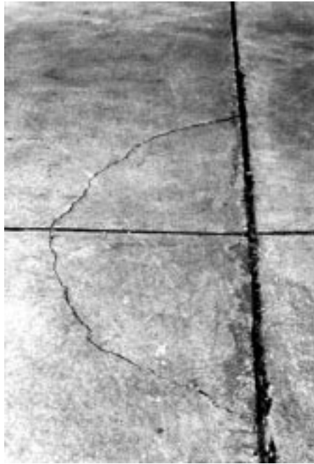
FIG. X2.4 Low-Severity Corner Break
