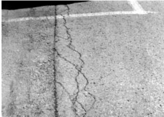
FIG. X1.20 Medium-Severity Edge Cracking
