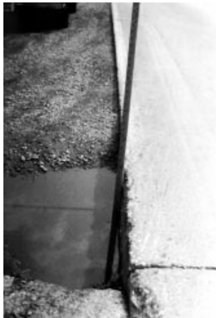
FIG. X2.21 High-Severity Lane/Shoulder Drop-Off
