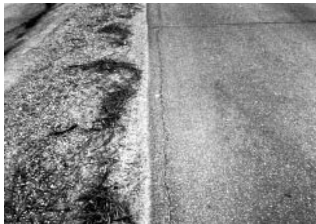
FIG. X1.19 Low-Severity Edge Cracking
