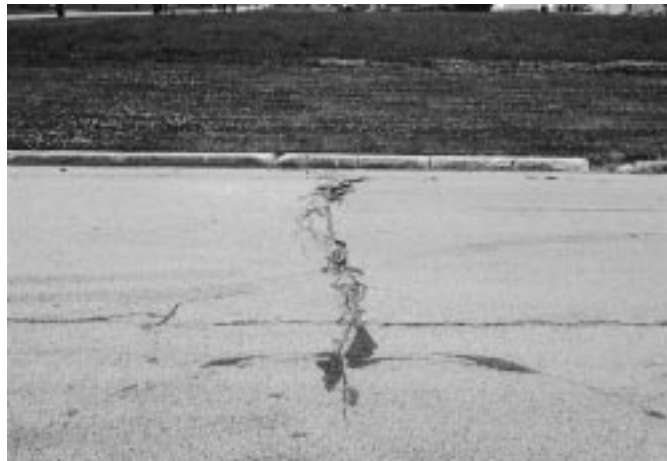
FIG. X1.30 High-Severity Longitudinal and Transverse Cracking
