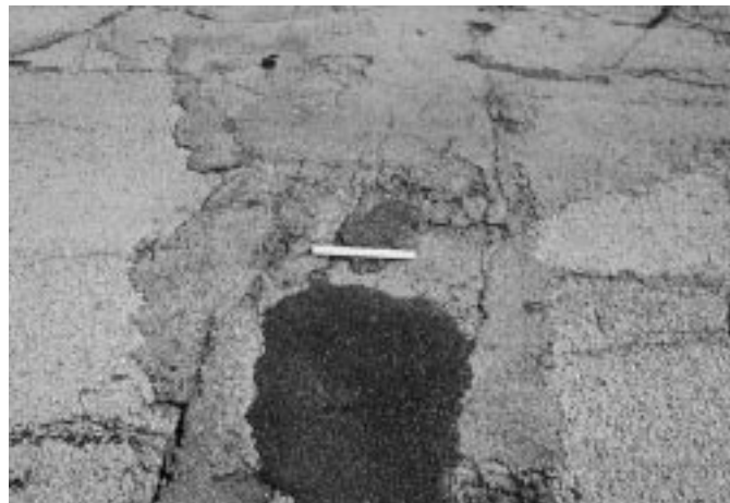
FIG. X1.33 High-Severity Patching and Utility Cut Patching
