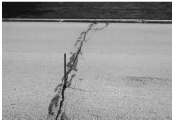
FIG. X1.29 Medium-Severity Longitudinal and Transverse Cracking
