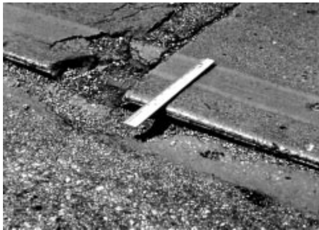
FIG. X2.19 Low-Severity Lane/Shoulder Drop-Off
