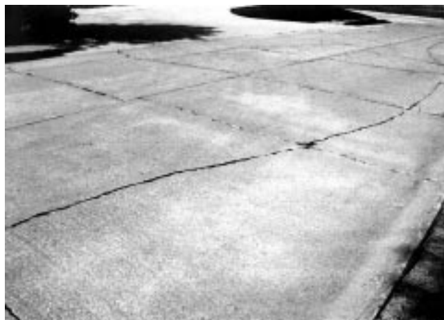
FIG. X2.7 Low-Severity Divided Slab
