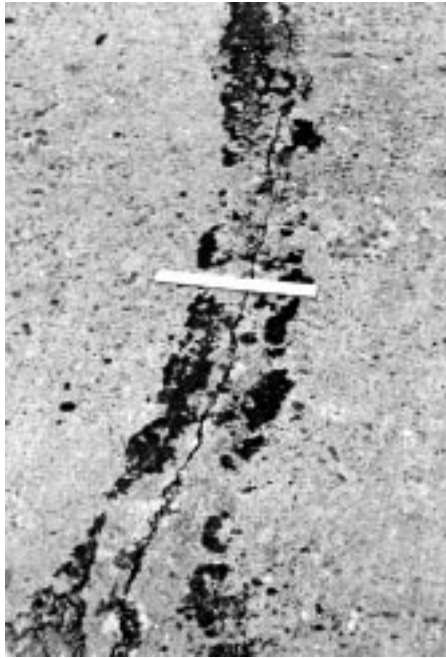
FIG. X2.22 Low-Severity Linear Cracking
