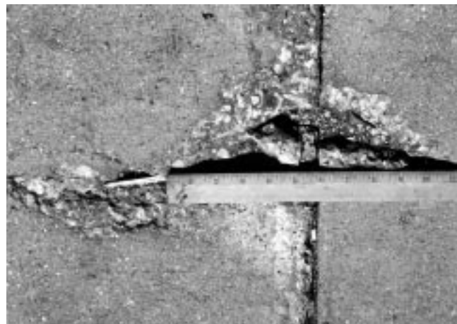
FIG. X2.46 Medium-Severity Spalling, Corner
