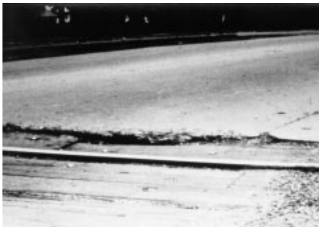
FIG. X2.40 High-Severity Railroad Crossing
