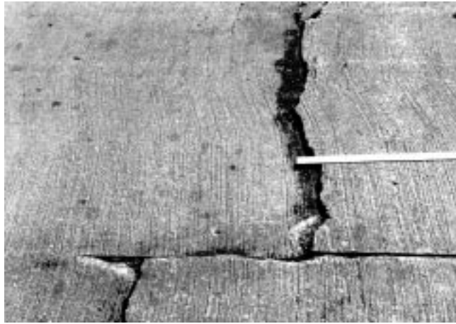
FIG. X2.24 High-Severity Linear Cracking
