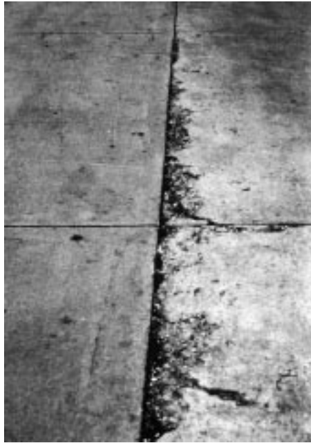
FIG. X2.49 Medium-Severity Spalling, Joint
