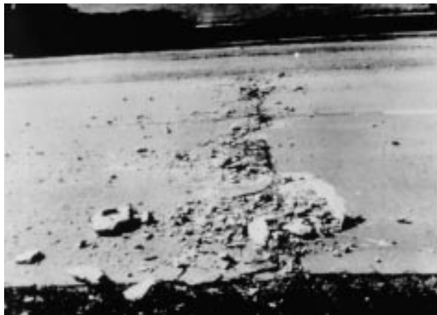
FIG. X2.2 Medium Severity Blowup/Buckling
