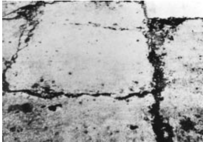
FIG. X2.27 High-Severity Patching, Large and Utility Cuts
