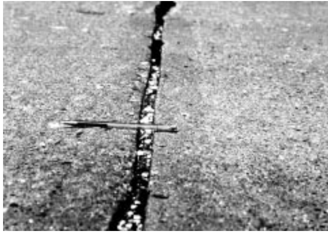
FIG. X2.18 High-Severity Joint Seal Damage
