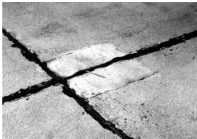
FIG. X2.28 Low-Severity Patching, Small
