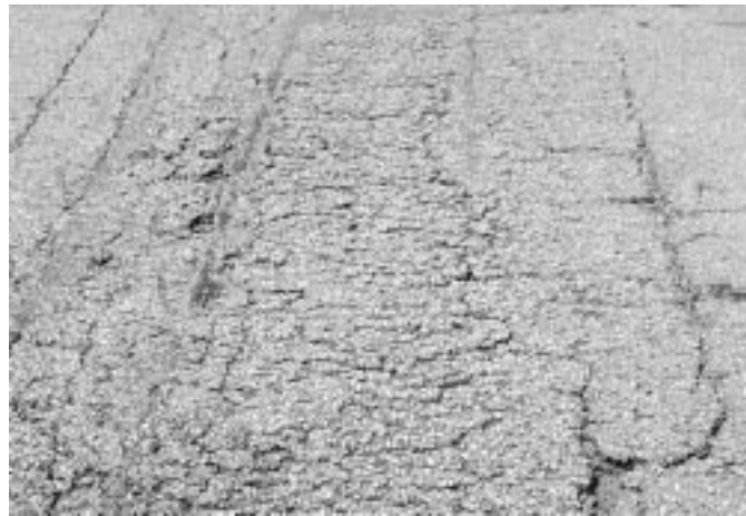
FIG. X1.52 Medium-Severity Weathering and Raveling
