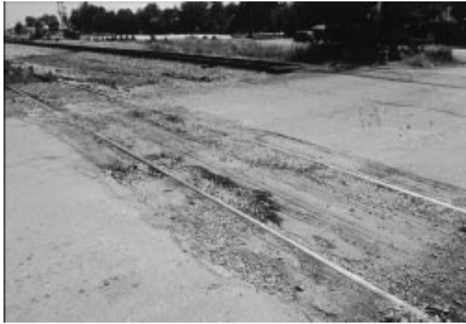
FIG. X1.40 High-Severity Railroad Crossing
