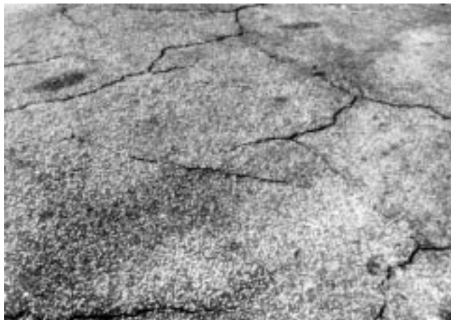
FIG. X1.9 High-Severity Block Cracking
