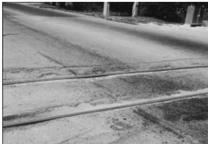
FIG. X1.39 Medium-Severity Railroad Crossing
