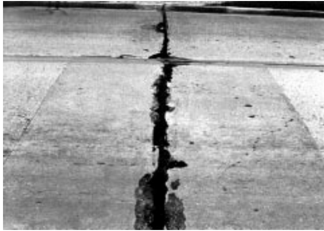
FIG. X2.16 Low-Severity Joint Seal Damage
