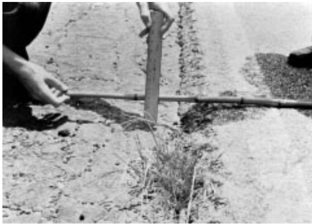
FIG. X1.26 Medium-Severity Lane/Shoulder Drop-Off
