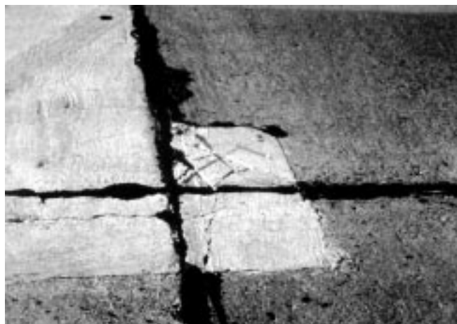
FIG. X2.29 Medium-Severity Patching, Small
