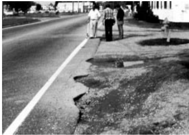
FIG. X1.21 High-Severity Edge Cracking
