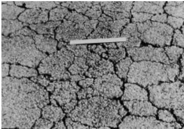
FIG. X1.3 High-Severity Alligator Cracking
