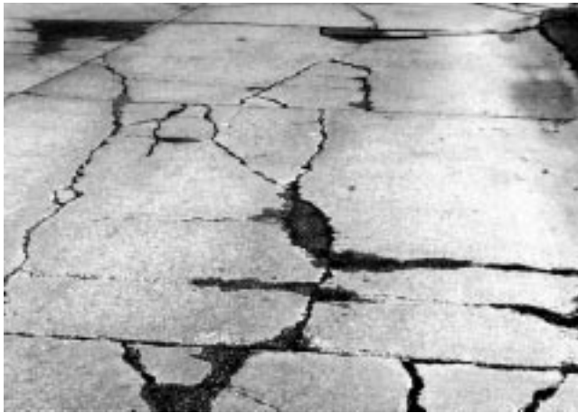
FIG. X2.9 High-Severity Divided Slab
