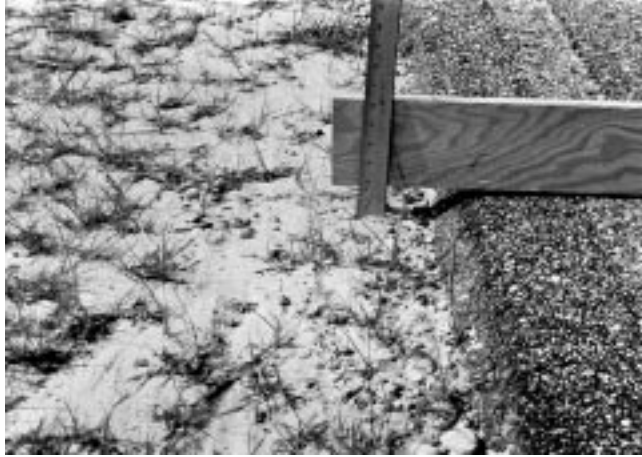
FIG. X1.25 Low-Severity Lane/Shoulder Drop-Off
