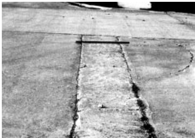
FIG. X2.26 Medium-Severity Patching, Large and Utility Cuts
