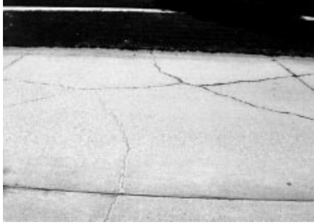
FIG. X2.8 Medium-Severity Divided Slab
