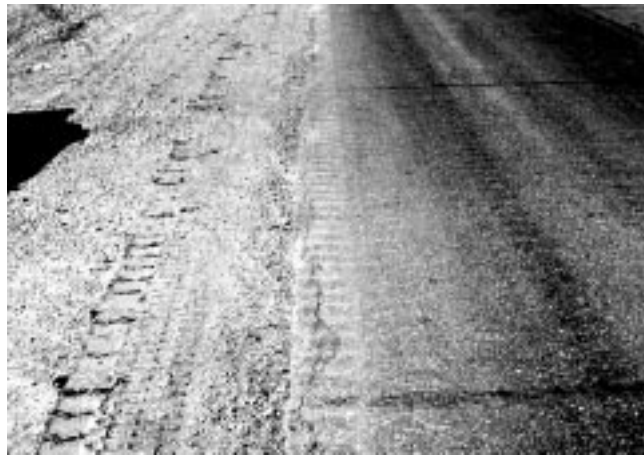
FIG. X1.22 Low-Severity Joint Reflection Cracking
