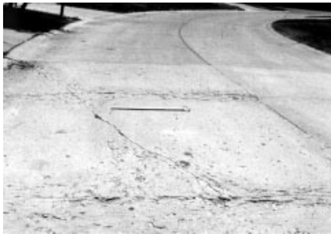
FIG. X2.12 High-Severity Durability Cracking
