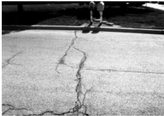
FIG. X1.8 Medium-Severity Block Cracking
