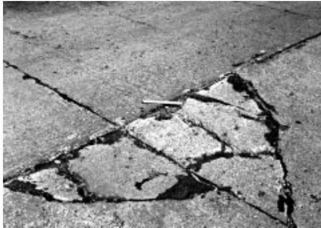
FIG. X2.6 High-Severity Corner Break
