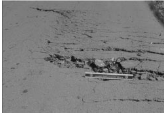
FIG. X1.49 High-Severity Slippage Cracking
