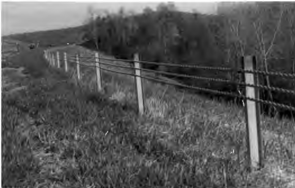
Figure 5-5. Three-Strand Cable Barrier
