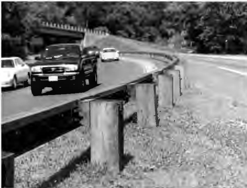
Figure 5-18. Backed Timber Guardrail
