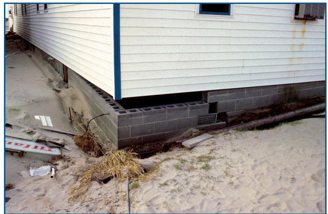
Failure of crawlspace foundation undermined by scour.
