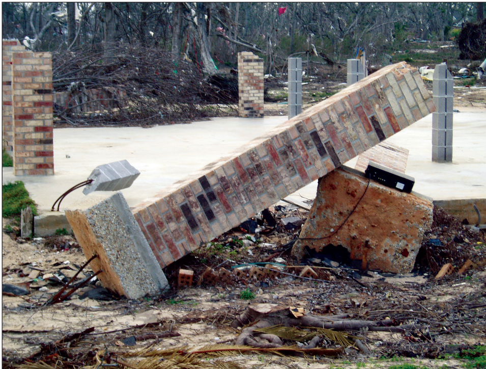
Figure 2-7. Performance comparison of pier foundations. Piers on discrete footings (foreground) failed by rotating and overturning while piers on more substantial footings (in this case a concrete mat) survived (Pass Christian, Mississippi).
