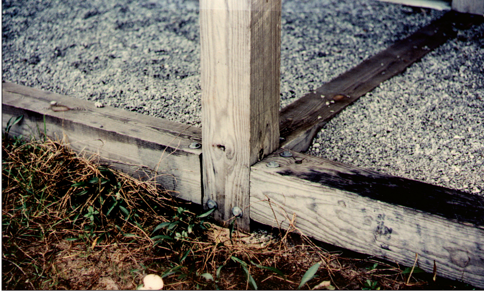
Figure 2-3. Compression strut at base of a wood piling. Struts provide some lateral support for the piling, but very little resistance to rotation.
