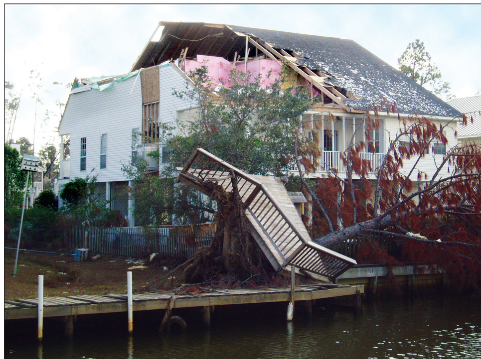
Figure 1-1. Wind damage to roof structure and gable end wall from Hurricane Katrina (2005) (Pass Christian, Mississippi)
