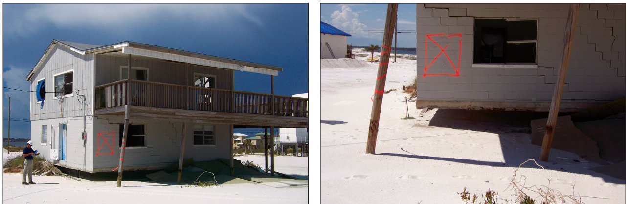
Figure 2-2. Slab-on-grade foundation failure due to erosion and scour undermining and closeup of the foundation failure from Hurricane Dennis, 2005 (Navarre Beach, Florida)
