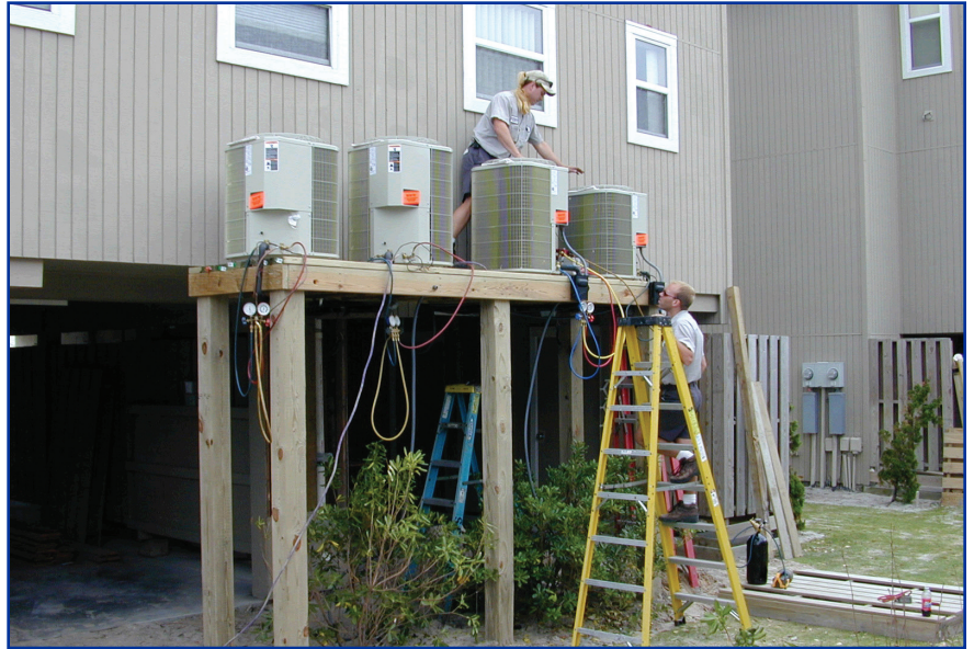
Elevated air conditioning compressors.
