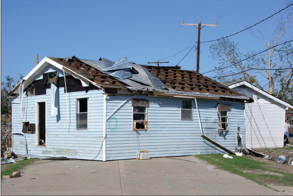
Figure 1-7. Building floated off of foundation (Plaquemines Parish, Louisiana)
