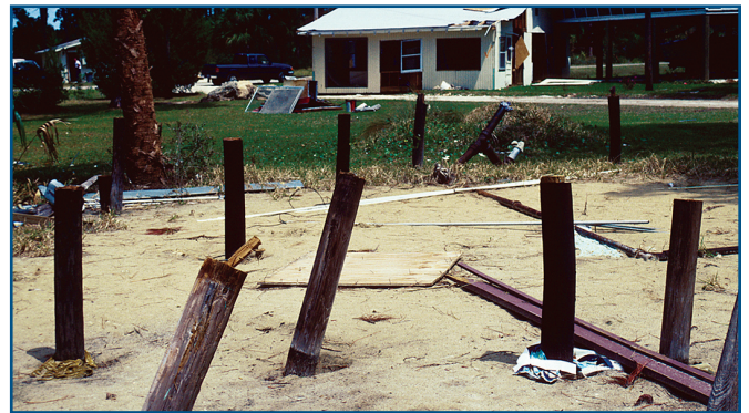
Insufficient pile embedment and failure of connections at tops of piles allowed elevated building to be floated off its foundation.
