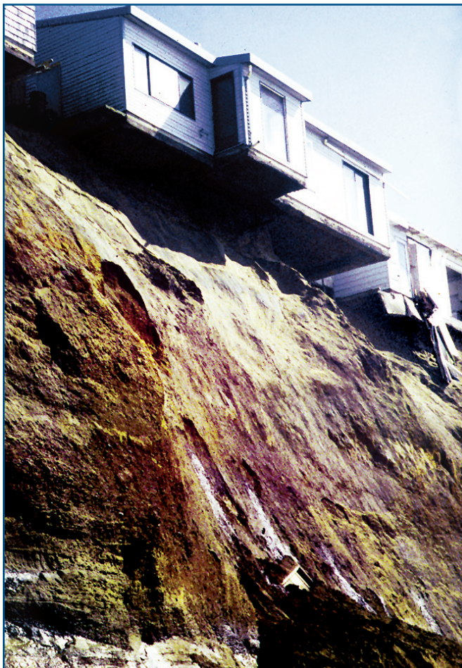
House undermined by bluff erosion. Photograph by Lesley Ewing. Courtesy of California Coastal Commission.
