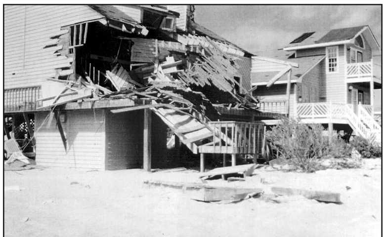
Figure 2. Well-sited building that still sustained damage.
