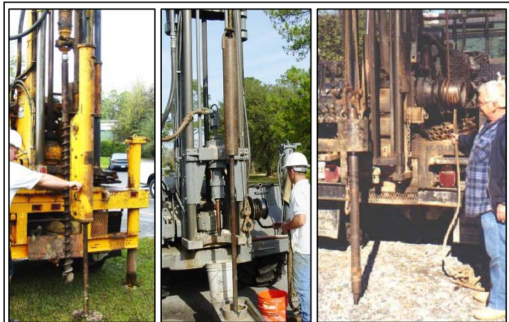
Figure 2: a) Automatic Hammer ~95% eff., b) Safety Hammer ~60% eff., c) Donut Hammer ~45% eff. (photo from GeoServices Corp.)
