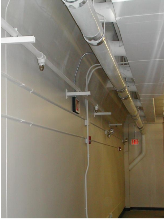
Photo 6 – Return air ductwork at top of wall system. Discrete duct “taps” connect top of wall return plenum to main return air ductwork.
