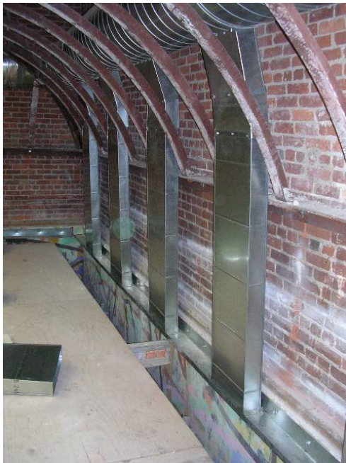
Photo 8 – Return air ductwork concealed in attic above curved ceiling.
