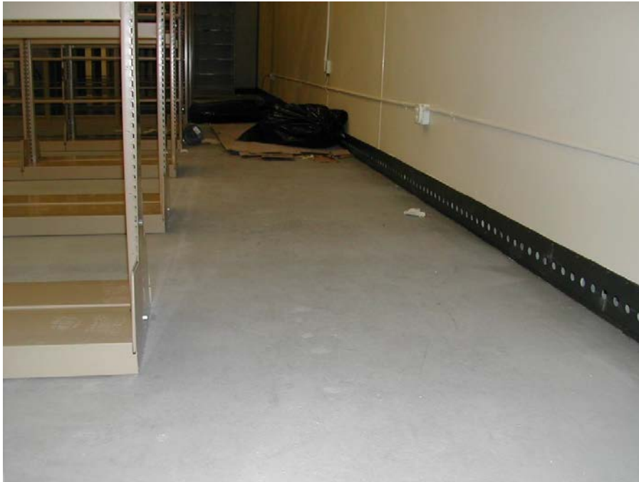
Photo 5 – Calibrated restrictor plate exposed at base of vented wall.
