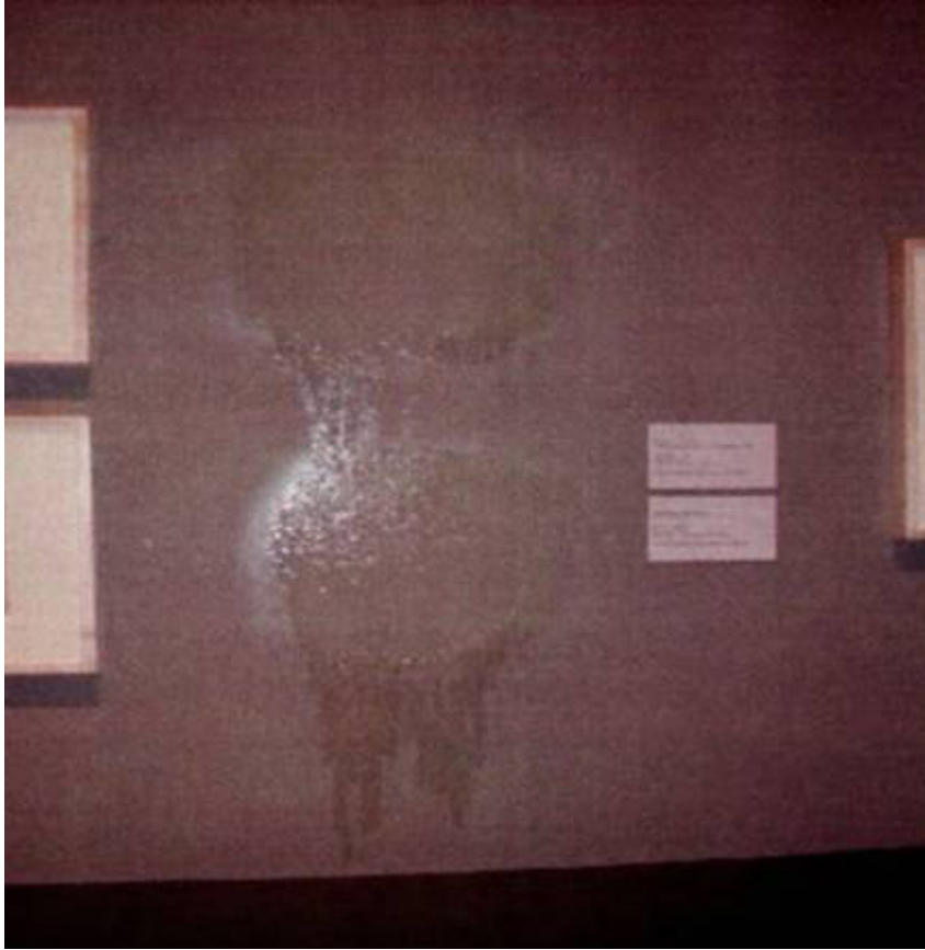
Photo 4 – Moisture accumulation on an exterior wall (plaster installed over 3-wythe brick masonry) behind hung artwork. Artwork has been removed in this photograph.
