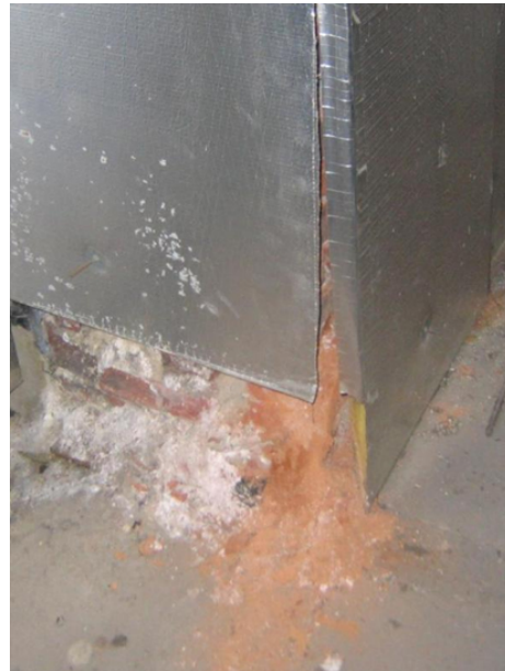
Photo 3 – insulation combined with a vapor retarder led to accelerated freeze-thaw damage to interior wythe of masonry in a solid brick wall.
