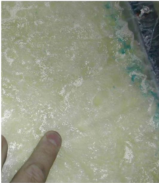
Photo 2 – Moisture trapped on the outboard face of an interior vapor retarder installed over a solid masonry wall.
