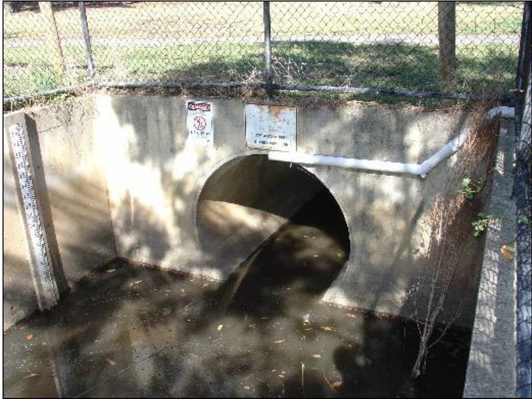
Figure 3-19 Pipe outlet at Doncaster (sampling point is 15 m upstream)
