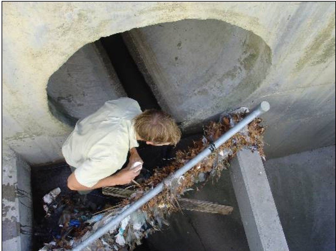
Figure 3-13 Pipe outlet at Richmond. The sampling point is 250m upstream of the pipe outlet
