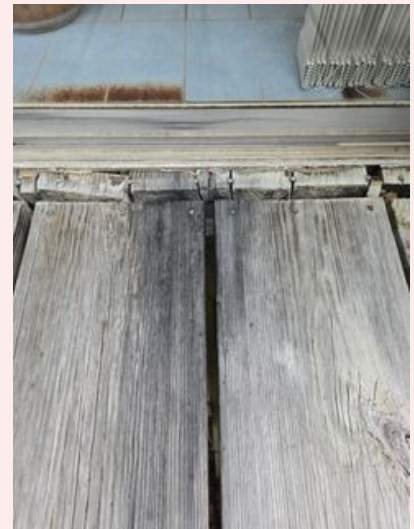
Additional decay noted under the flower pots and hummingbird Peter were additional moisture is added to the horizontal surfaces
