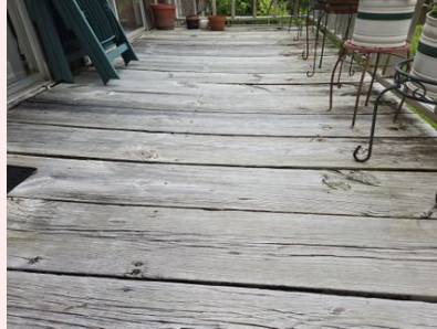
Uneven cupping and where on the various boards
