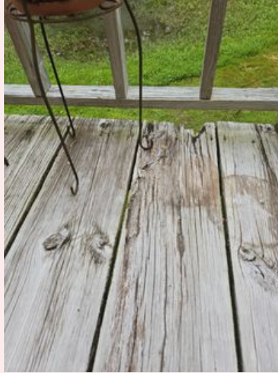
Wood rot and excessive material loss at end of board near joist
