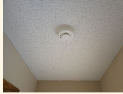
It's supposed to be a smoke alarm not a CO2 and is located between bedrooms two and three
