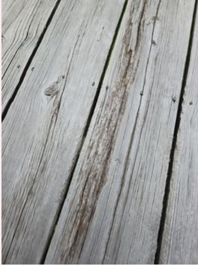
Excessive where and we getting a board due to missing material
