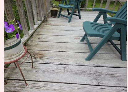
Excessively weather worn and cracks beginning to show in the middle of the boards
