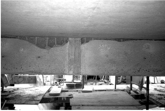
Effects of not filling the cavity.
