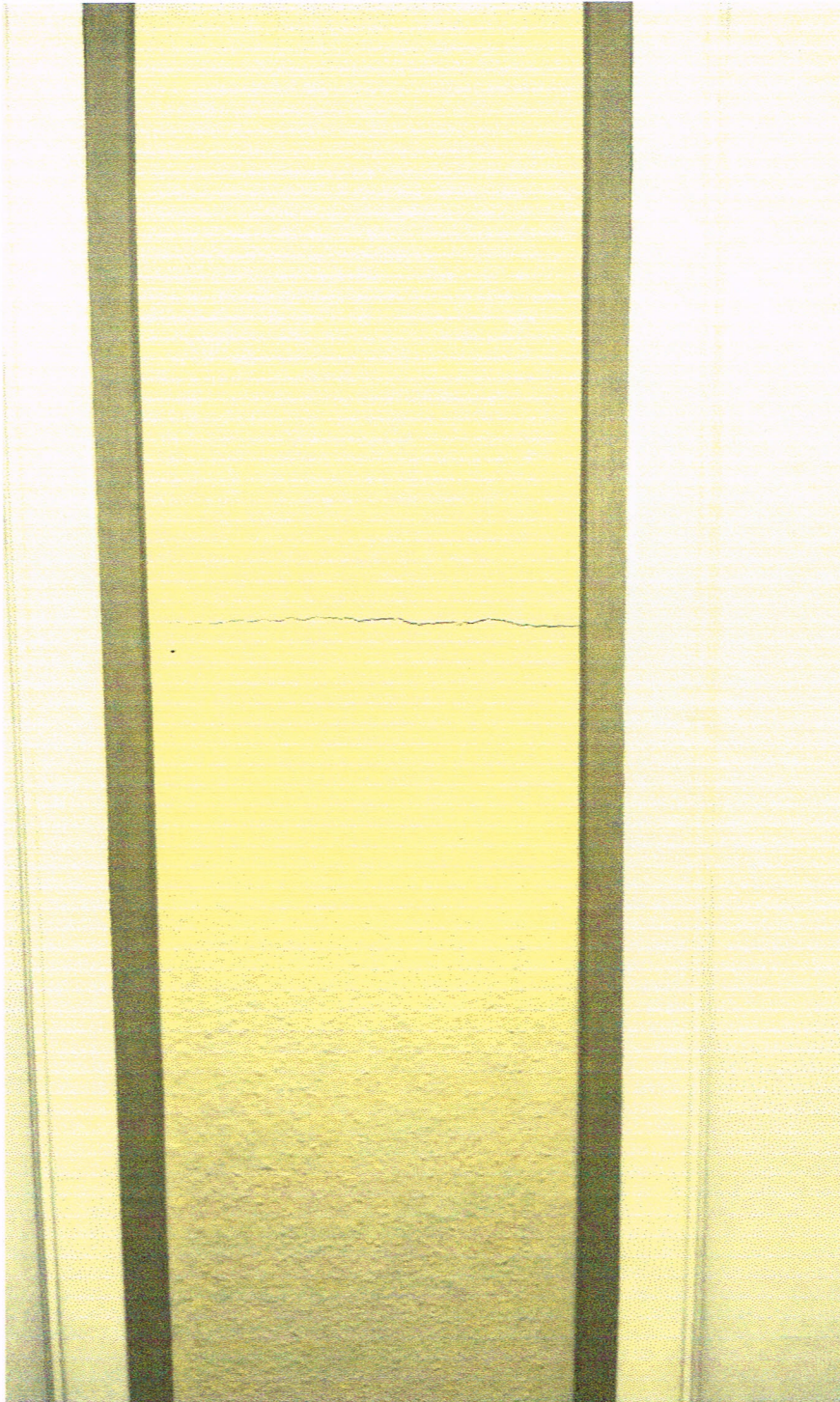
Photograph 1: Hallway gypsum wallboard cracking near rooms 203 and 205.
