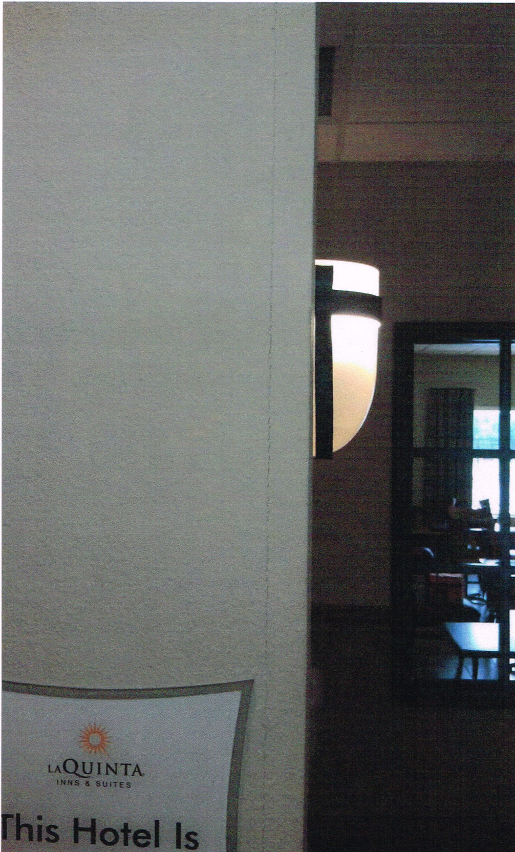
Photograph 7: Another view of the gypsum wallboard cracking near the front desk.
