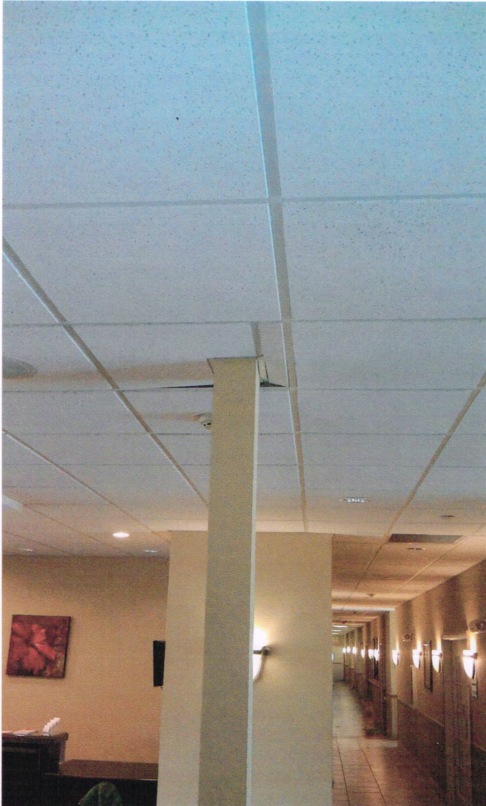
Photograph 5: Column in the atrium placed approximately below Room 203/ 201 to support the beam that provides support to the floor trusses in the hallway and the walls above it to provide the clear opening in the atrium below. The ceiling tile is reflecting movement of the structural framing surrounding the column.
