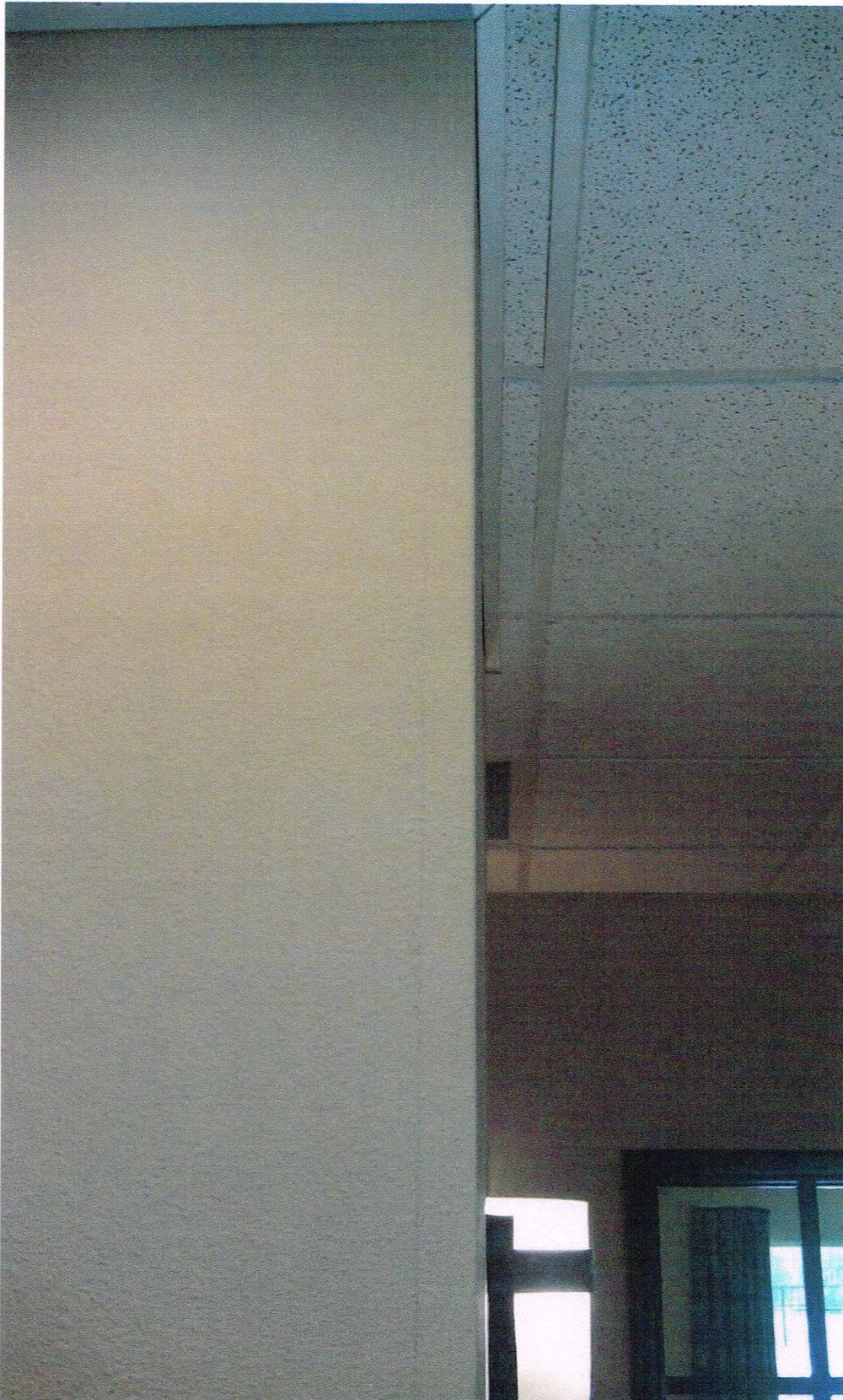
Photograph 8: A view of the gypsum wallboard cracking near the front desk and a view toward the ceiling tile.
