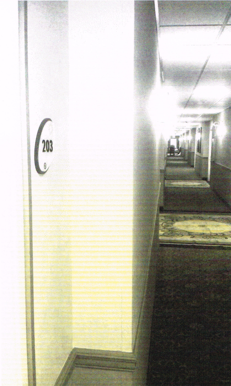
Photograph 3: Hallway gypsum wallboard cracking near room 203.
