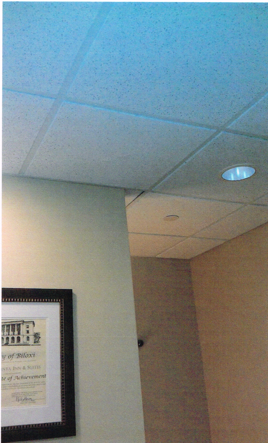
Photograph 9: Ceiling tile movement at the front entry way corner near the backside of the front desk.
