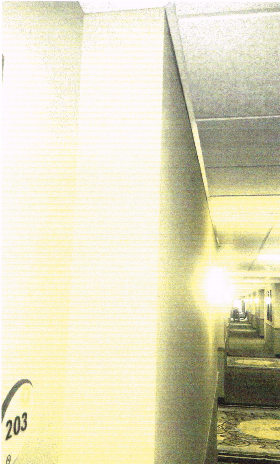
Photograph 2: Hallway gypsum wallboard cracking near room 203.
