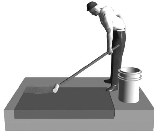
Fig. 11—Cure with wet coverings, or use a spray- or roller-applied curing compound as shown here.
