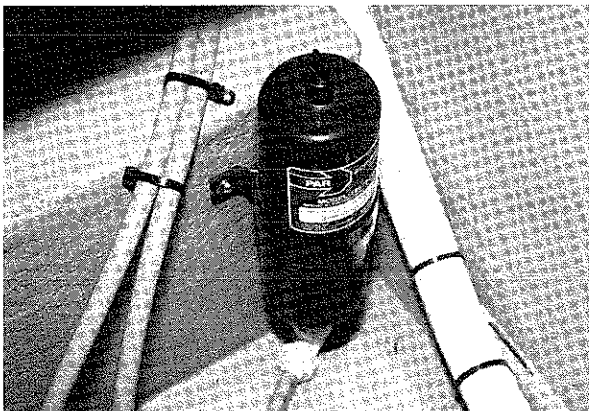
Pneumatic Accumulator Tank
