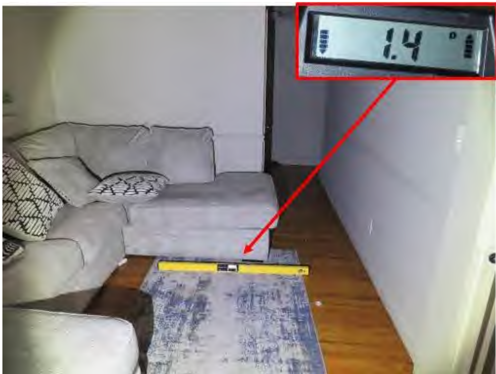
Photo No. 28: The living room's floors were not level.
