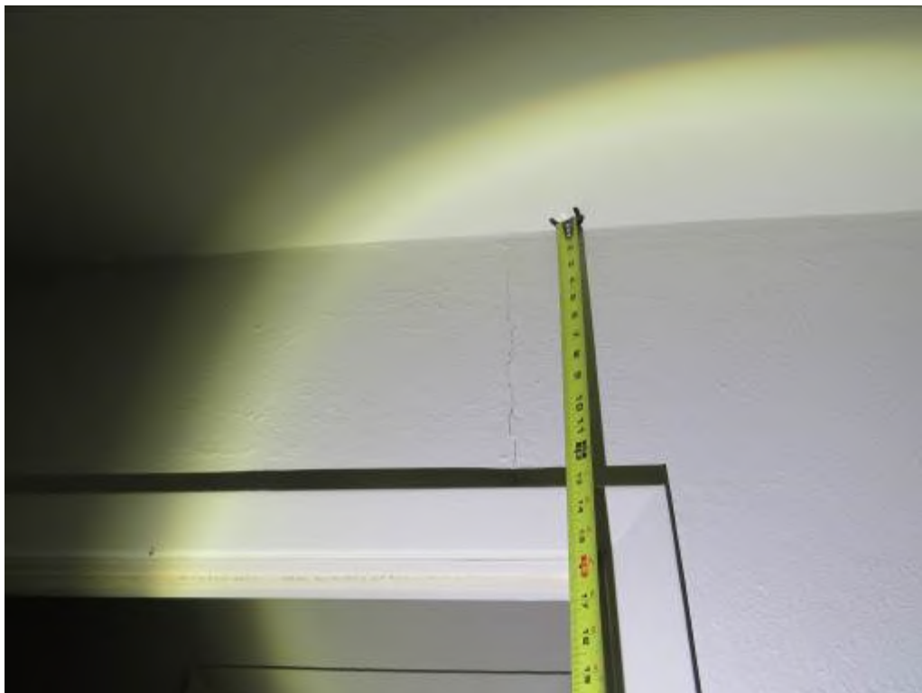
Photo No. 32: A crack was noted in the drywall above the door.
