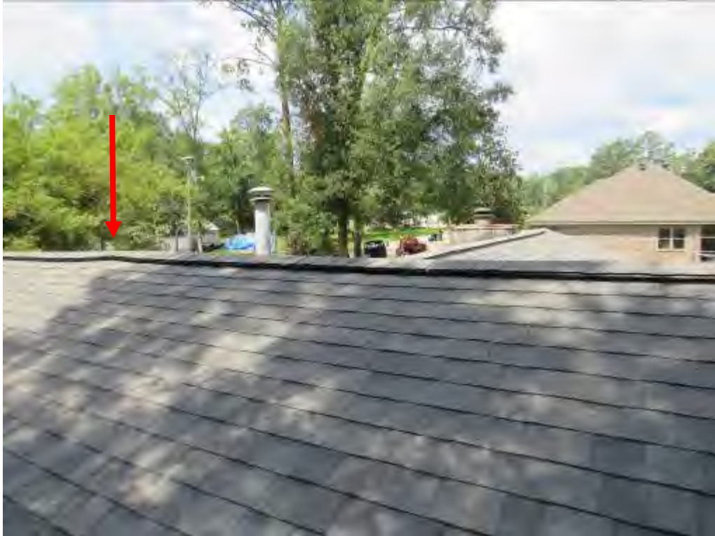
Photo No. 13: A high-point was noted near the middle of the roof.
