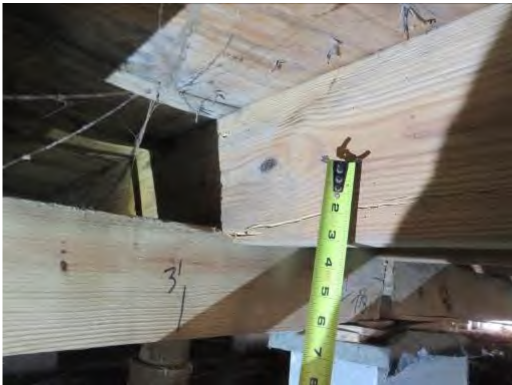
Photo No. 56: One broken floor framing member was noted adjacent to the repair location.
