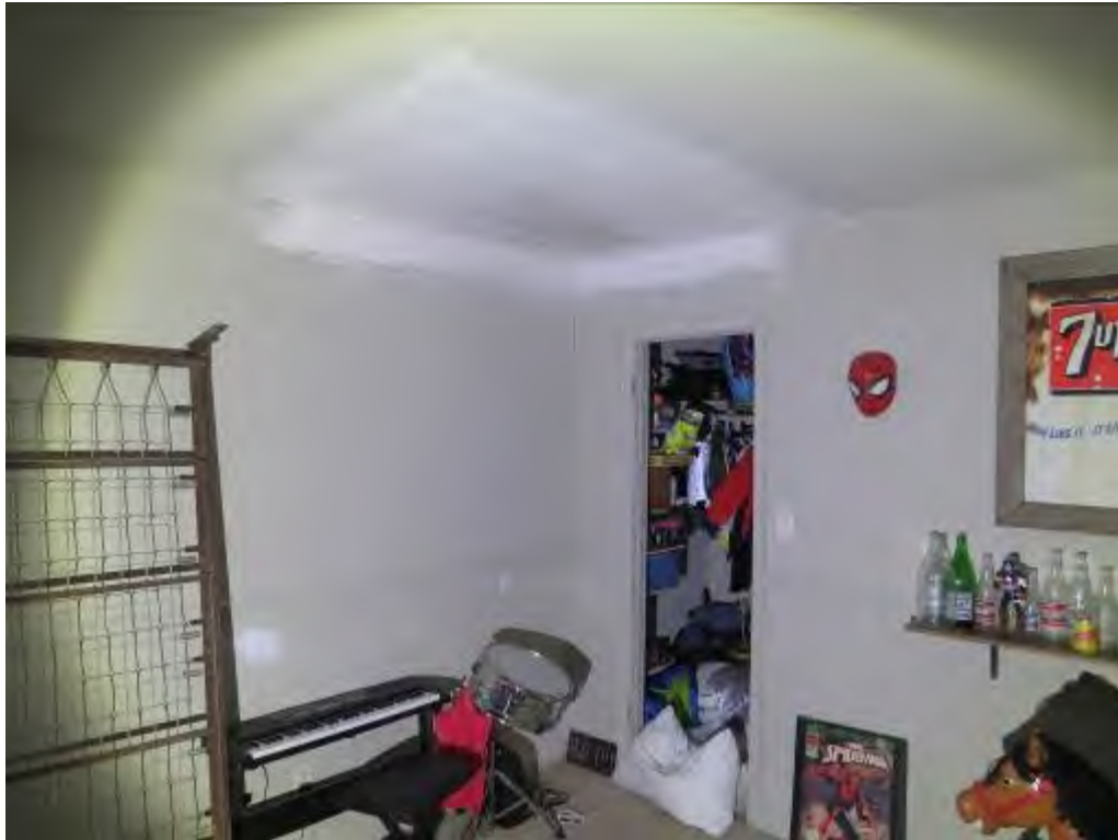
Photo No. 35: On-going repair activities were noted in the southeast bedroom's ceiling.
