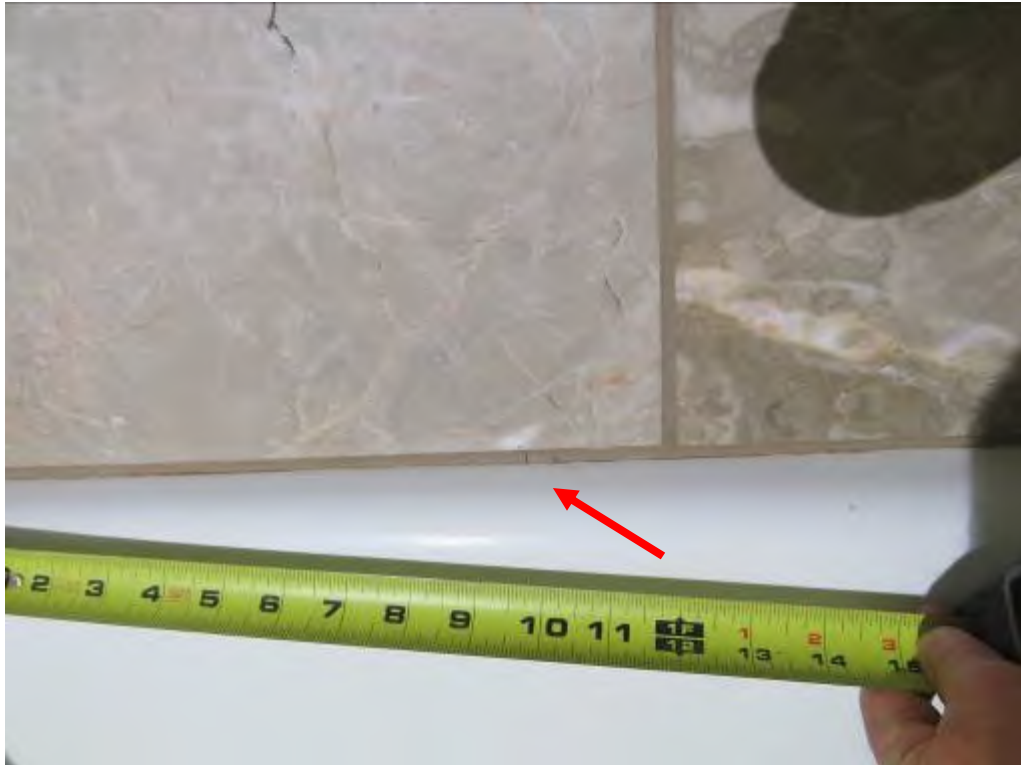
Photo No. 43: Cracks were noted in the ceramic tile's grout.
