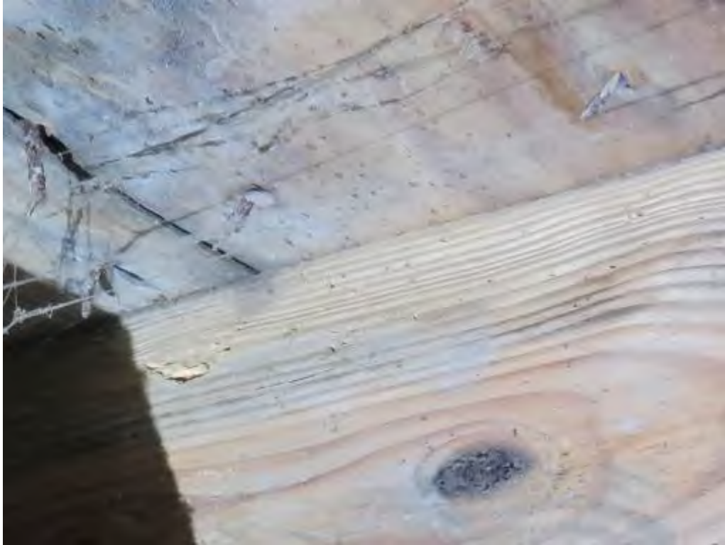
Photo No. 57: Numerous small holes were noted in the framing member.
