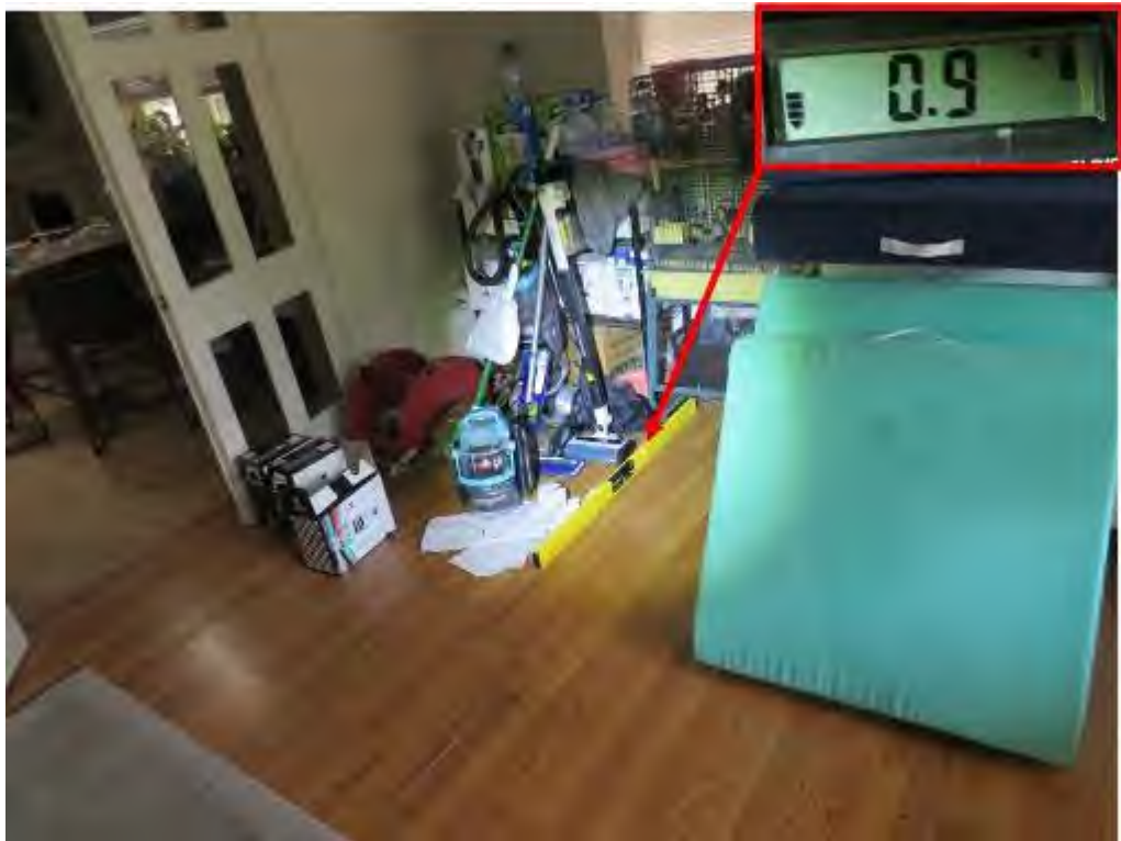
Photo No. 18: The playroom's west-side floors sloped down toward the west.
