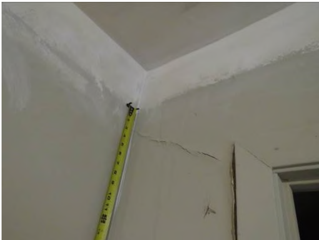
Photo No. 36: The room's east-side wall paint was cracked and delaminated.
