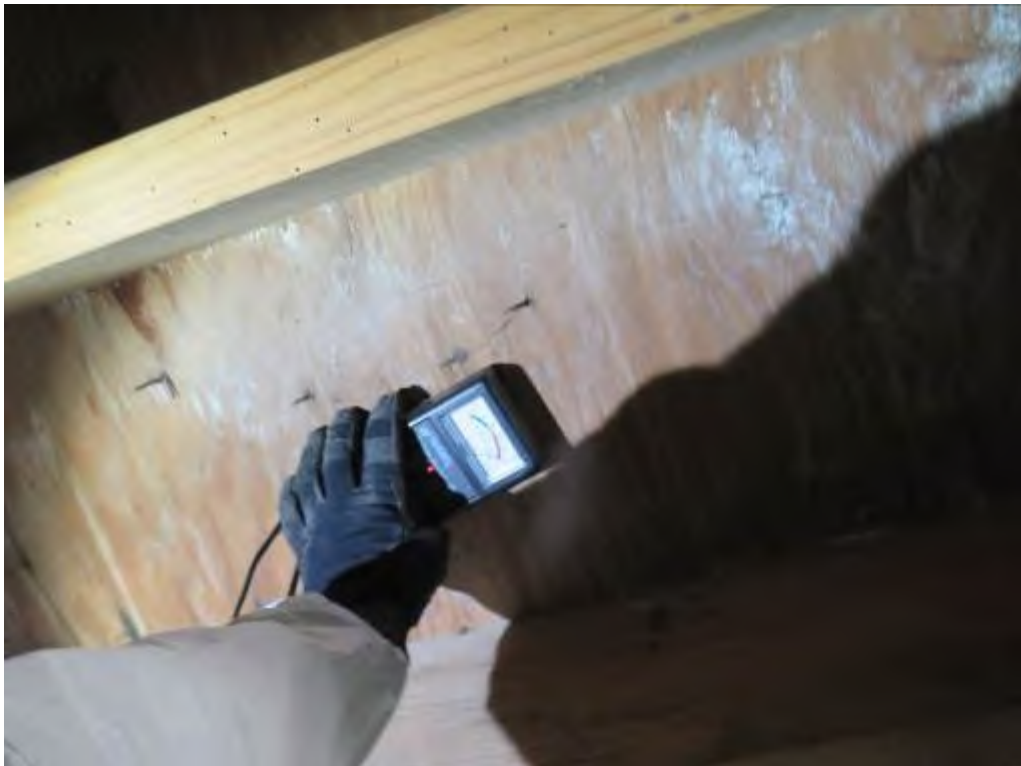
Photo No. 54: The subfloor's moisture content was elevated above 30%.
