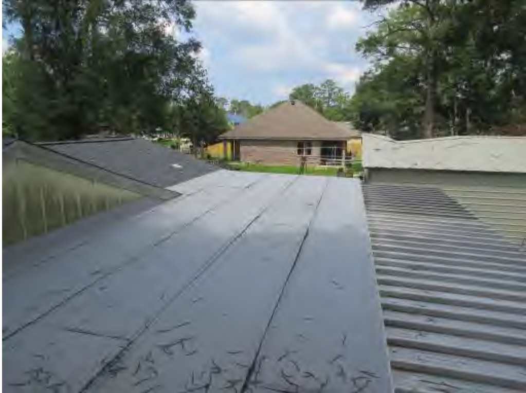
Photo No. 11: A modified-bitumen membrane covered the rear portion of the residence.
