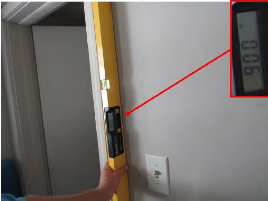
Photo No. 19: The playroom's walls were plumb or near plumb.
