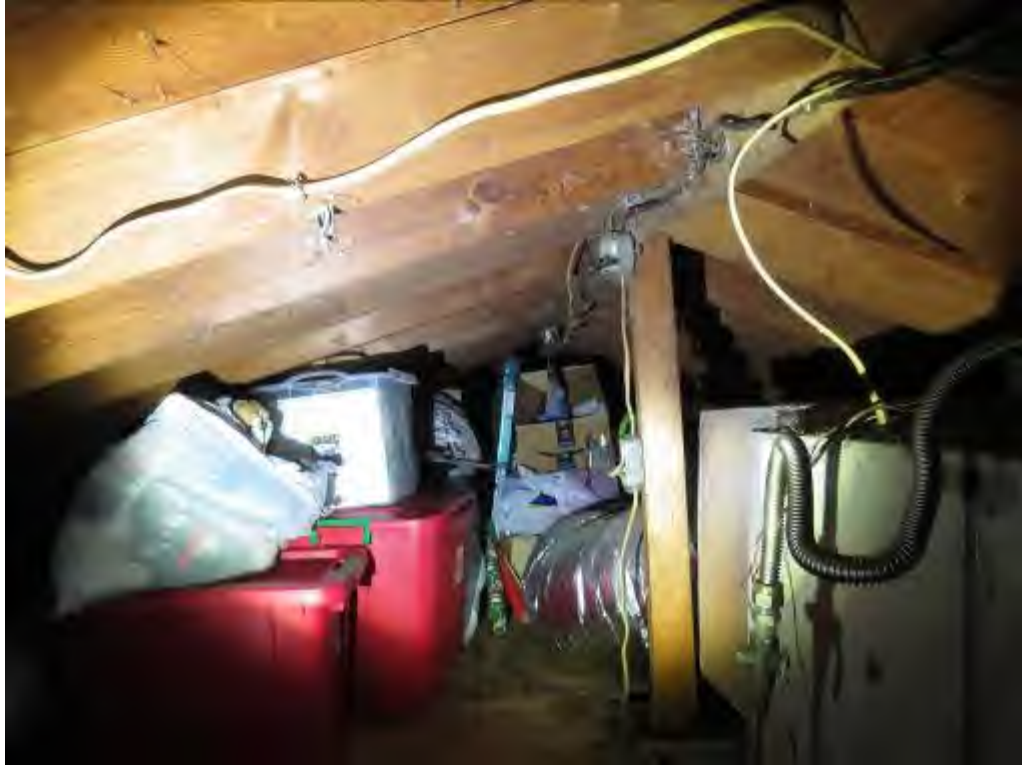
Photo No. 51: The north-south ridge beam was supported by one (1) king post.
