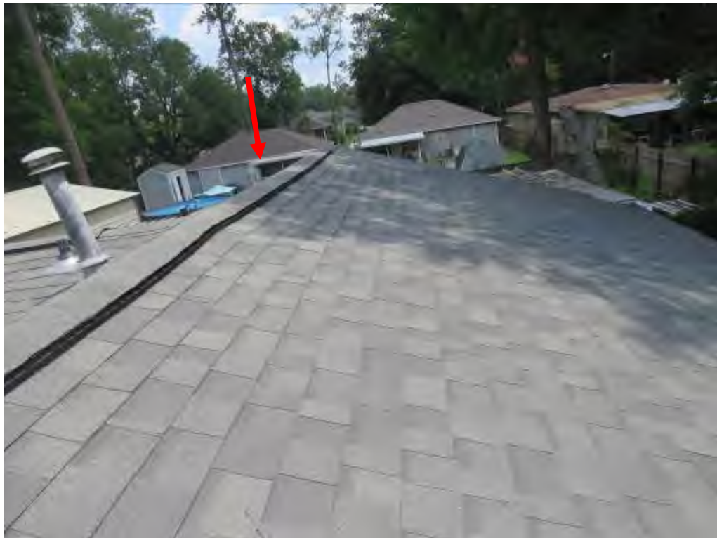
Photo No. 12: The roof ridgeline spanning in the north-south direction was sagging.
