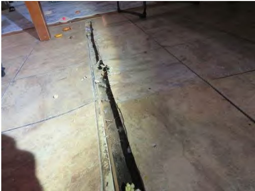
Photo No. 22: Dirt and debris were noted within the missing area
