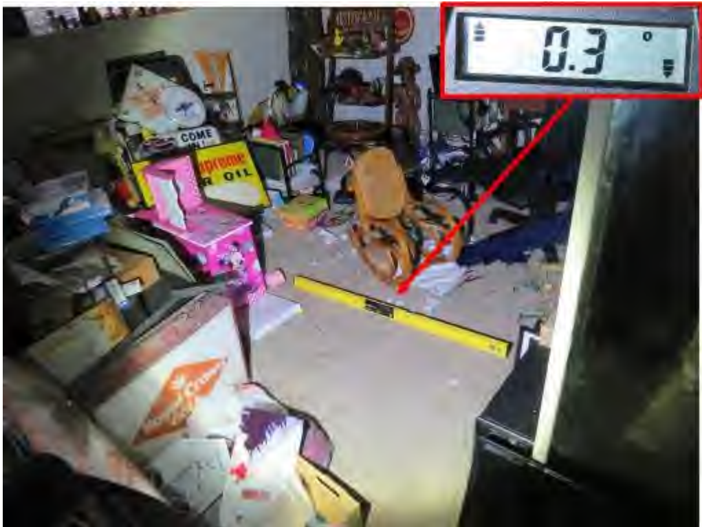
Photo No. 34: The bedroom's floors were near level.
