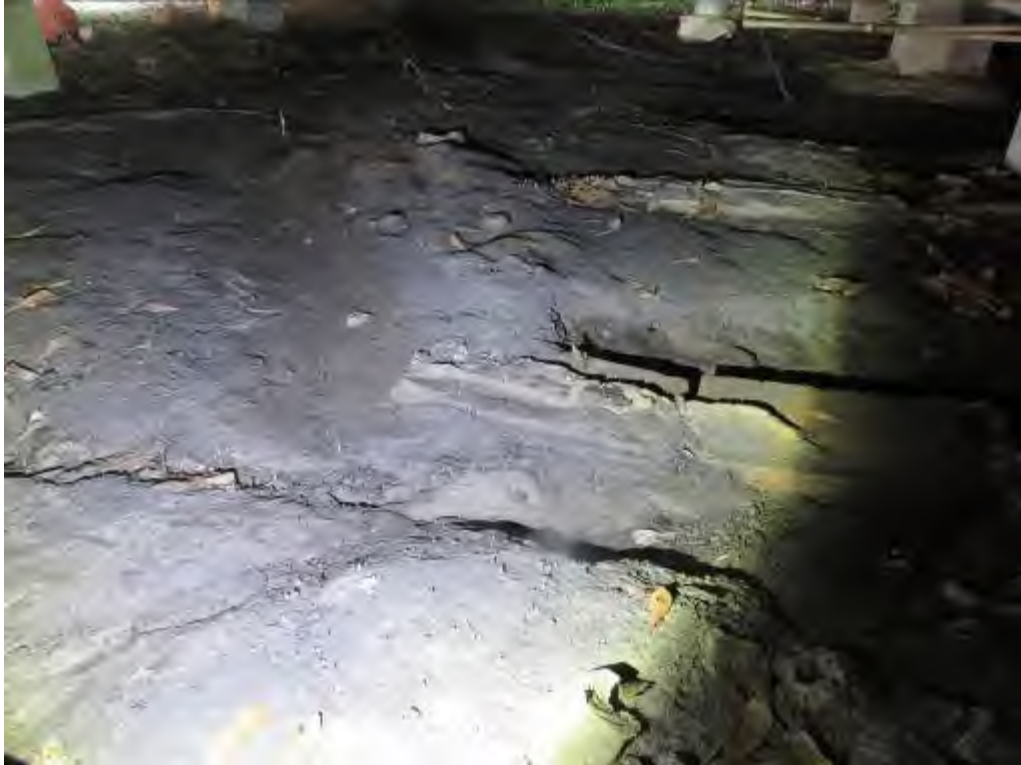
Photo No. 53: Several trenches were noted in the crawlspace floor.
