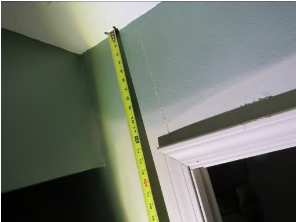
Photo No. 50: The cracks were vertical on the walls.
