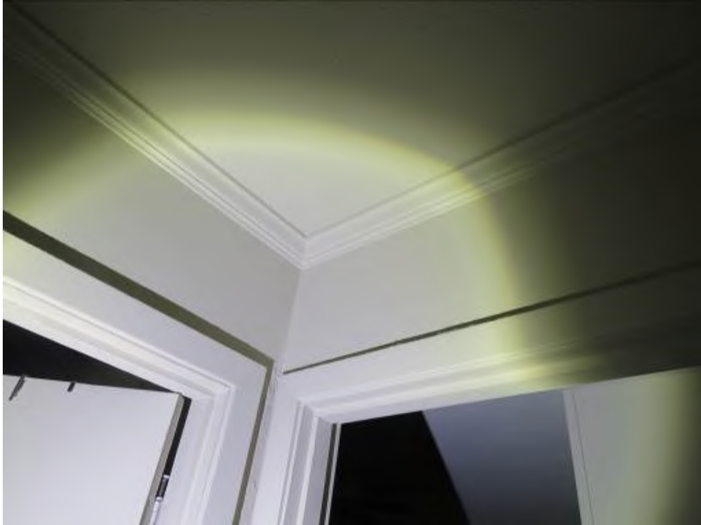
Photo No. 33: No cracks were noted in the adjacent hallway's drywall.
