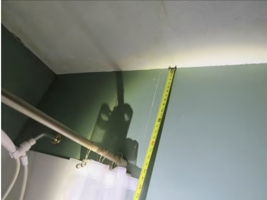
Photo No. 49: The wall drywall was cracked.
