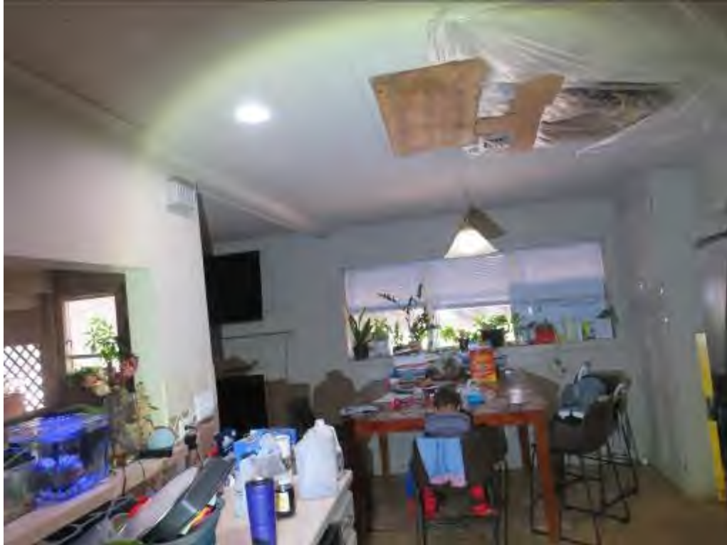
Photo No. 21: A section of the kitchen's ceiling drywall was missing.
