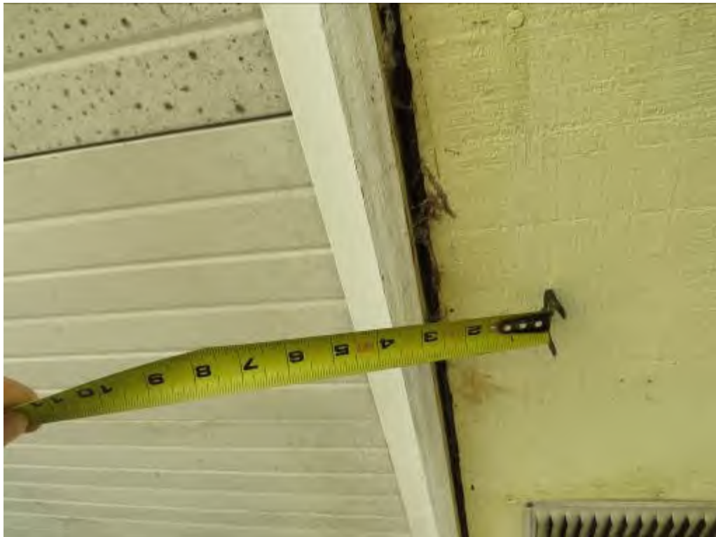
Photo No. 10: A gap was visible between the rear soffit and fascia board.
