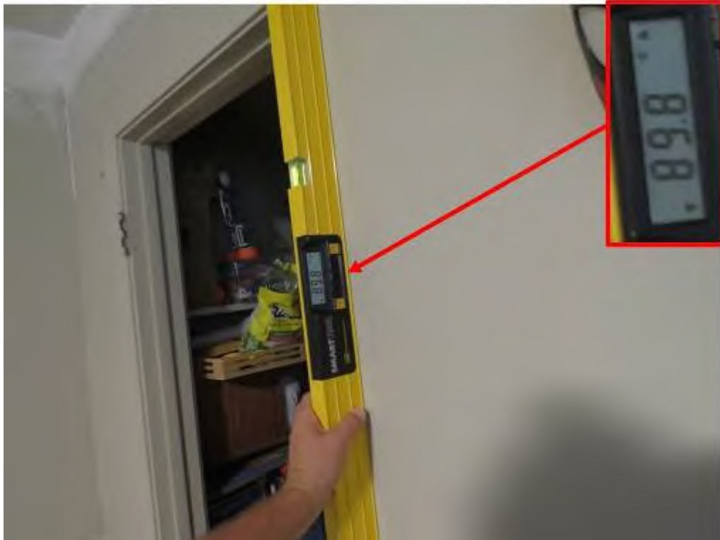
Photo No. 39: The room's walls were plumb or near plumb.
