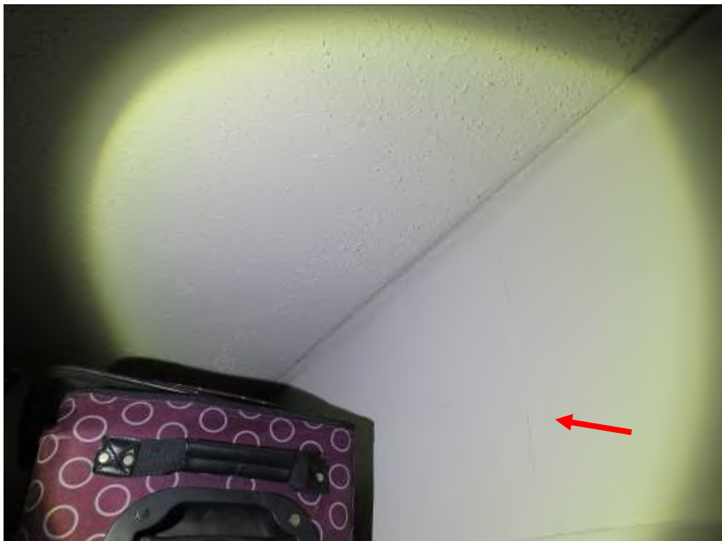
Photo No. 44: A crack was noted in the closet's drywall, above the door.
