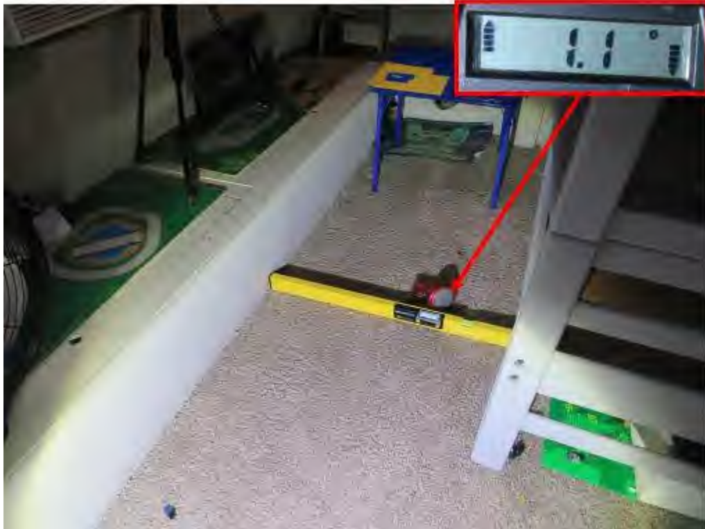
Photo No. 41: The bedroom's floors were not level.
