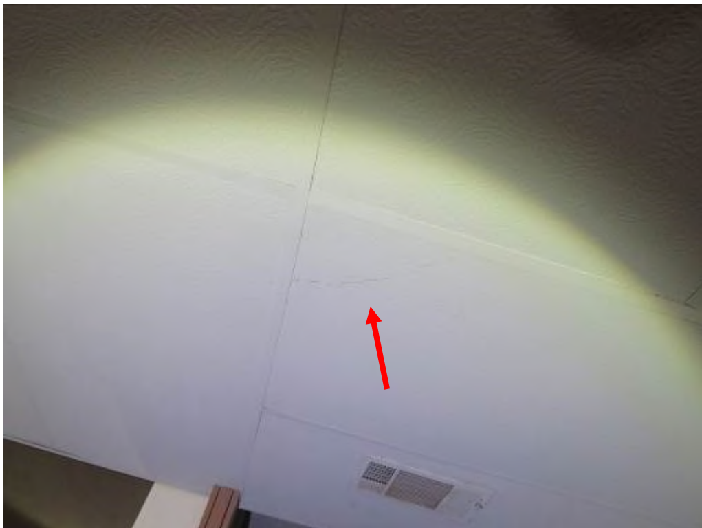
Photo No. 46: One of the tiles was broken.
