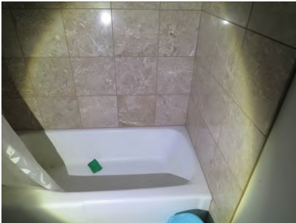
Photo No. 42: The bathtub surround was comprised of ceramic tiles.
