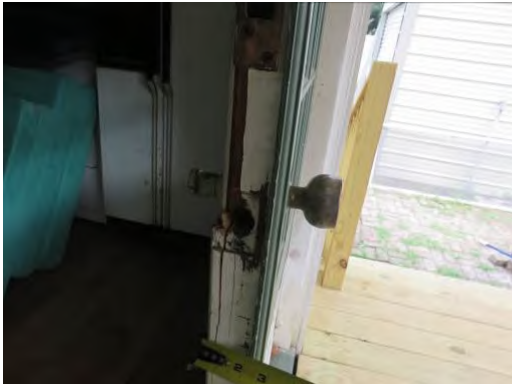
Photo No. 16: The rear door was broken.
