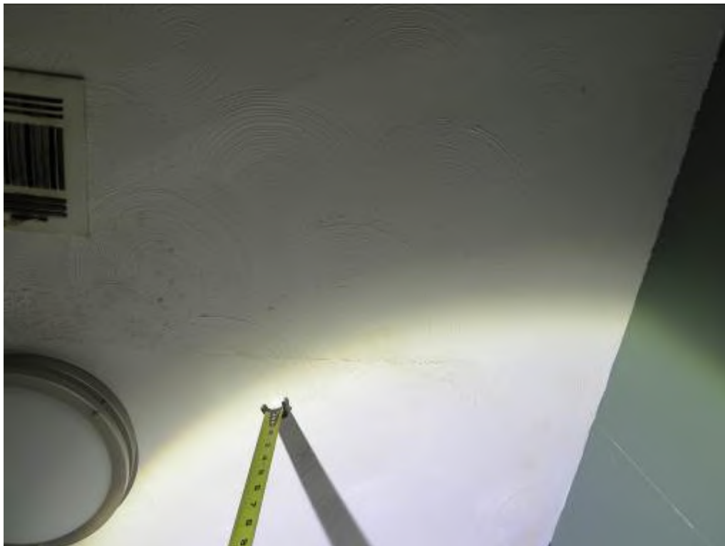
Photo No. 48: The ceiling drywall was cracked.
