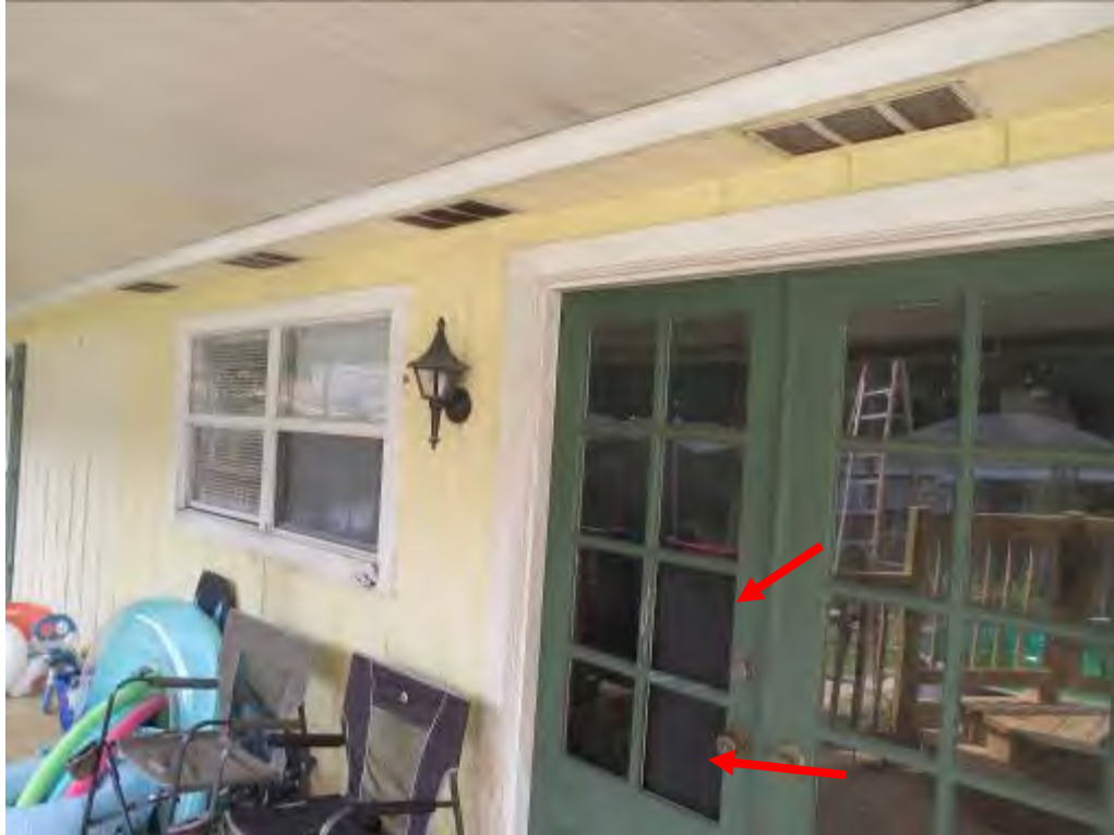
Photo No. 15: Two of the rear door's window panes were missing.
