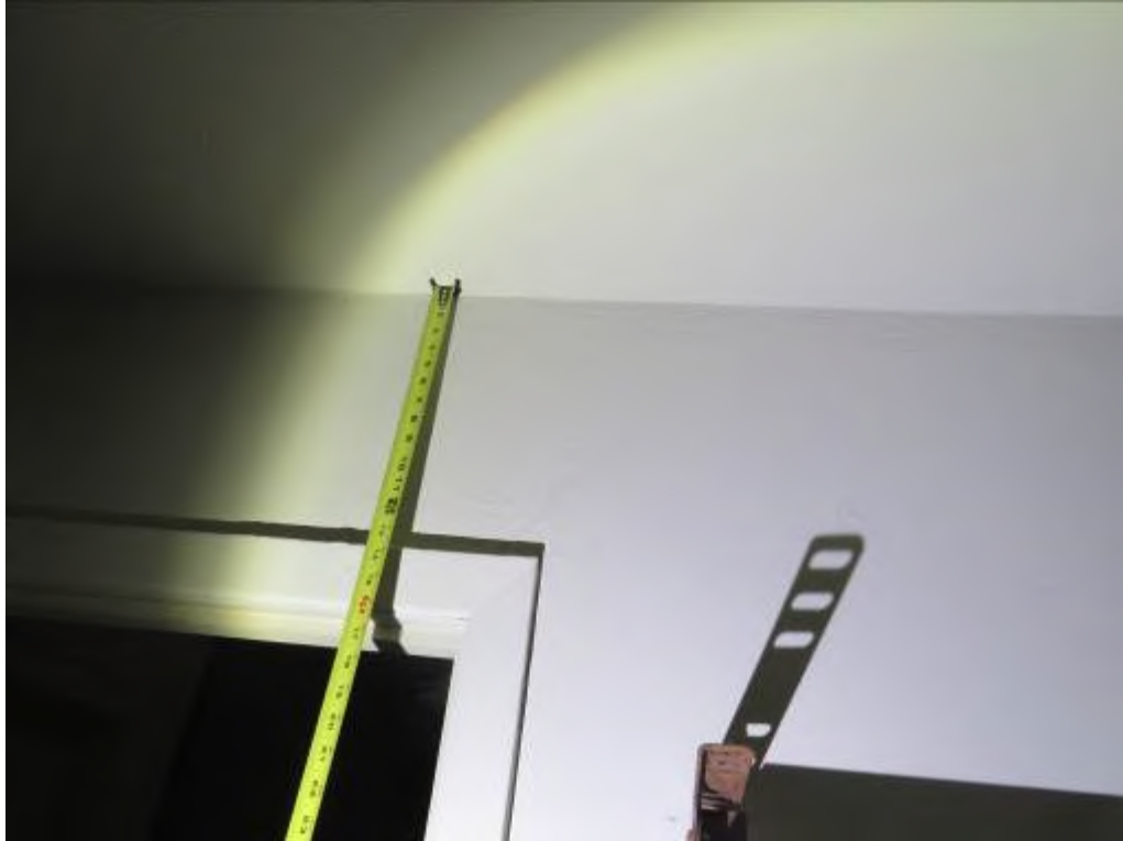
Photo No. 37: A crack was noted above the door to the bedroom.
