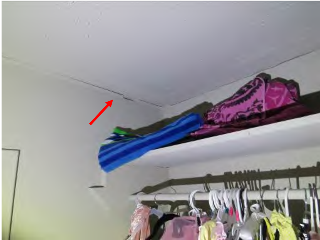
Photo No. 45: The drywall tape at the ceiling wall interface, above the door was delaminated.
