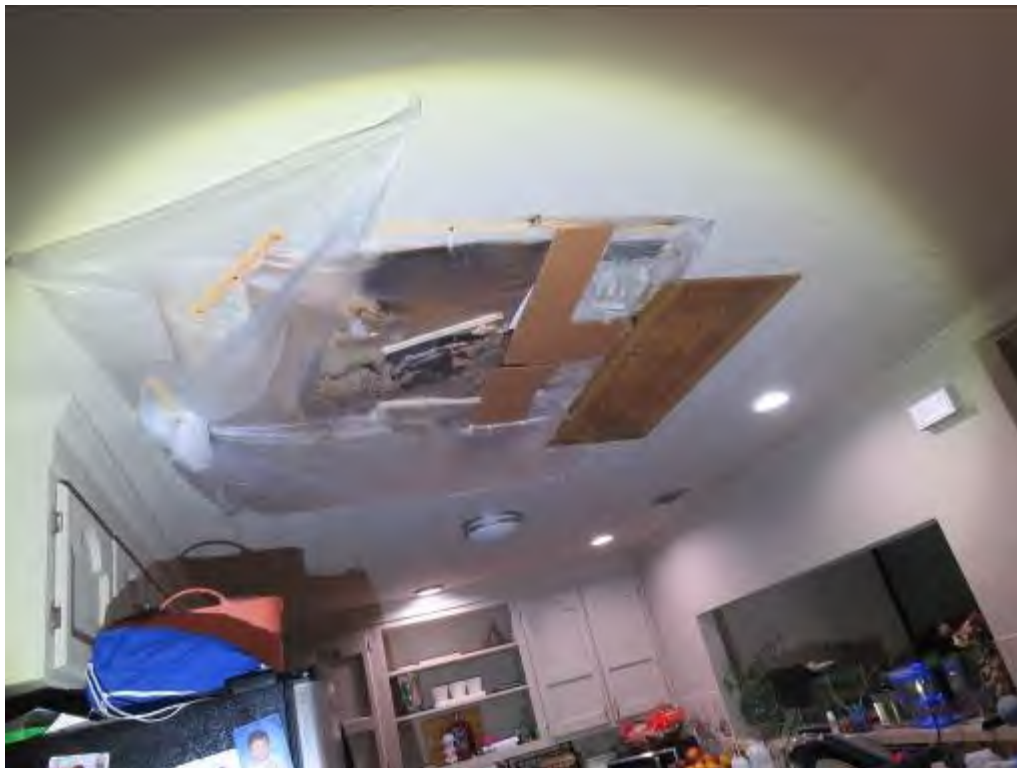
Photo No. 26: No cracks were noted in the remainder of the kitchen's ceiling or walls.
