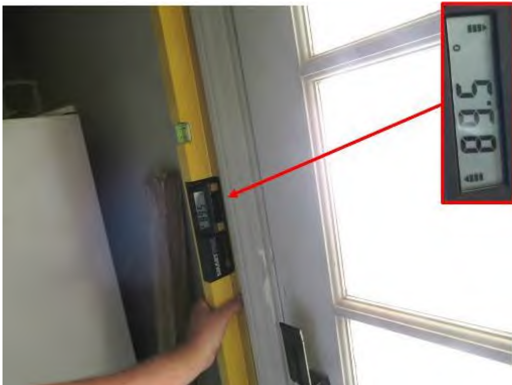
Photo No. 20: The playroom's walls were plumb or near plumb.
