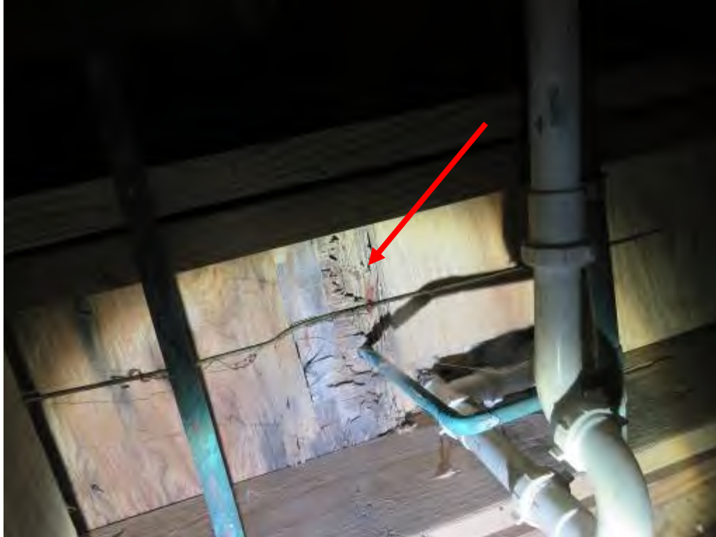
Photo No. 55: Deteriorated subfloor was noted under the bathrooms area.
