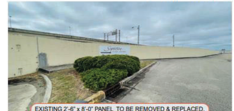
EXISTING 2'-6" x 8'-0" PANEL TO BE REMOVED & REPLACED. WILL REQUIRE NEW 4' x 4' PRESSURE TREATED POSTS.
