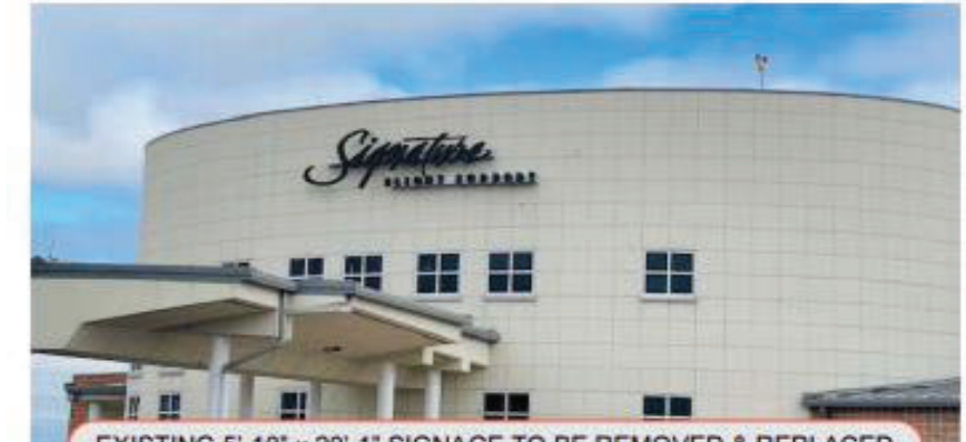
EXISTING 5'-10" x 20'-1" SIGNAGE TO BE REMOVED & REPLACED WALL TO BE REPAIRED AS REQUIRED
