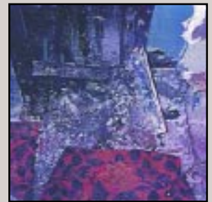
Burned gypsum shaft
